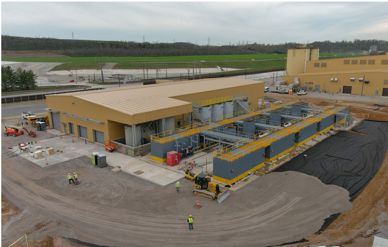
Ghent – ELG Water Treatment – April 2023
