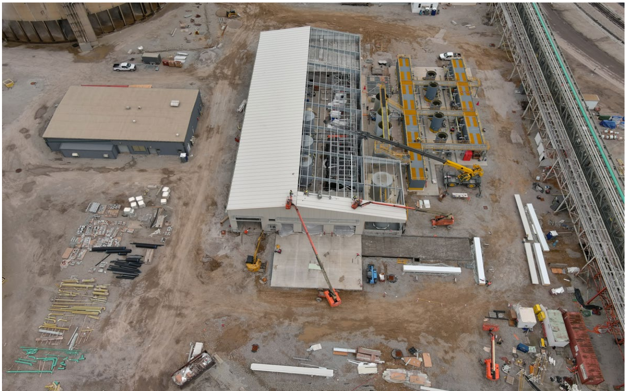
Mill Creek – ELG Water Treatment – April 2023
