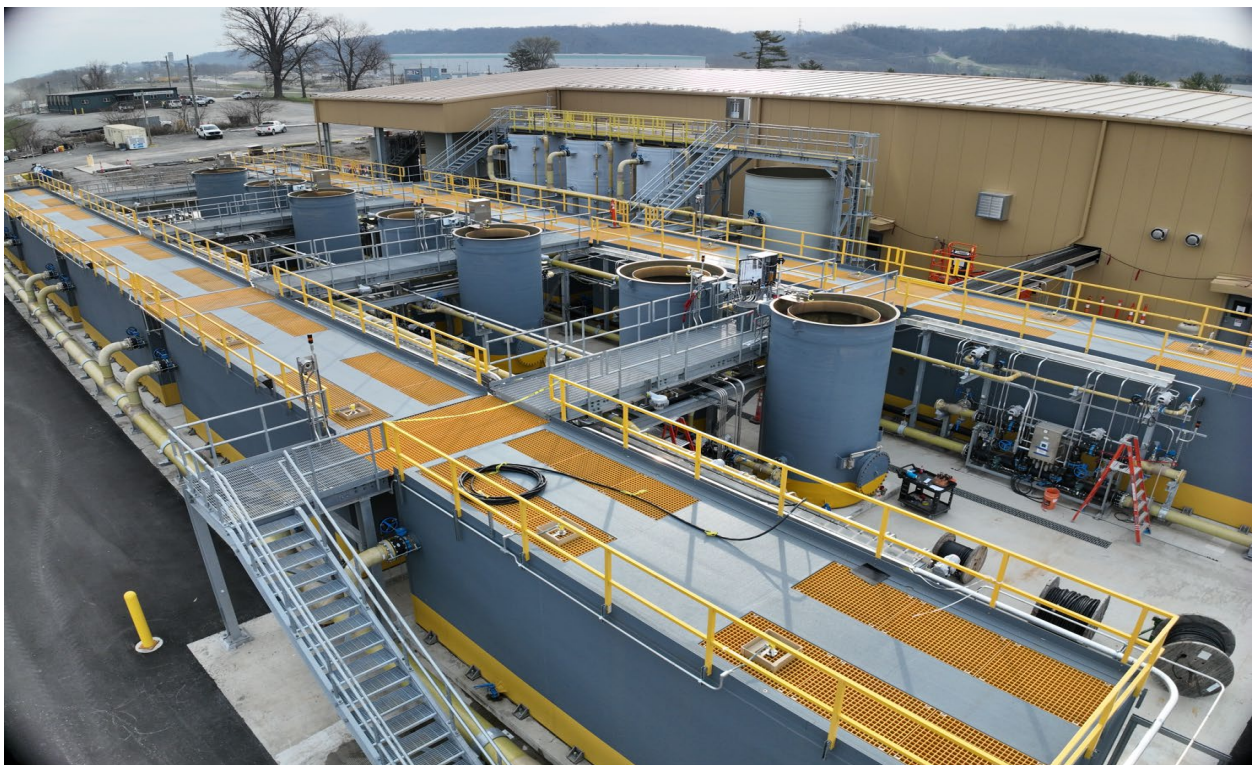
Ghent – ELG Water Treatment – March 2024
