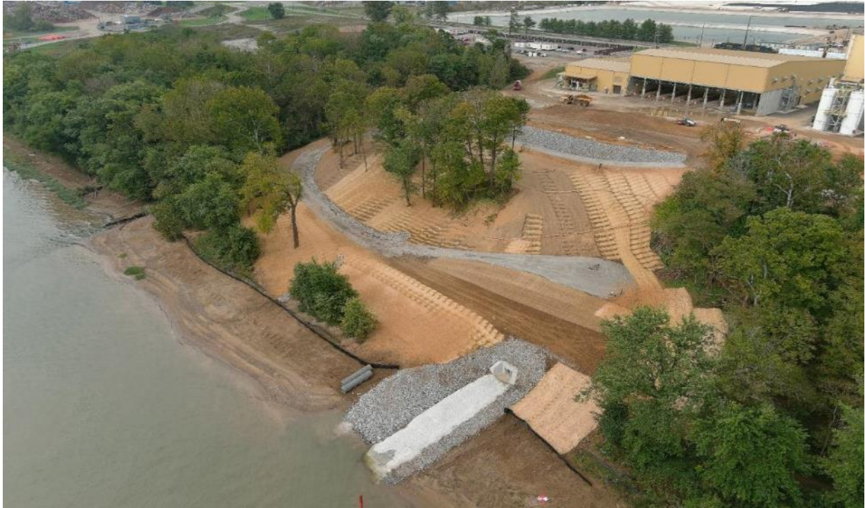
Ghent Outfall 001 Diffuser – Land Overview Looking Southeast – October 2021
