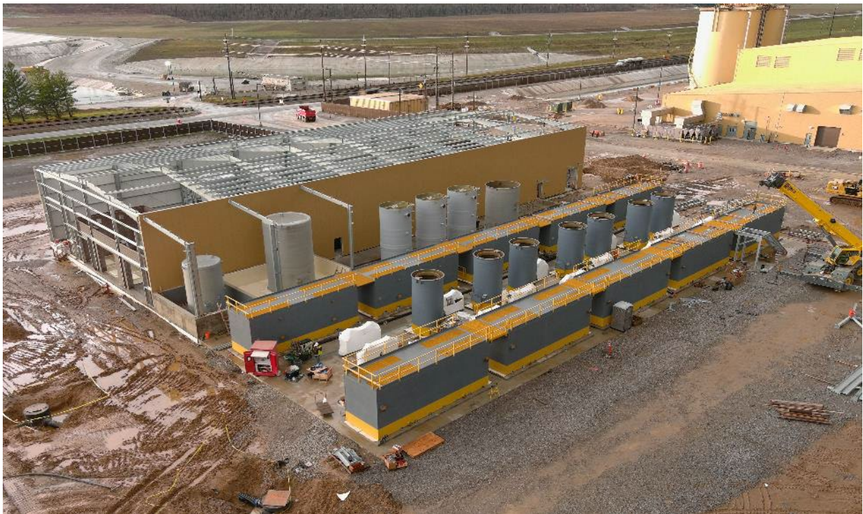
Ghent – ELG Water Treatment– December 2022
