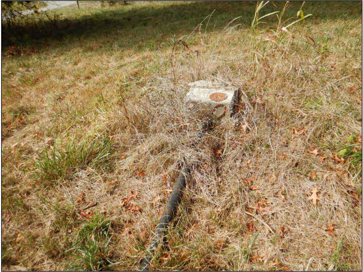
Heating oil tank at old residence
