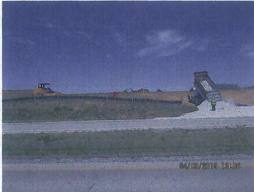
Photo Location 6. View of proposed Aero Station north of Aero Parkway. Photograph taken facing north.
