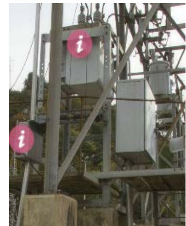
12kV Hazard CB C 11
