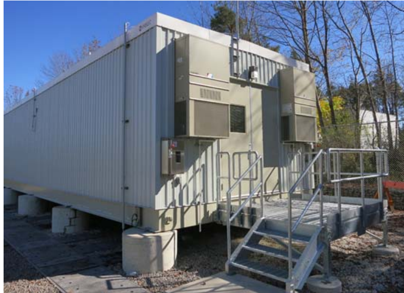
Figure 1 - Drop-In Relay/Control Room
