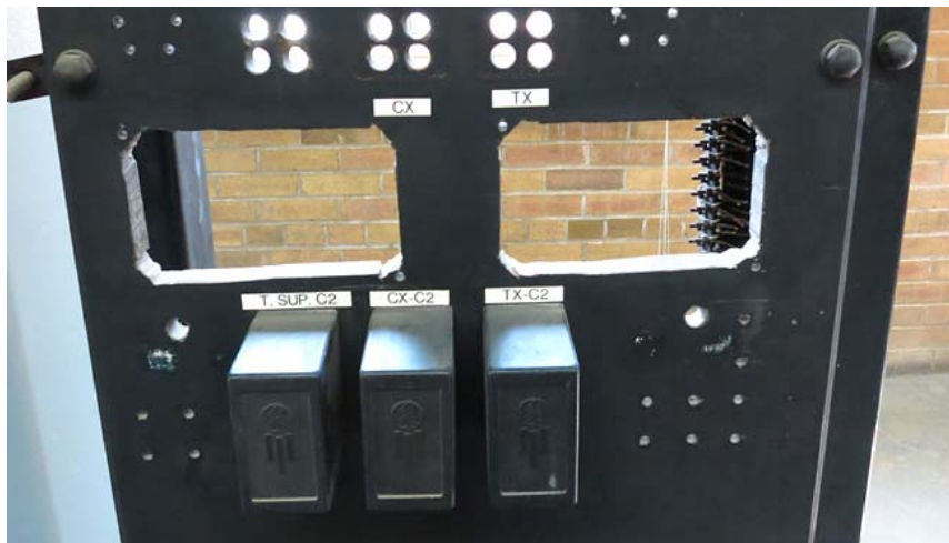
Figure 4 - Ebony-Asbestos Relay Panel
