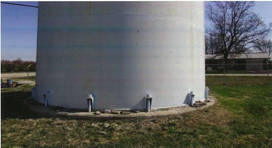
Photos show the area around the tank foundation is properly graded and in compliance with AWWA D100-11; 12.7.1: Height aboveground.
