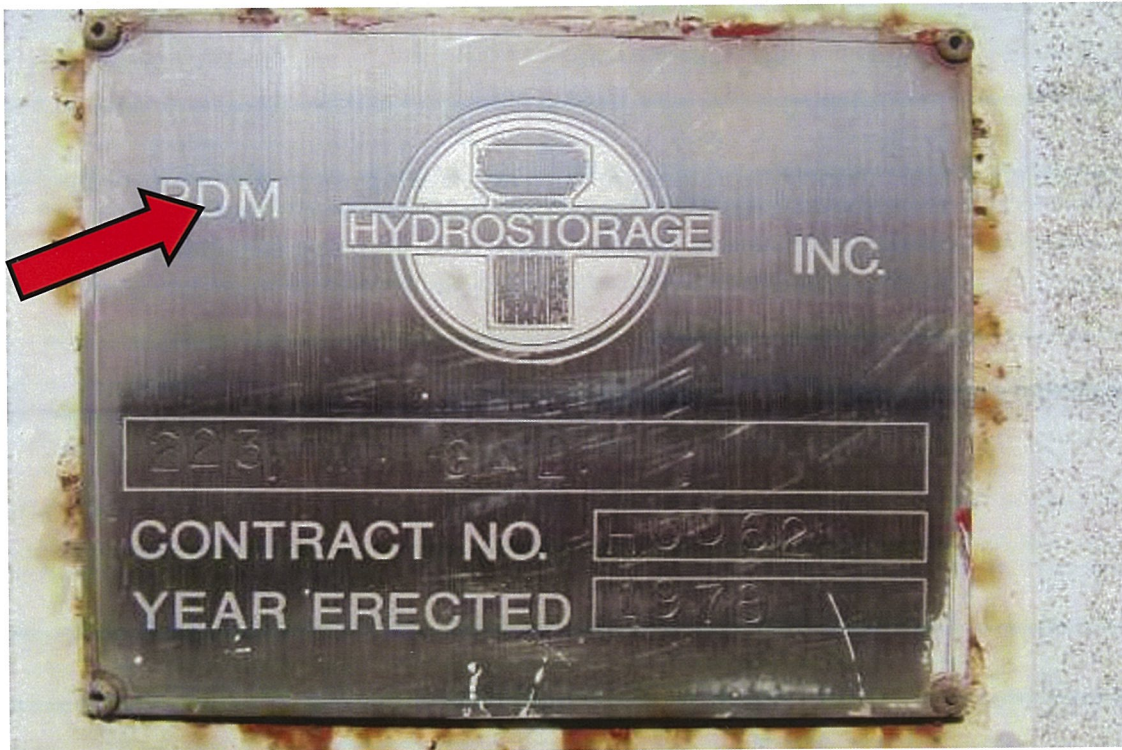
Photo shows the tank nameplate, which appears to be in good condition.
