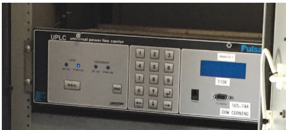
Figure 32: Power line carrier set.
