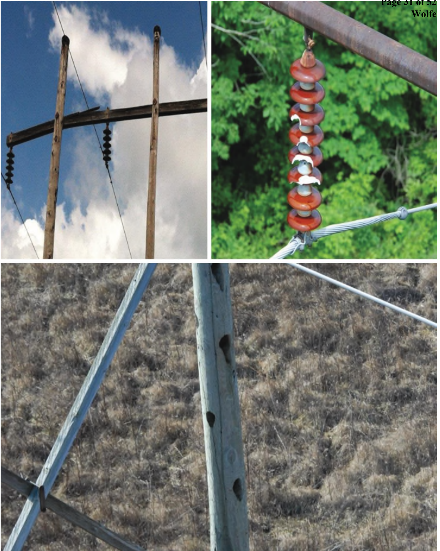
Figure 24: Examples of defective line equipment (deteriorated wood cross arm, damaged string of porcelain bell insulators and woodpecker damage on the pole).
