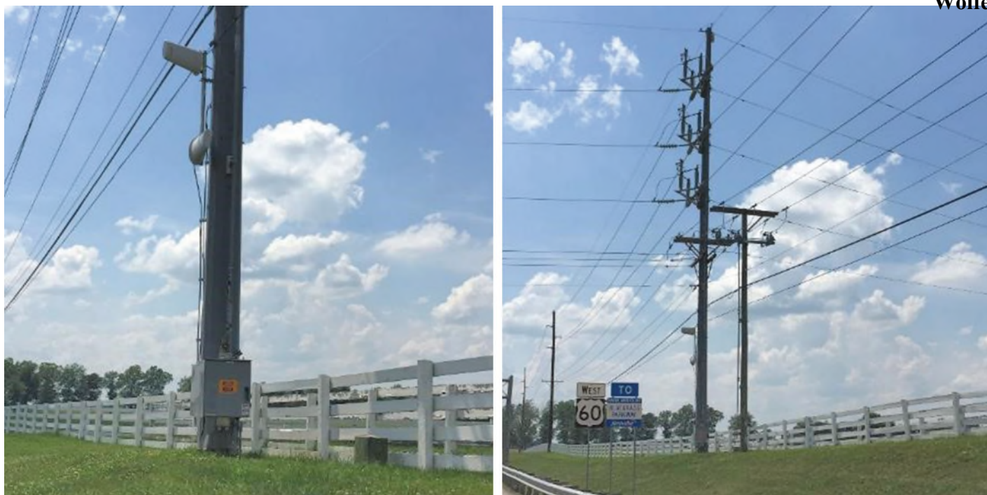
Figure 22: Example of a recent MOS installation in Lexington.
