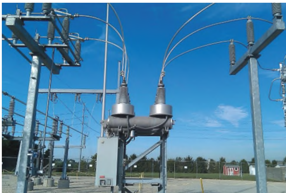
Figure 21: New circuit breaker installation inside the substation.
