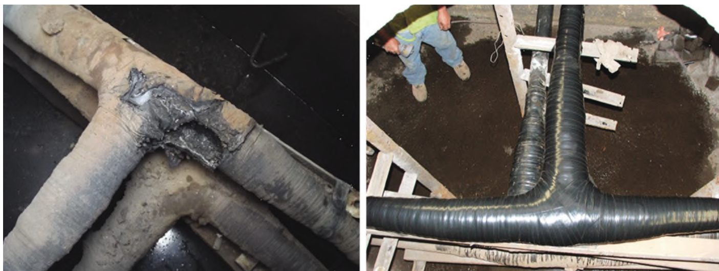
Figure 37: Example of a failed underground transmission splice.
