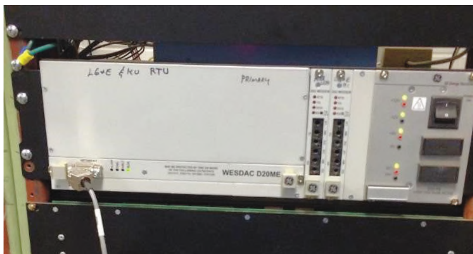
Figure 31: GE D20 remote terminal unit.
