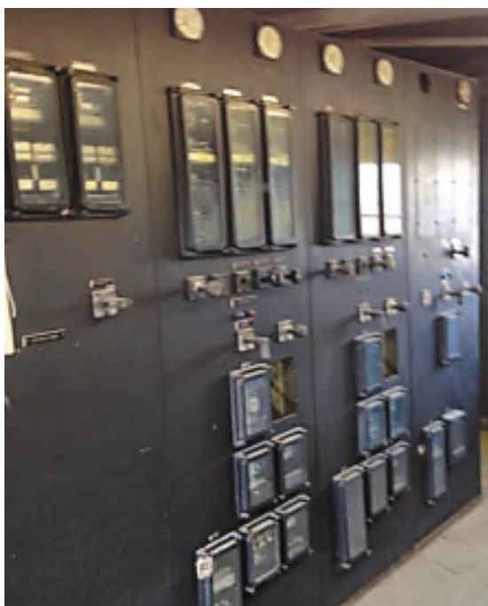
Figure 29: Electro-mechanical relay panels.
