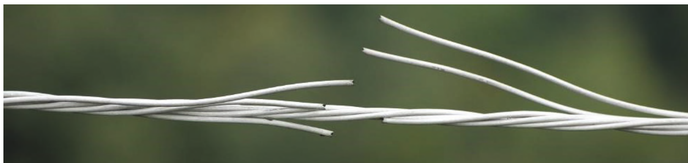
Figure 26: Example of a shield wire with broken strands.
