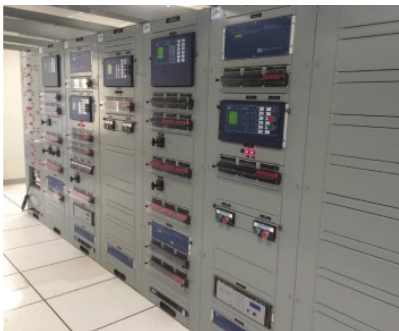
Figure 30: Microprocessor relay panels.
