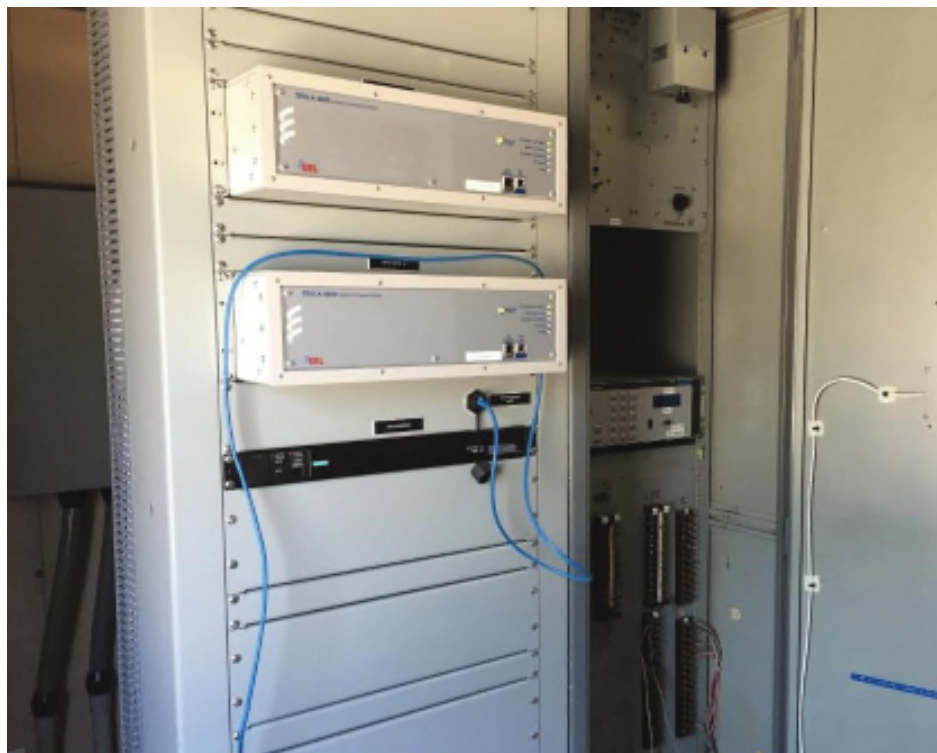
Figure 33: Tesla digital fault recorder.
