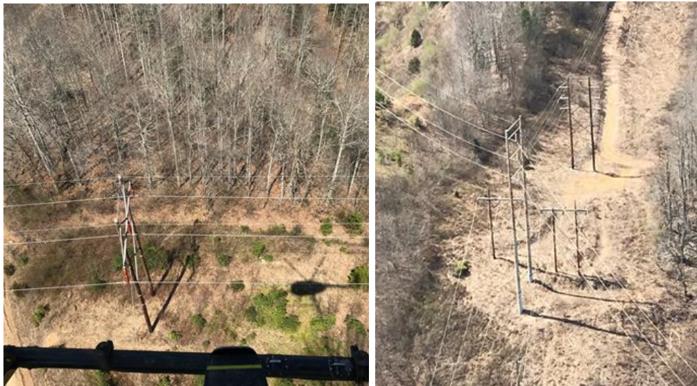
Figure 3. Example of Vegetation Conditions on Completed Circuits Observed During 2018 Aerial Workload Suvery.
