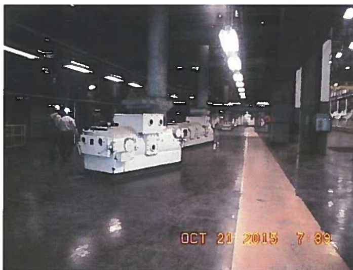
Coal Feeders at Mill Creek Generating Station
