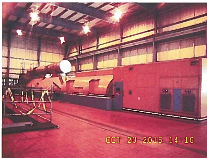
Unit 3 Turbine at Ghent Generating Station
