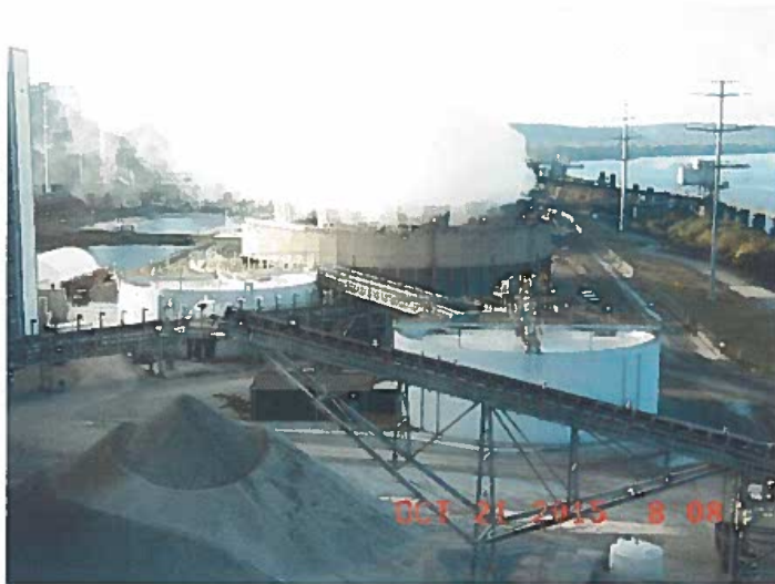
Limestone Slurry and Unit 4 Cooling Tower at Mill Creek Generating Station
