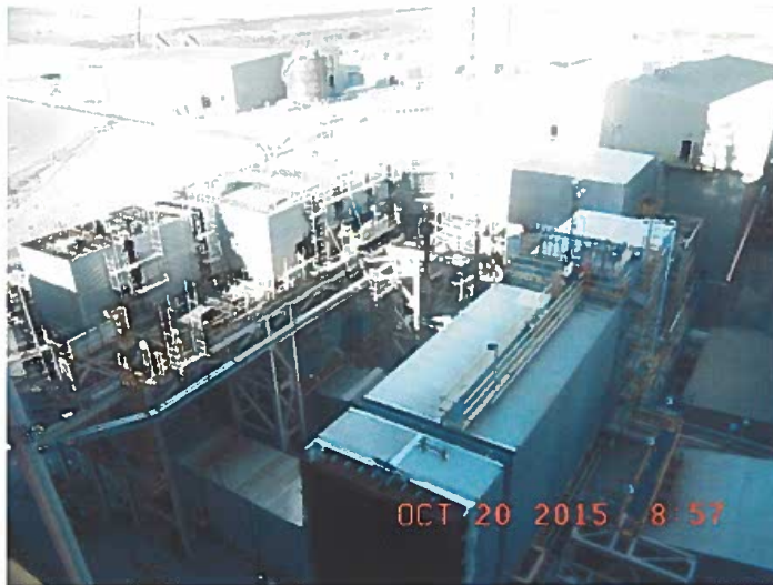
Air Exhaust/ID Fan at Brown Generating Station
