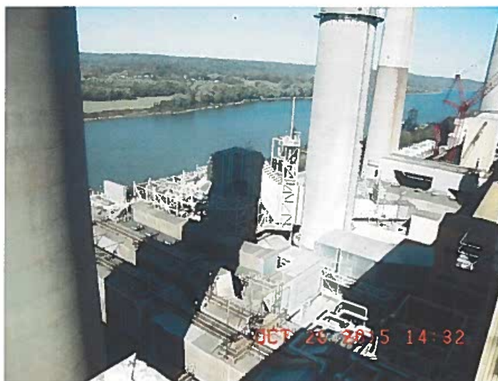
Unit 3 Scrubber at Ghent Generating Station
