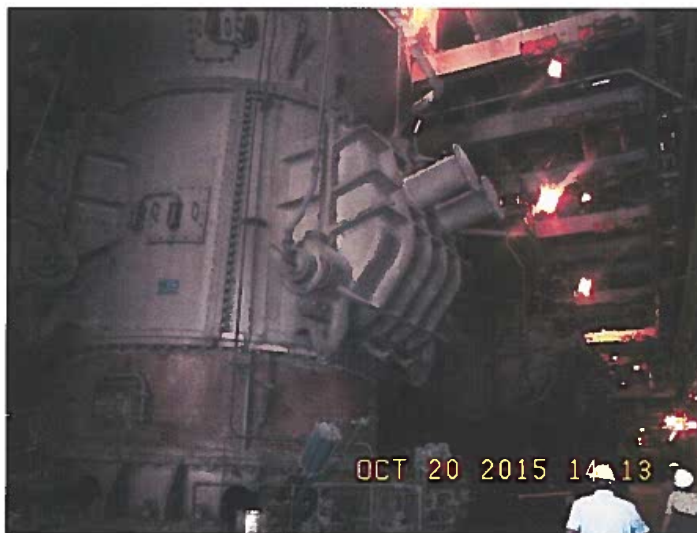
Pulverizers Unit 4 at Ghent Generating Station
