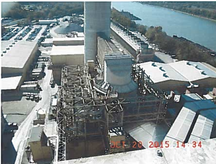
Unit 4 Scrubber at Ghent Generating Station
