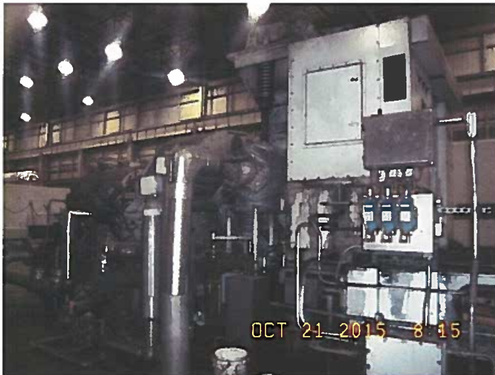
Steam Driven Boiler Feed Pump (Unit 3) at Mill Creek Generating Station
