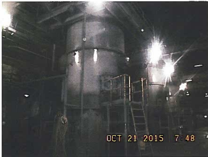
Unit 3 Pulverizers at Mill Creek Generating Station
