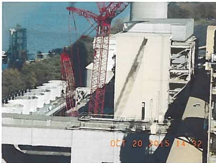
Unit 1 Scrubber at Ghent Generating Scrubber
