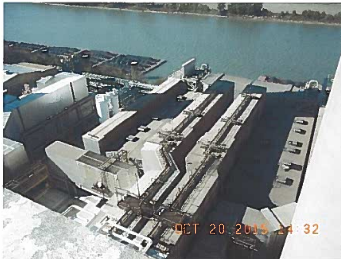
Unit 4 Precipitator at Ghent Generating Station
