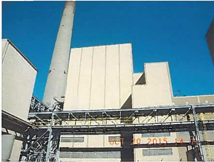
Unit 4 Boiler at Ghent Generating Station
