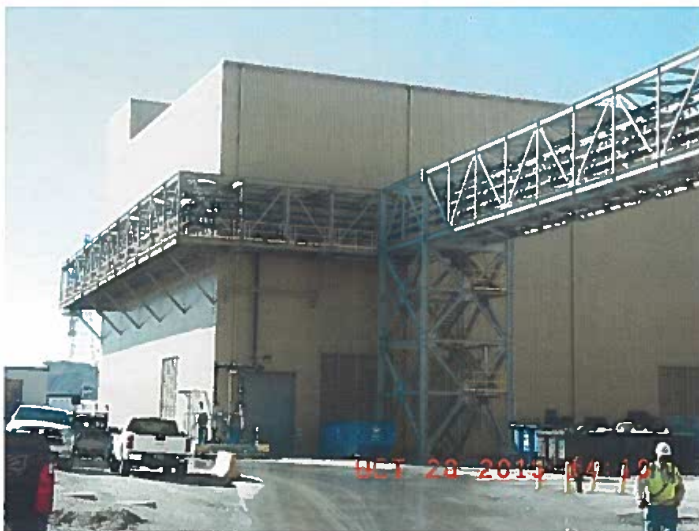
Limestone Prep Building at Ghent Generating Station
