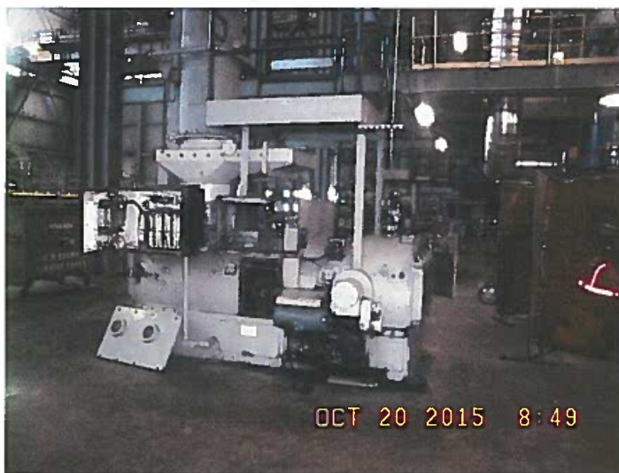
Unit 3 Coal Feeders at Brown Generating Station
