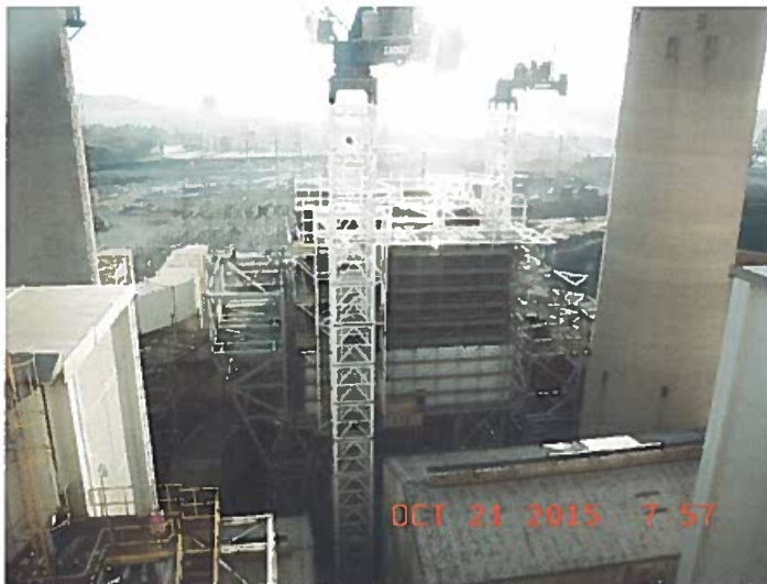
Unit 3 Baghouse at Mill Creek Generating Station
