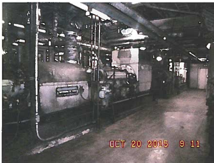
Boiler Feed Pumps at Brown Generating Station
