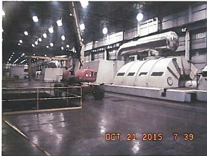
Units 1 & 2 Turbines at Mill Creek Generating Station
