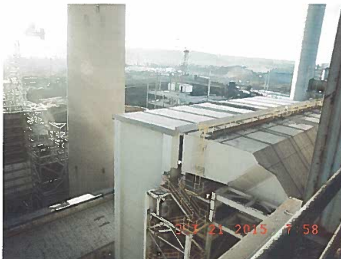
Unit 3 SCR at Mill Creek Generating Station
