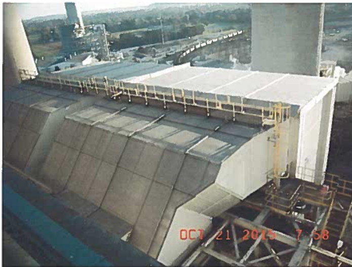
Unit 2 SCR at Mill Creek Generating Station
