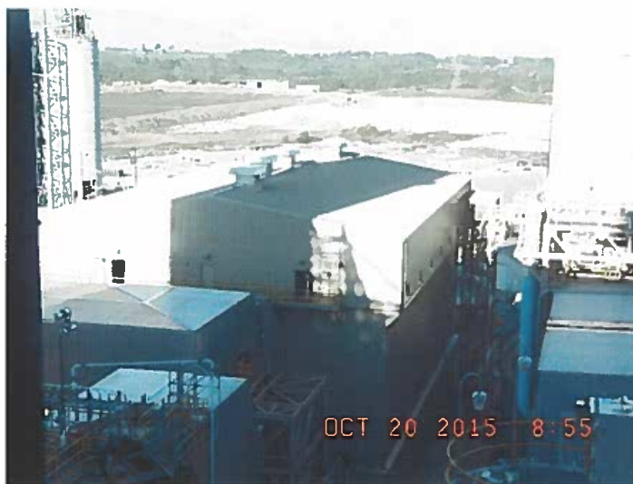
Baghouse at Brown Generating Station
