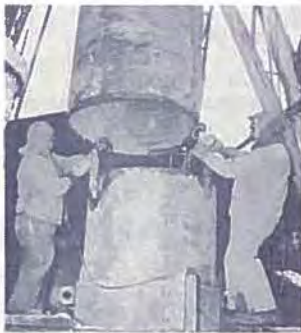
Welders preparing section of 42" diameter main shaft for welding and insertion in 60" diameter surface casing.
