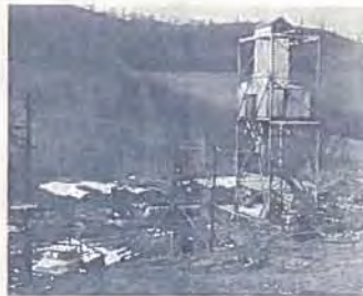
Erection of mining hoist used to lift buckets of mined limestone from the Constance Cavern.
