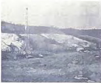
Erection of the Drilling rig used to drill the main shaft. The rugged terrain at the cavern site is shown in this over-all photograph.
