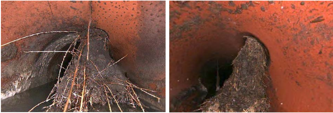
Root intrusion breaking the pipes, causing deposition resulting in H 2 S formation
