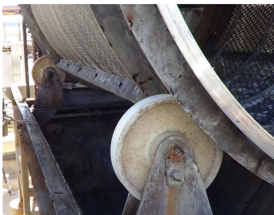
Raw wastewater screen located in a highly corrosive area with a very short life.
