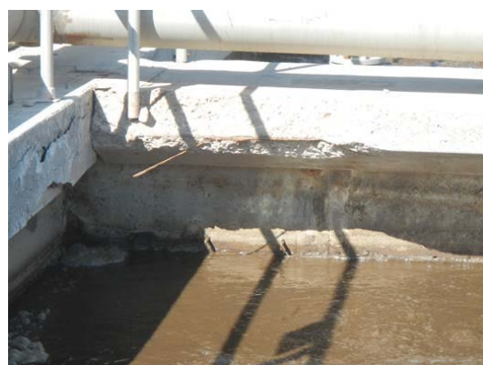
Concrete corrosion at a wastewater treatment plant
