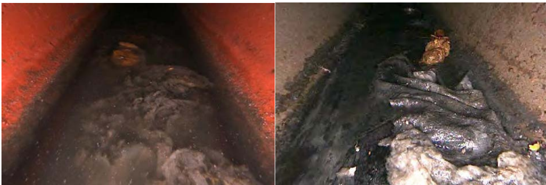
Solids deposition - lack of flow in the summer time causing H 2 S formation.
