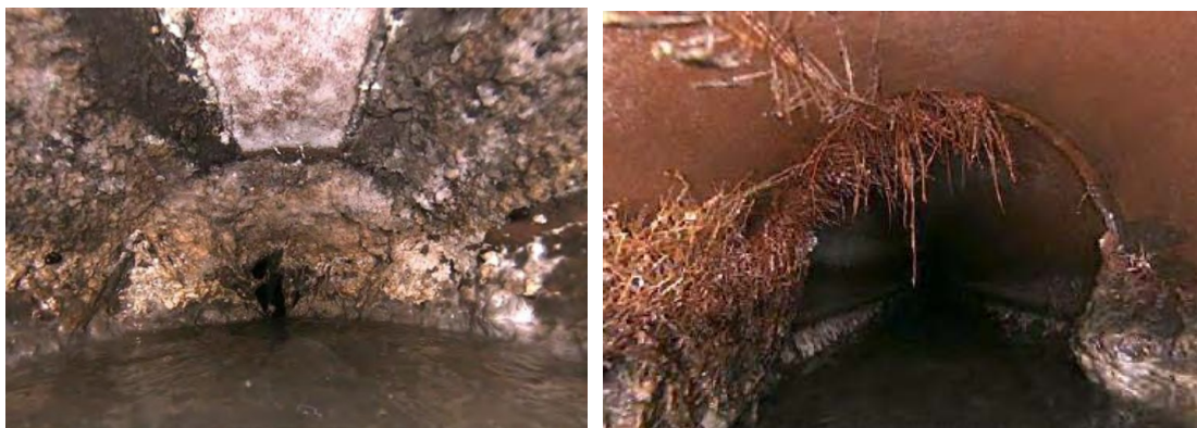
Root intrusion clogging the pipe causing solids deposition and increasing H 2 S production. Photos from CCTV inspection of EPCOR sewers
