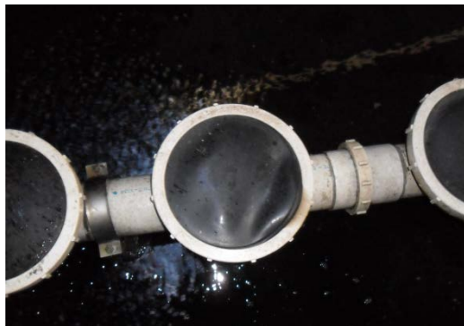
Air diffuser damage – Expected life 5-8 years
