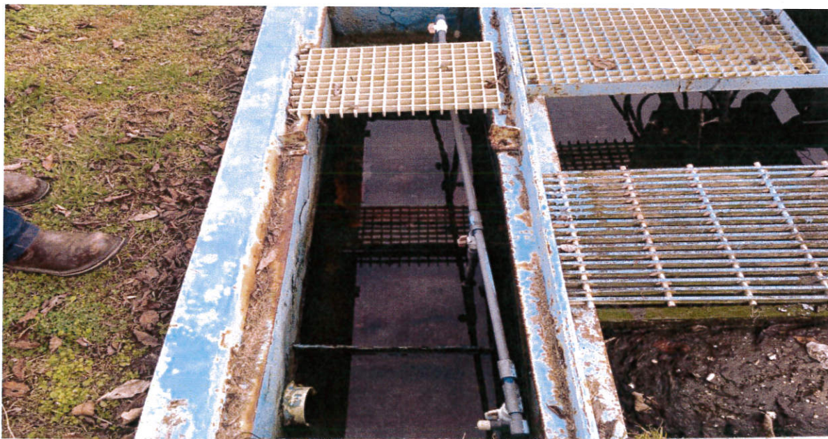
Modern MHP - Chlorine Contact Chamber
