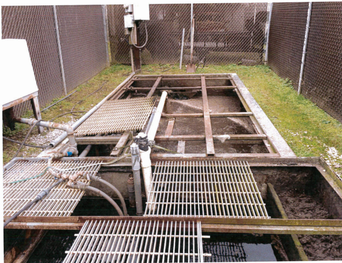
Keene Village WWTP - Clarifier and Aeration basin
