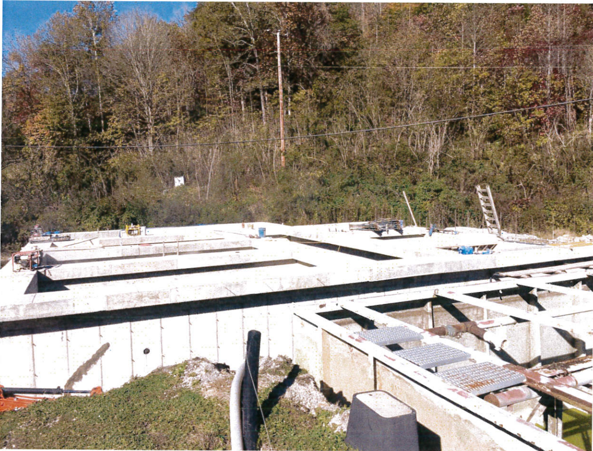
Douglas WWTP Upgrade Project – Douglas wwtp being converted to a membrane technology plant called a Membrane Bioreactor (MBR)
