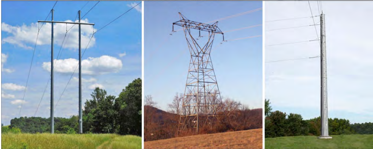
Figure 2. Typical Transmission Structures
