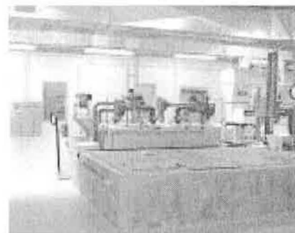
In 1999, Henry County Water Company constructed a new 2.4-MGD single pass pulsator flocculator/clarifier water treatment plant with dual-media gravity filtration.
