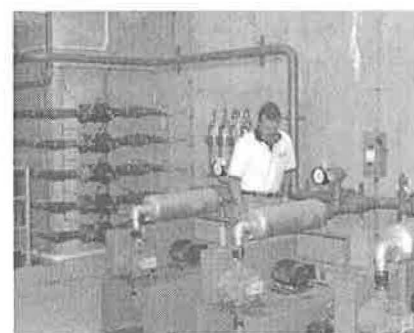
System Manager Richard Webber inspects the system's pulsator clarifier blowers. Alliance provided planning and management for the financing, design and construction of this new system, resulting in a capital savings of more than $1.5 million.
