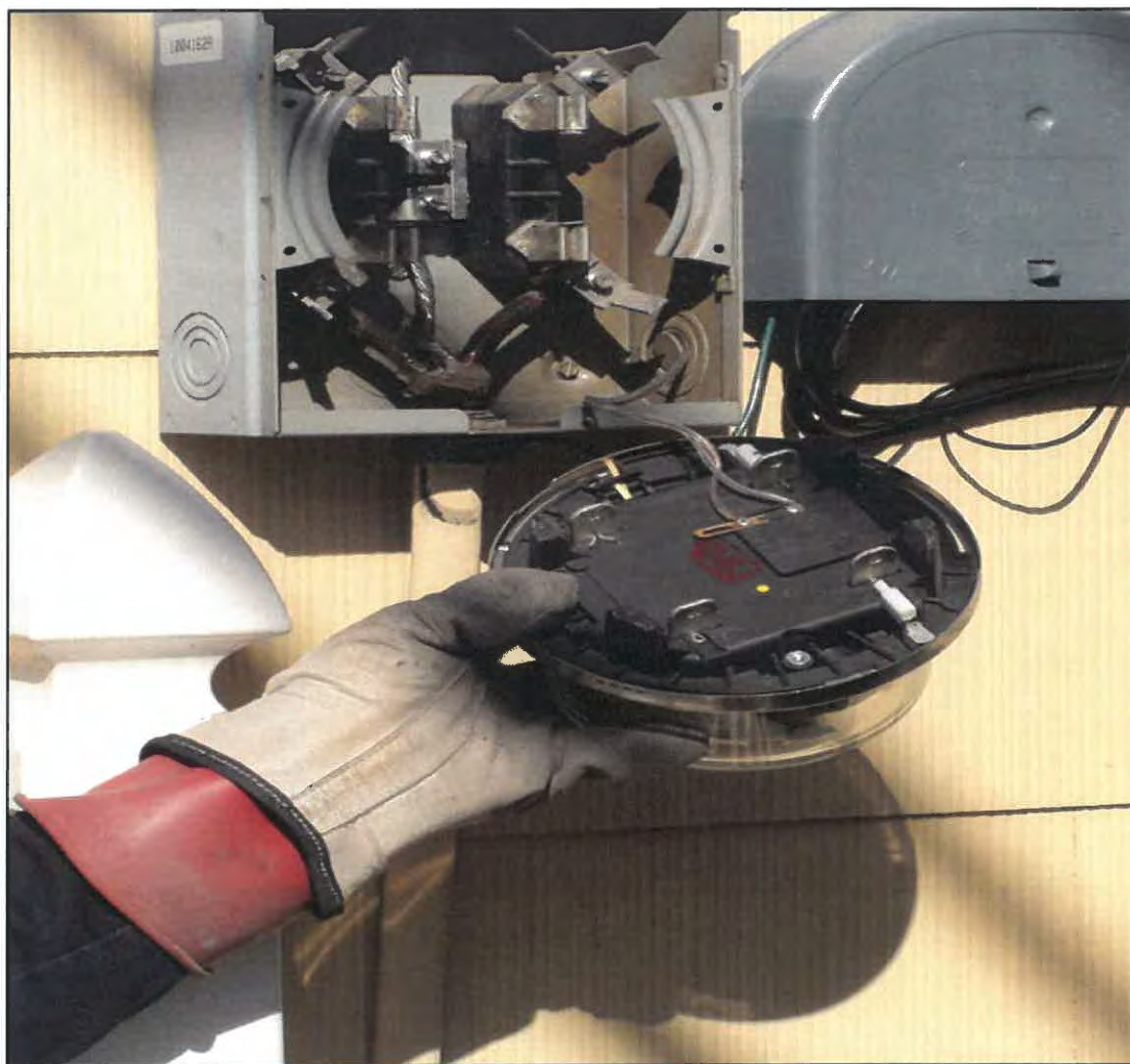
Figure 4-8 Meter recorded in Figure 7 with wires attached to its potential clip
