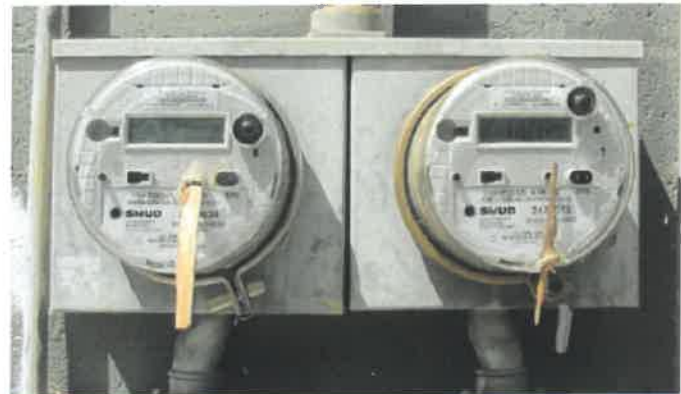
Figure 1 – Example of Attempted Power Theft
