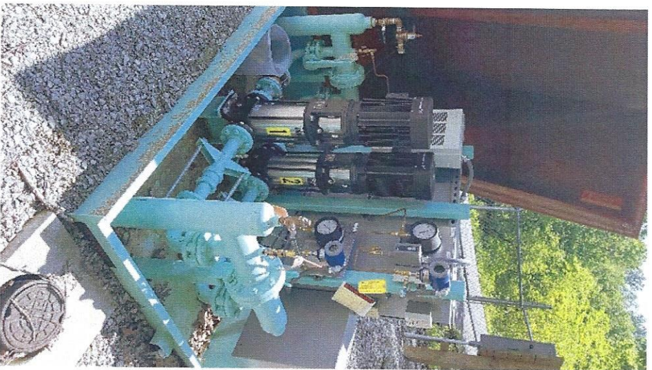
Gilgal Booster Station
