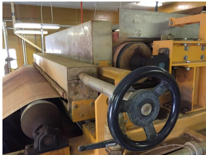
Figure 7 – Belt Cleaning Assembly / Shower Box
