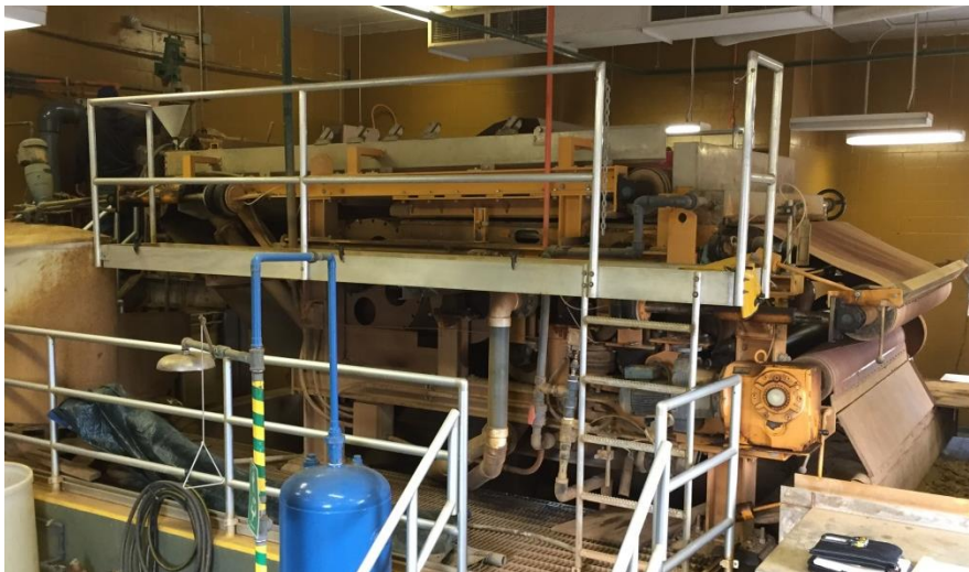
Figure 1 - Overall View of installed belt press
