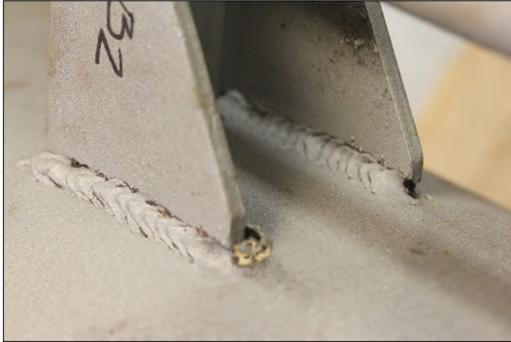
Figure 8. Image of the Lug B2 exterior weld which exhibited substantial fusion except for some undercut, and overlap.
