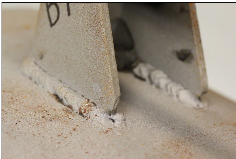
Figure 8. Image of the Lug B1 welds showing good fusion with some undercut and overlap.
