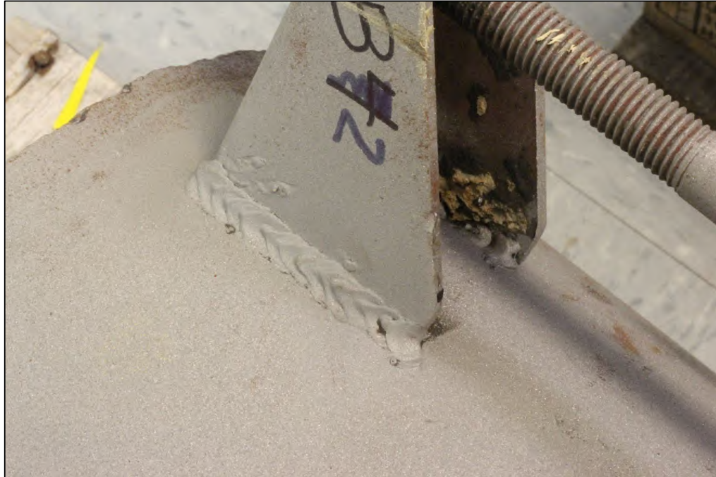
Figure 8. Image of the Lug B2 exterior bottom weld which exhibited substantial fusion except for some undercut, spatter, and arc strikes. A portion of the interior weld was obscured.
