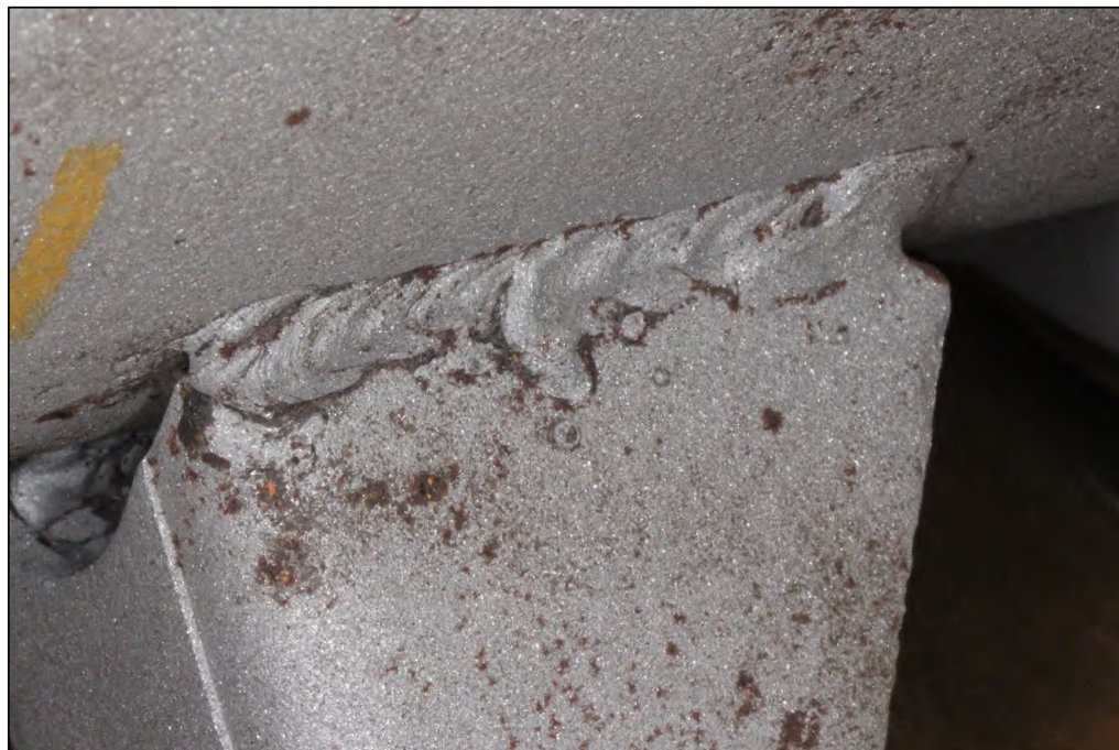
Figure 5. Image of the Lug A1 exterior bottom weld which exhibited substantial fusion except for some undercut, overlap, spatter, and arc strikes.
