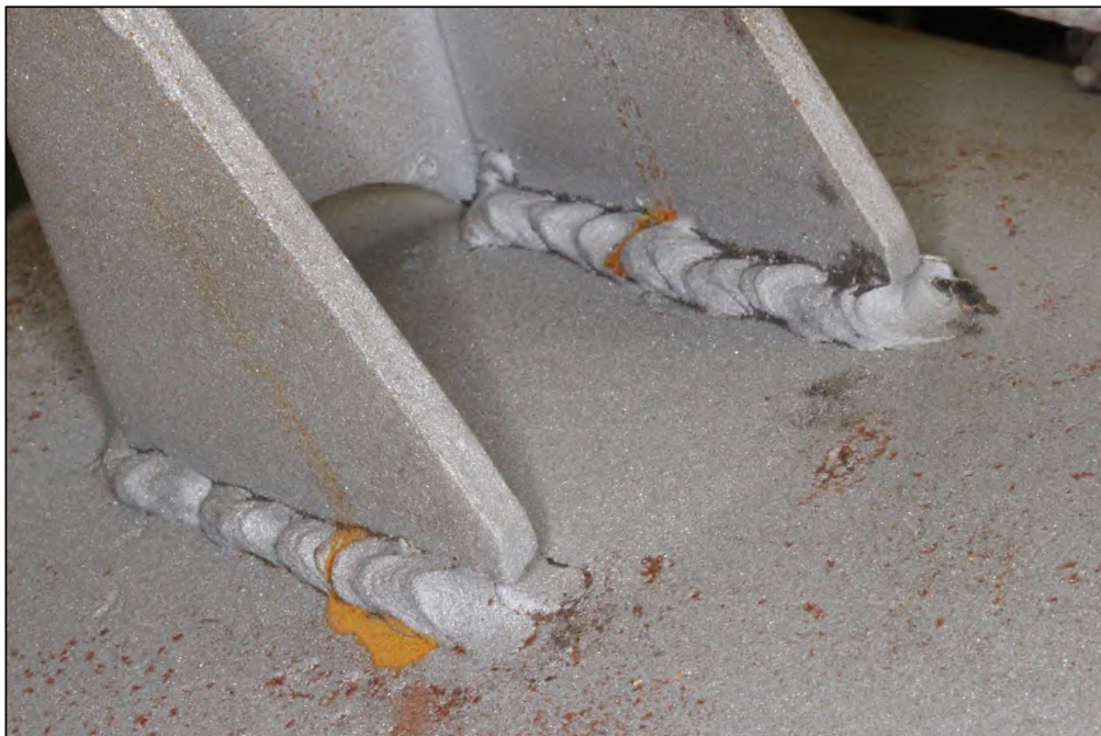
Figure 10. Image of the Lug B5 exterior bottom weld which exhibited substantial fusion except for some undercut and overlap.
