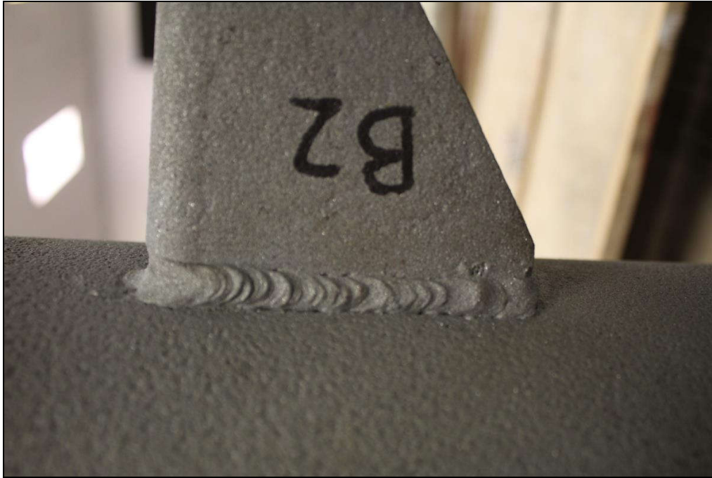
Figure 7. Image of the Lug B2 exterior top weld which exhibited substantial fusion except for some undercut and arc strikes.
