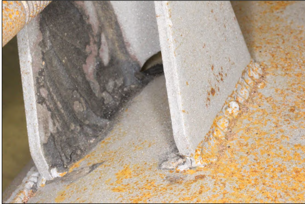
Figure 10. Image of the Lug B3 welds which exhibited substantial fusion except for some undercut, overlap, arc strikes, and spatter. The interior weld to the left was obscured.
