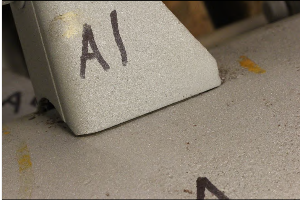
Figure 6. Image of the Lug A1 exterior top weld which was not welded.
