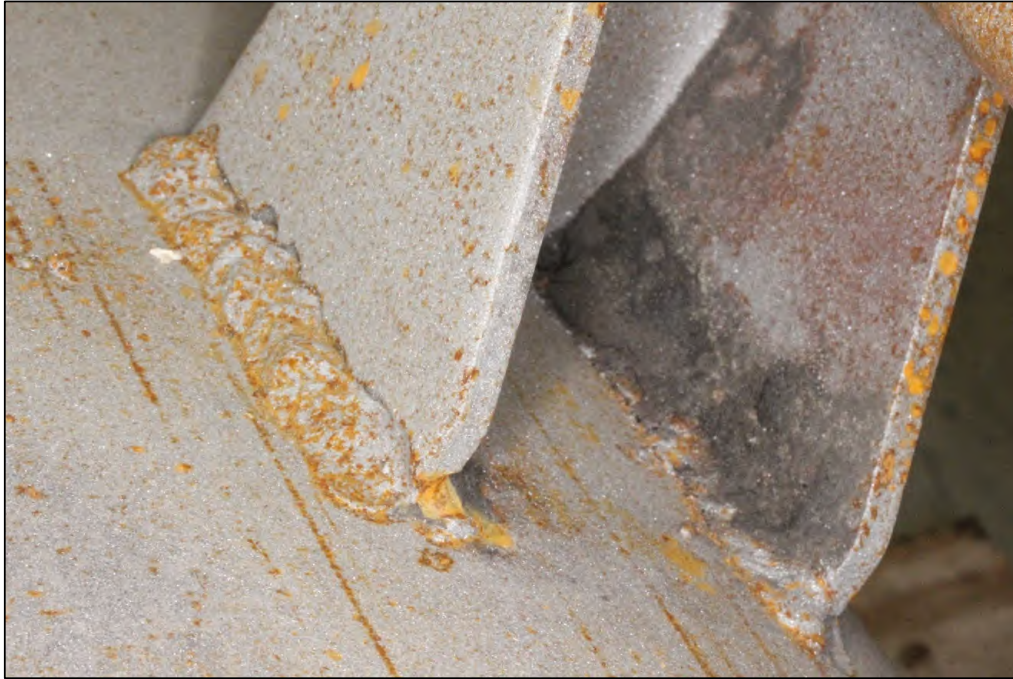
Figure 6. Image of the Lug A3 exterior and interior welds which exhibited overlap, undercut, spatter, and arc strikes.
