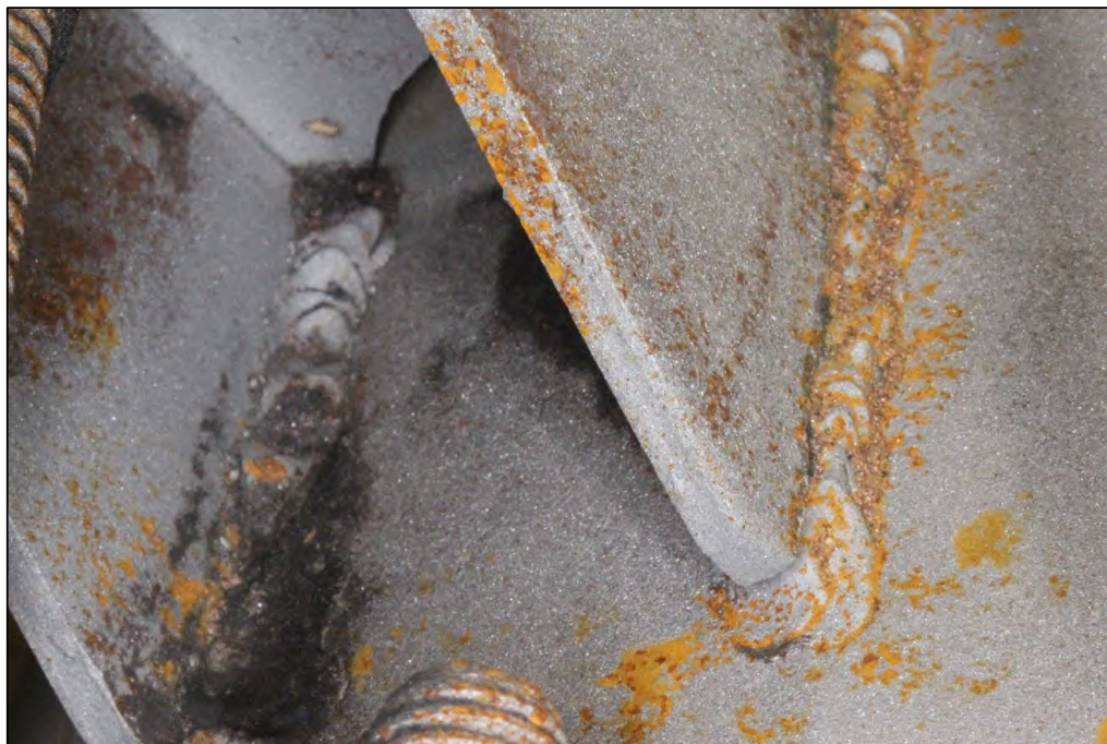
Figure 9. Image of the Lug B4 exterior top weld which was fractured and exhibited substantial fusion except for some undercut, arc strikes, and spatter.
