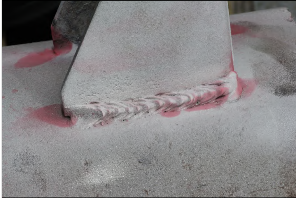
Figure 11. Image of the Lug B2 exterior top weld after dye penetrant media had been used during inspection.
