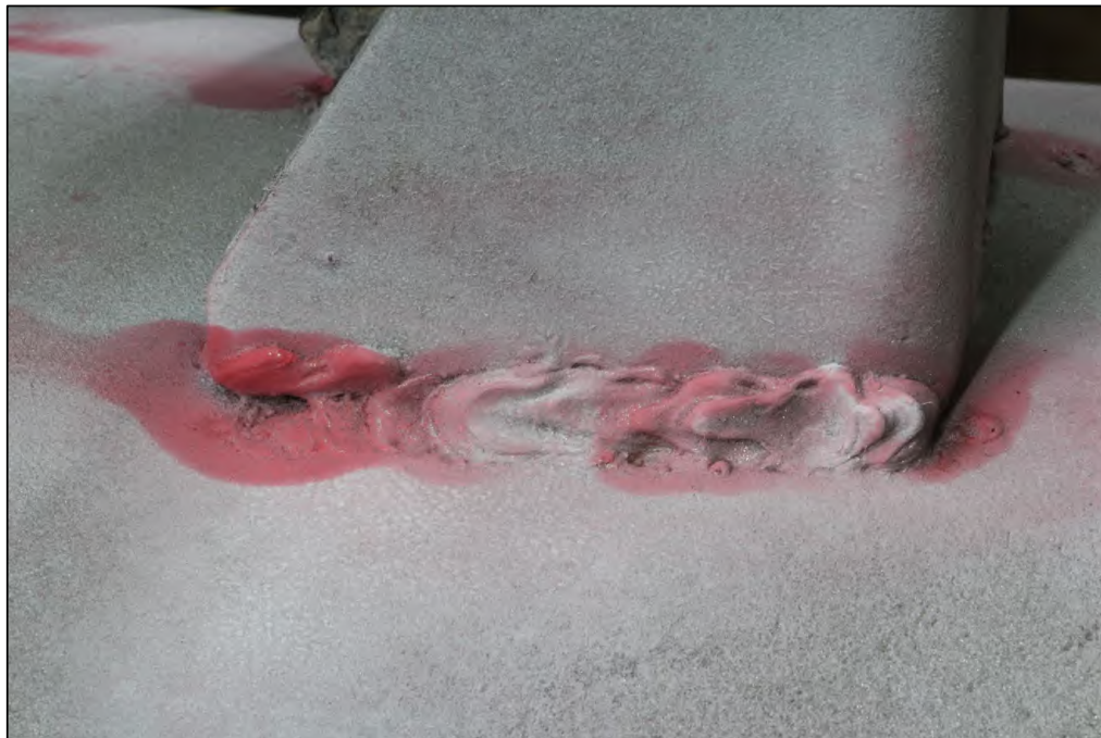
Figure 10. Image of the Lug A1 exterior weld after dye penetrant media had been used during inspection.
