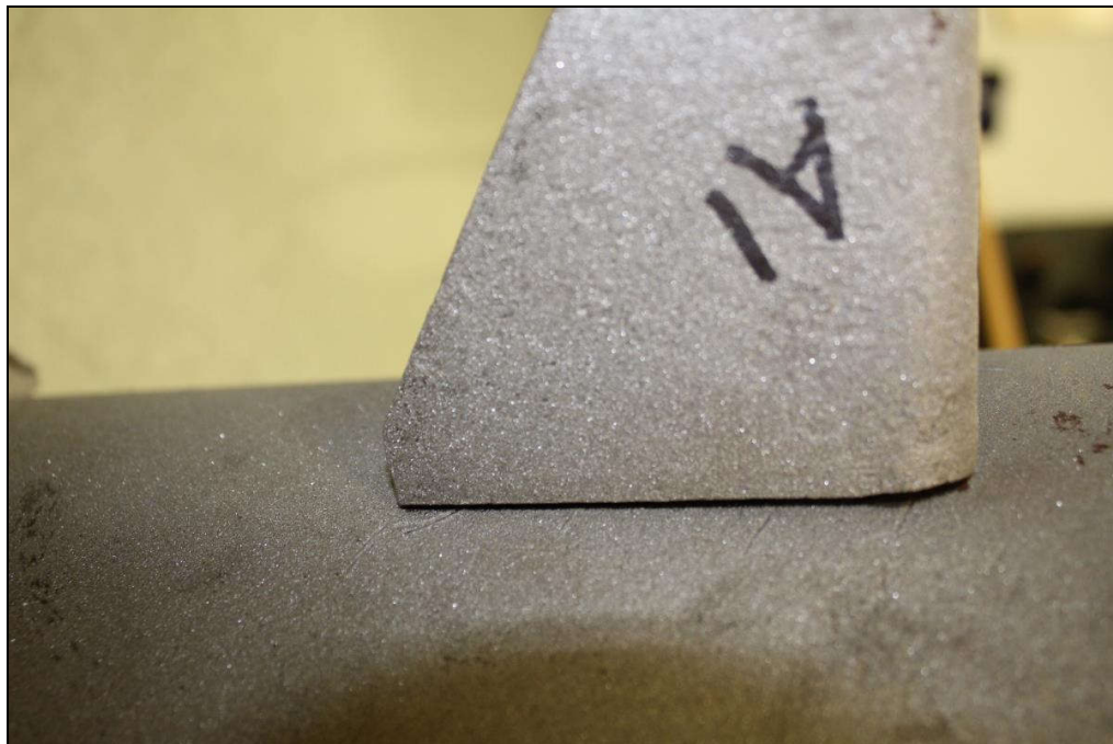
Figure 6. Image of the Lug A1 exterior bottom weld which exhibited no fusion.
