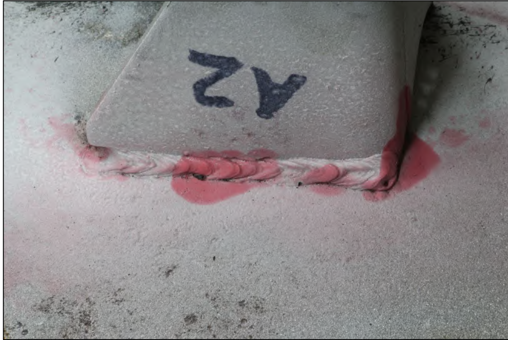
Figure 11. Image of the Lug A2 exterior top weld after dye penetrant media had been used during inspection.
