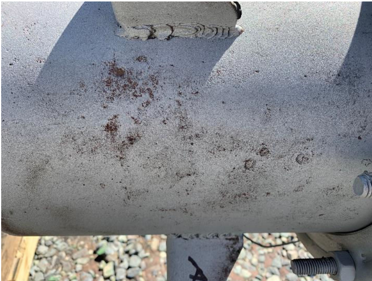
Figure 13 – General Corrosion on Pipe Side A
