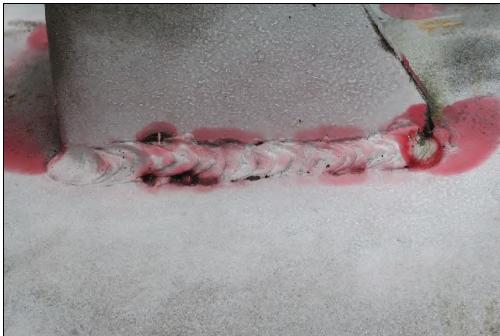
Figure 10. Image of the Lug A4 exterior top weld after dye penetrant media had been used during inspection.
