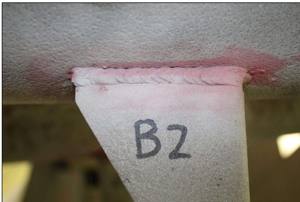
Figure 10. Image of the Lug B2 exterior top weld after dye penetrant media had been used during inspection.
