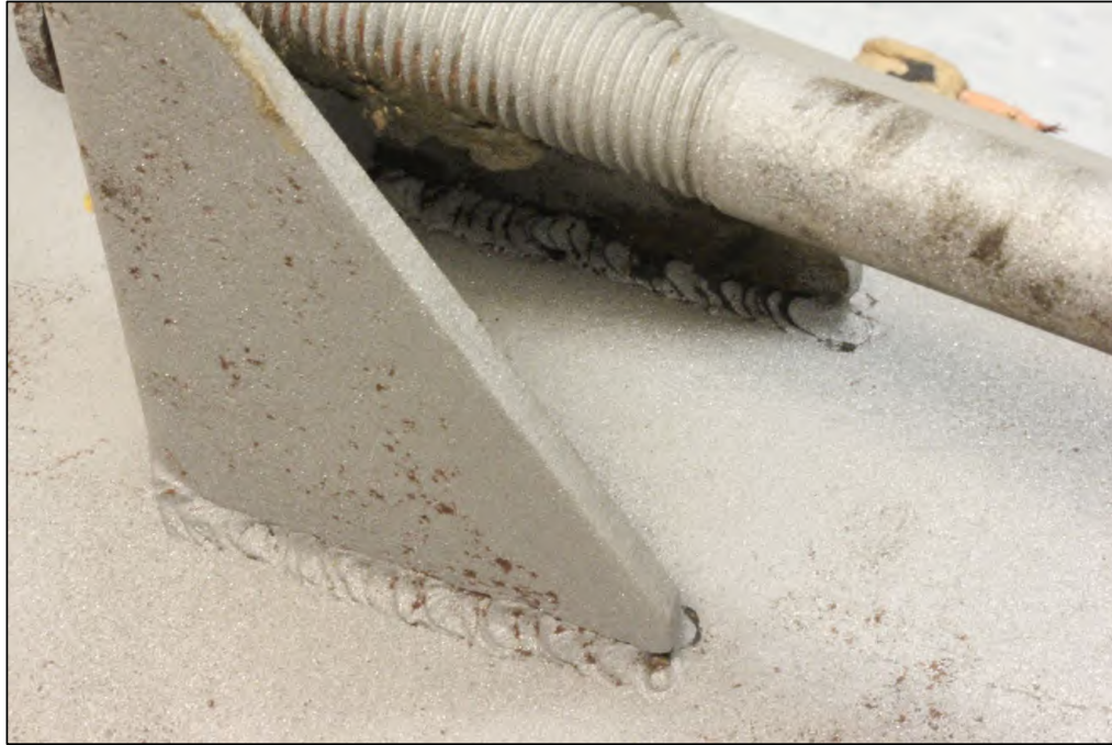
Figure 8. Image of the Lug B2 welds which exhibited substantial fusion along with undercut and overlap.
