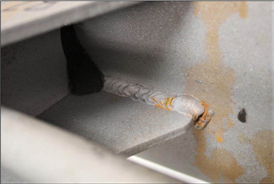
Figure 9. Image of the Lug B2 interior bottom weld which exhibited substantial fusion.
