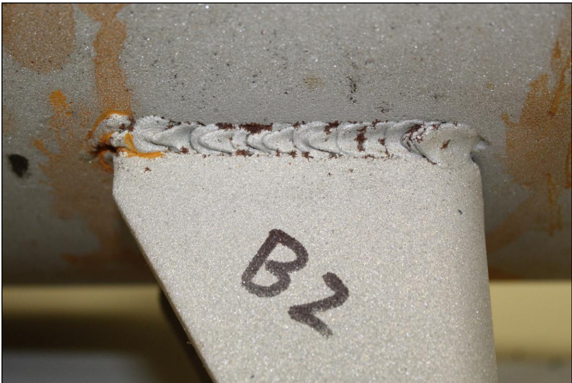
Figure 8. Image of the Lug B2 exterior bottom weld which exhibited substantial fusion except for some undercut.
