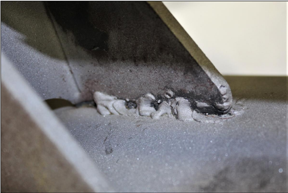
Figure 7. Image of the Lug A4 exterior top weld which exhibited substantial fusion except for some undercut and spatter.
