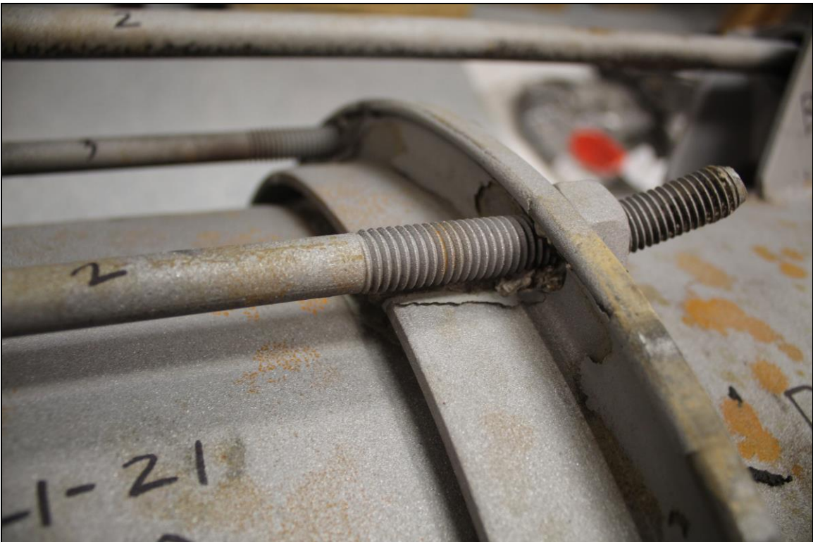
Figure 12. Image of the bent end of Bolt 2.
