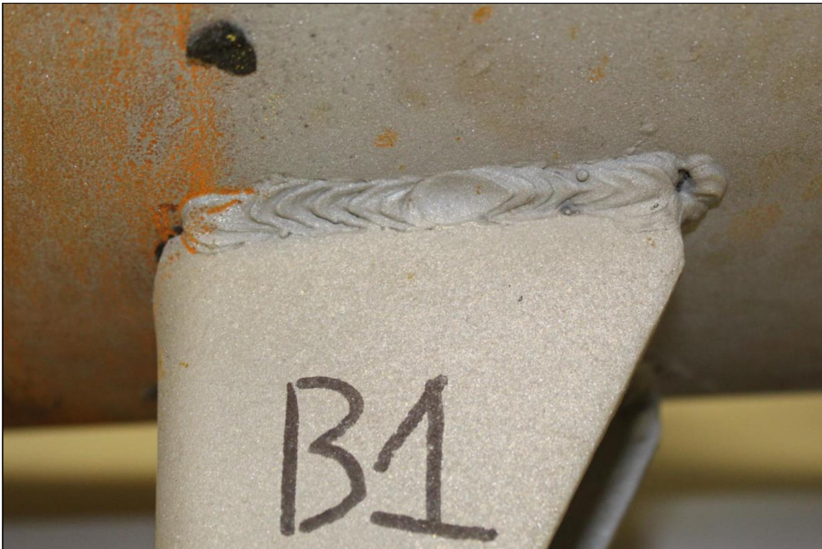
Figure 8. Image of the Lug B1 exterior bottom weld which exhibited substantial fusion except for some undercut, and spatter.
