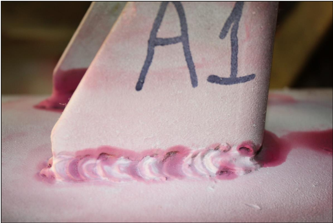
Figure 11. Image of the Lug A4 exterior top weld after dye penetrant media had been used during inspection.
