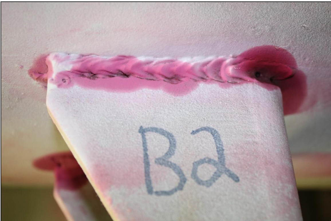
Figure 12. Image of the Lug B1 exterior top weld after dye penetrant media had been used during inspection.
