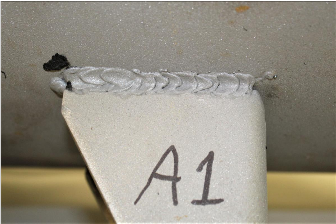
Figure 5. Image of the Lug A1 exterior bottom weld which exhibited substantial fusion except for some undercut, spatter, and arc strikes.
