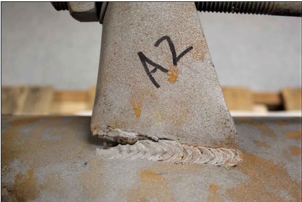
Figure 6. Image of the Lug A2 exterior top weld which was fractured and exhibited substantial fusion except for some undercut and porosity.
