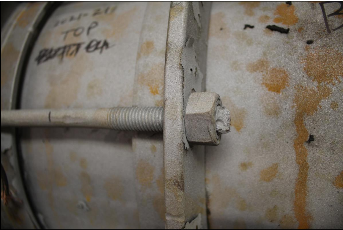
Figure 11. Image of the broken end of Bolt 1.
