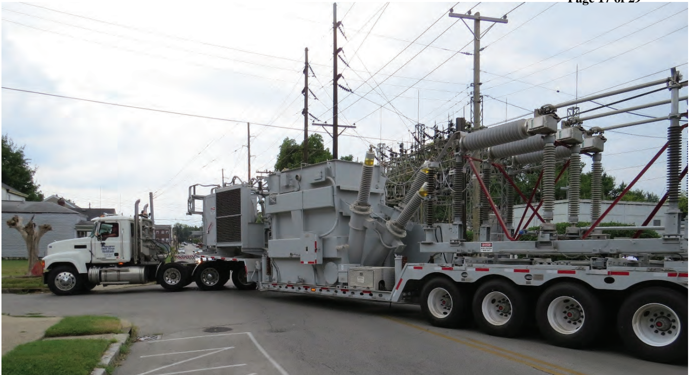
Figure 14: Mobile Transformer owned by LG&E and KU.
