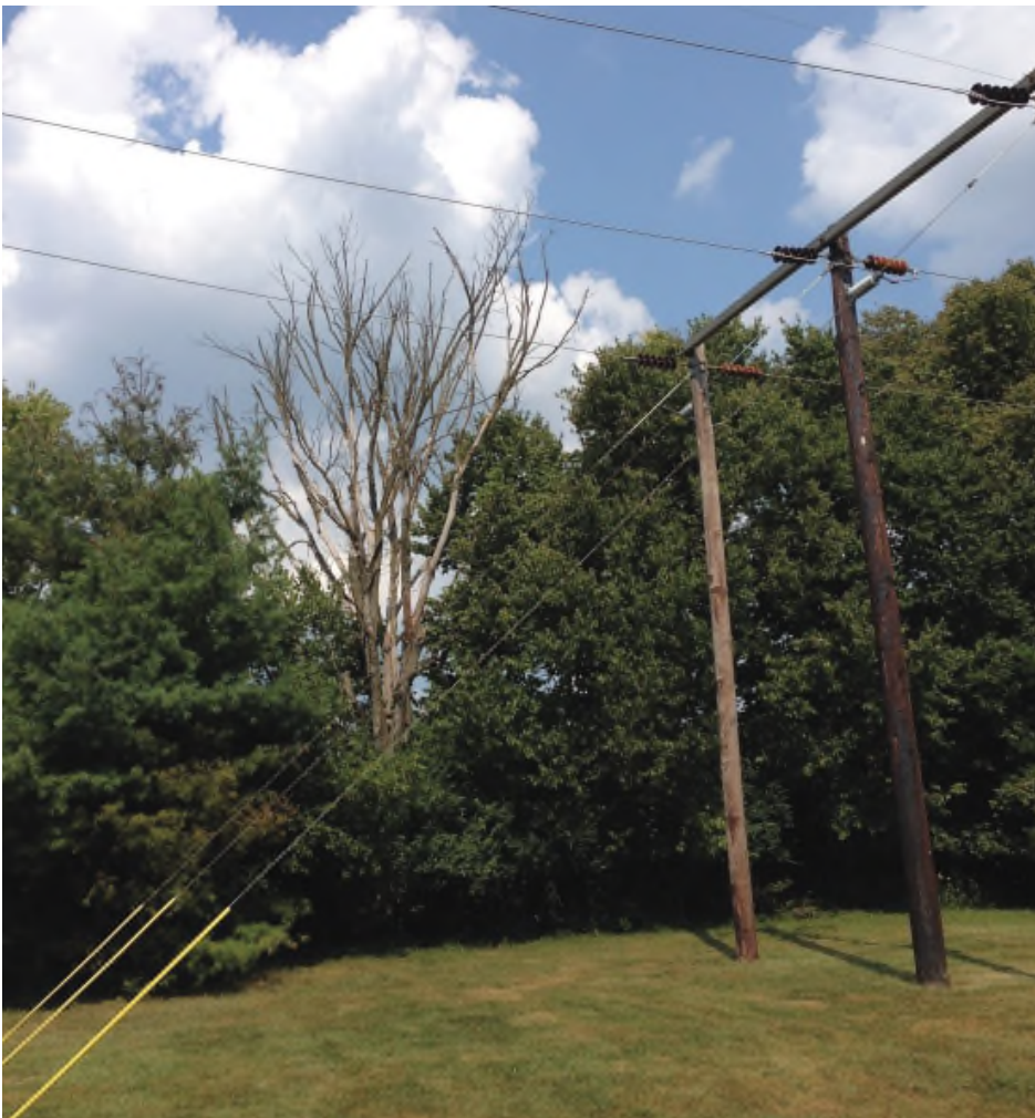
Figure 18: Example of a hazard tree adjacent to a 69kV transmission line.
