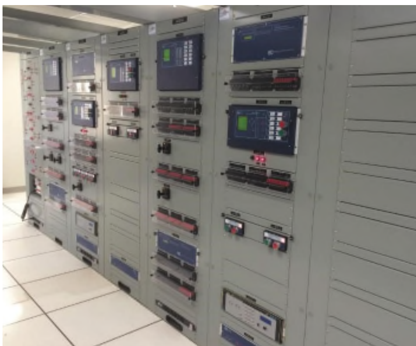
Figure 30: Microprocessor relay panels.
