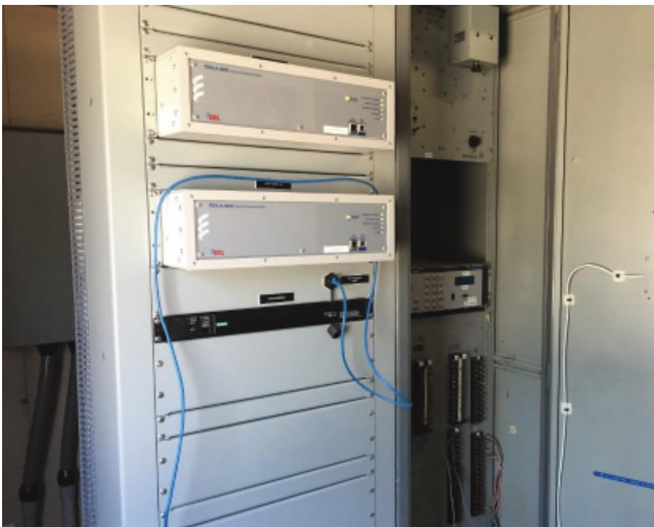
Figure 33: Tesla digital fault recorder.
