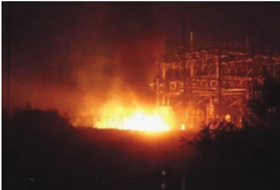
Figure 35: 69kV circuit breaker failure.
