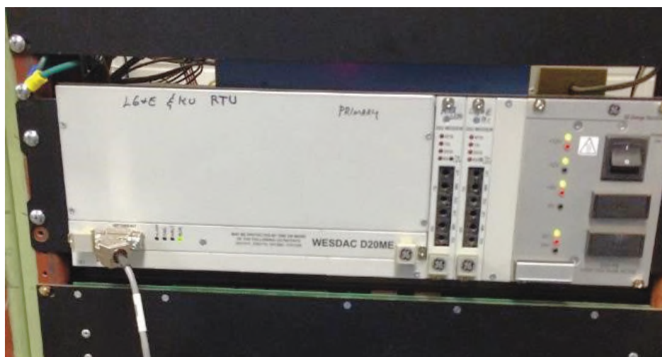
Figure 31: GE D20 remote terminal unit.
