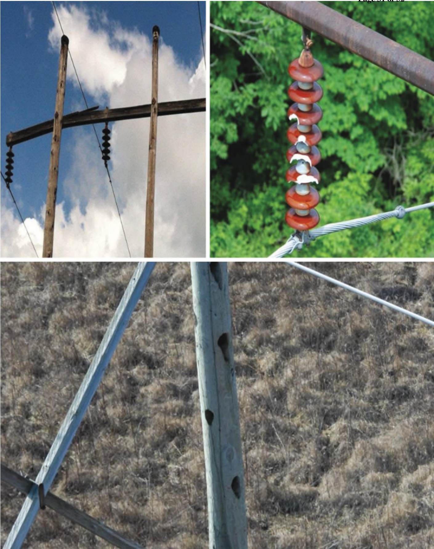
Figure 24: Examples of defective line equipment (deteriorated wood cross arm, damaged string of porcelain bell insulators and woodpecker damage on the pole).
