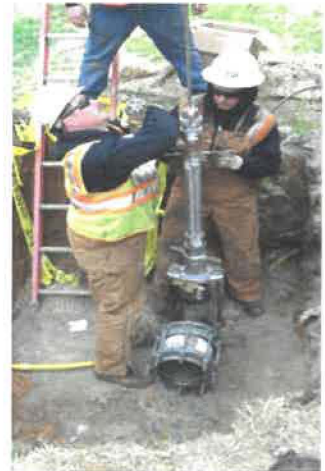
LG&E gas main replacement crews working to replace bare steel pipe with more durable and reliable plastic pipe.
