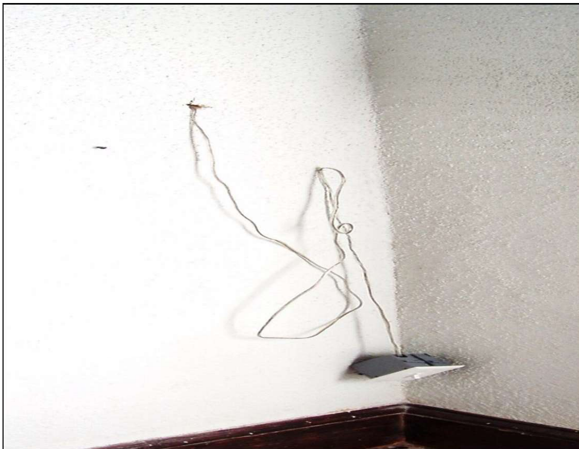
Figure 4-9 Toggle switch controlling the meter bypass
