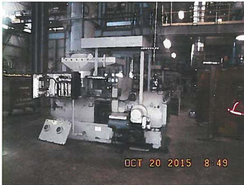
Unit 3 Coal Feeders at Brown Generating Station
