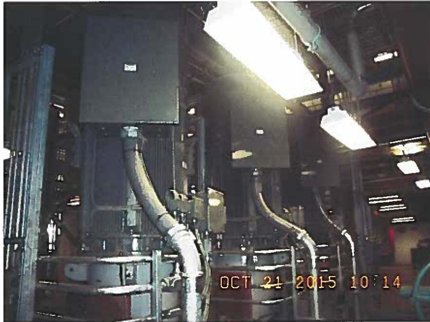
Condensate Pumps at Cane Run Unit 7
