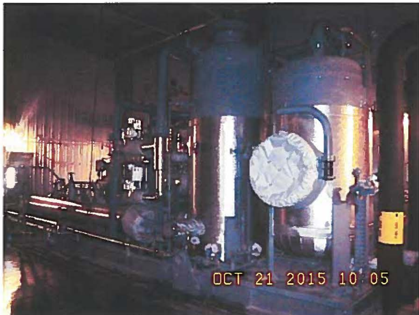
Gas Compressors at Cane Run Unit 7 Generating Station
