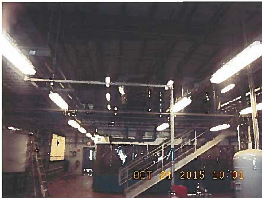
Filter Press (2) at Cane Run Unit 7
