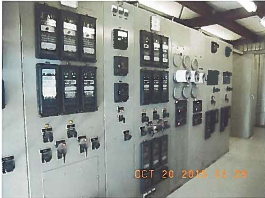
Relays at Toyota North Substation
