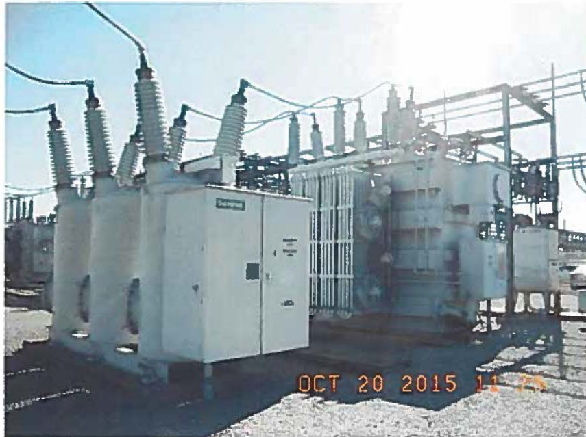
Oil Breakers and Transformer at Toyota North Substation
