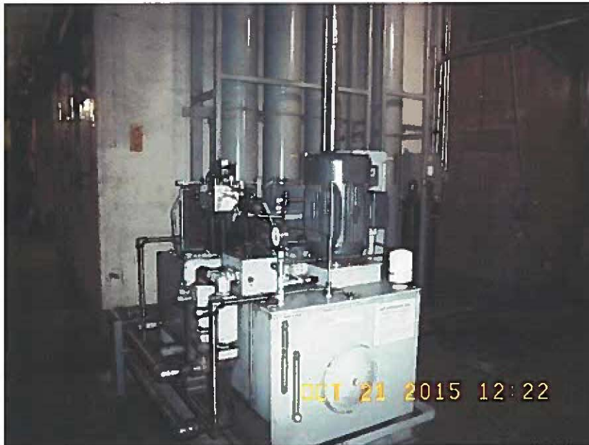
Unit 7 Governor System at Ohio Falls Hydro Plant
