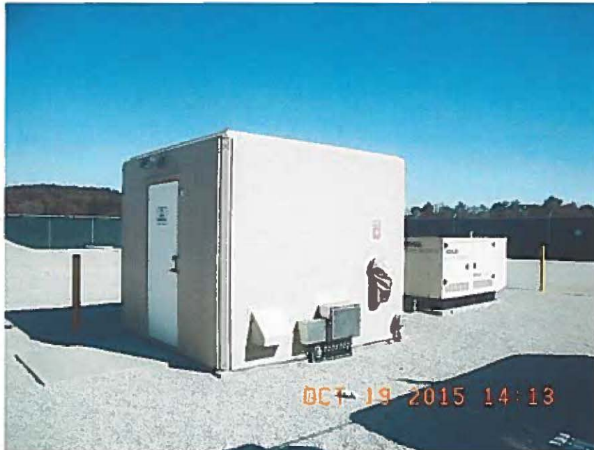
RTU Building and Kohler Generator at Cane Run City Gate Station
