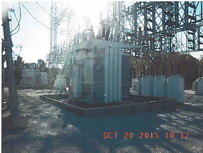
Oil Breakers and Transformers at Higby Mill Substation
