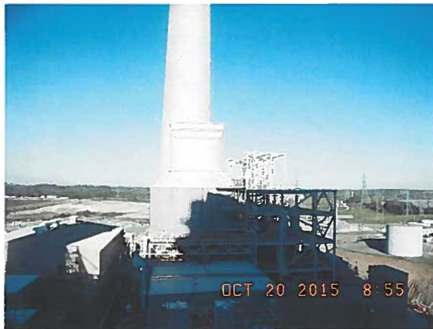
Scrubber at Brown Generating Station
