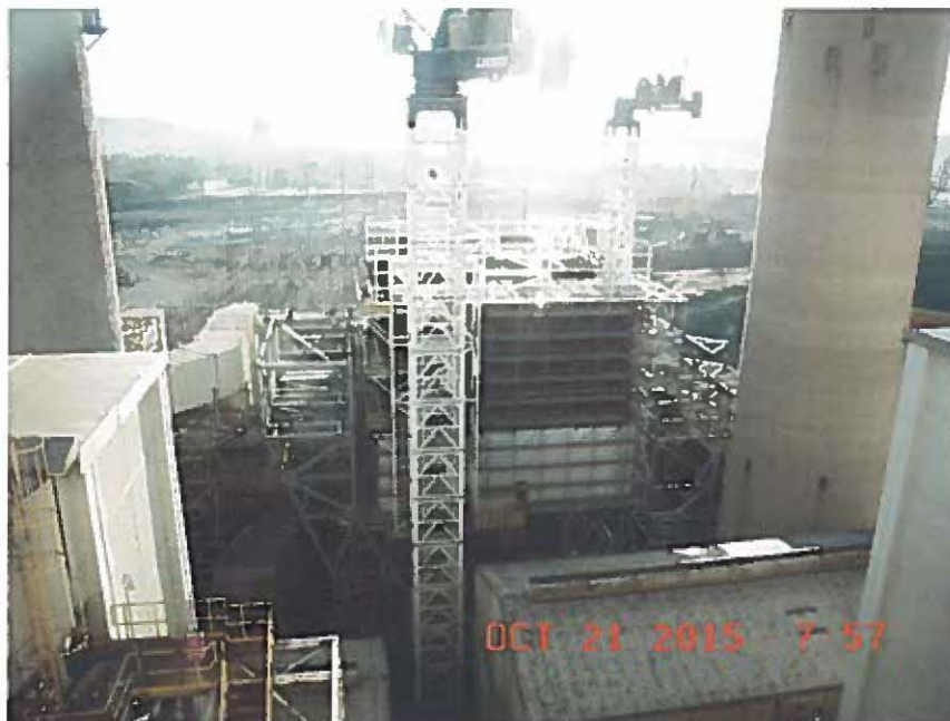
Unit 3 Baghouse at Mill Creek Generating Station
