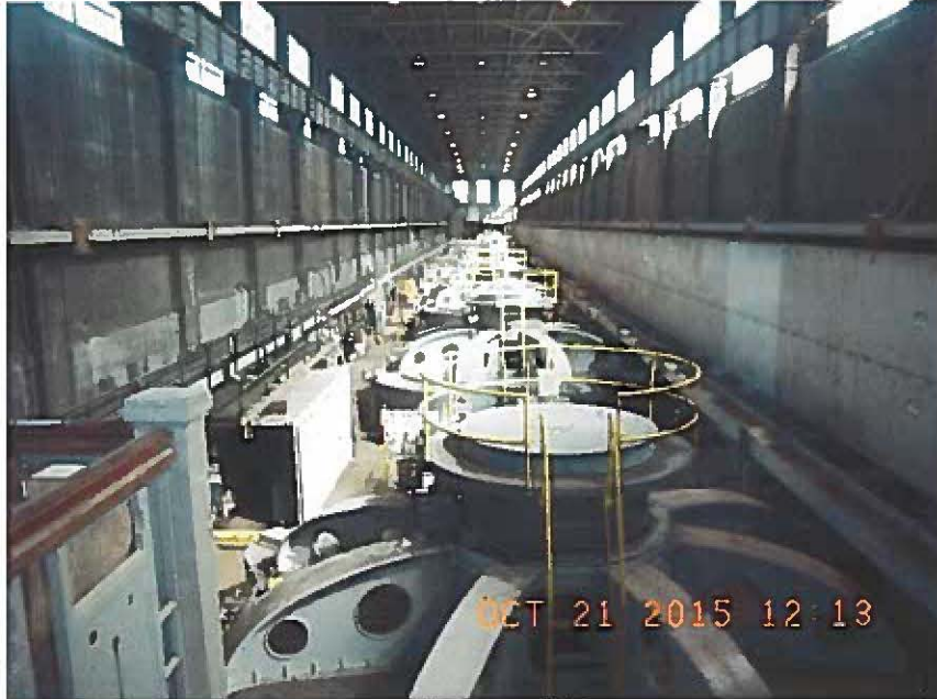
Generators at Ohio Falls Hydro Plant
