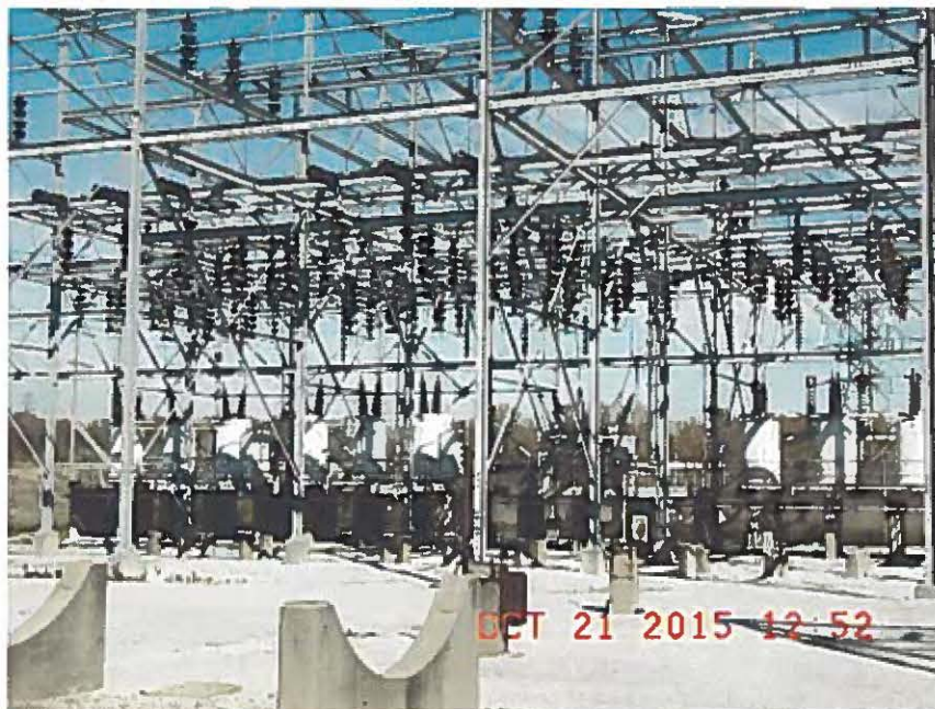
138KV Oil Breakers at Canal Substation
