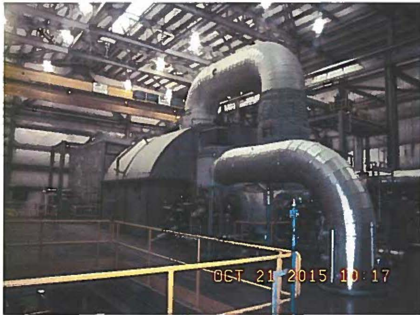
Steam Turbine at Cane Run Unit 7 Generating Station
