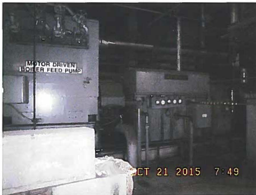
Boiler Feed Pump at Mill Creek Generating Station
