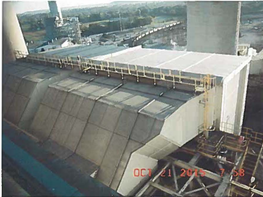
Unit 2 SCR at Mill Creek Generating Station
