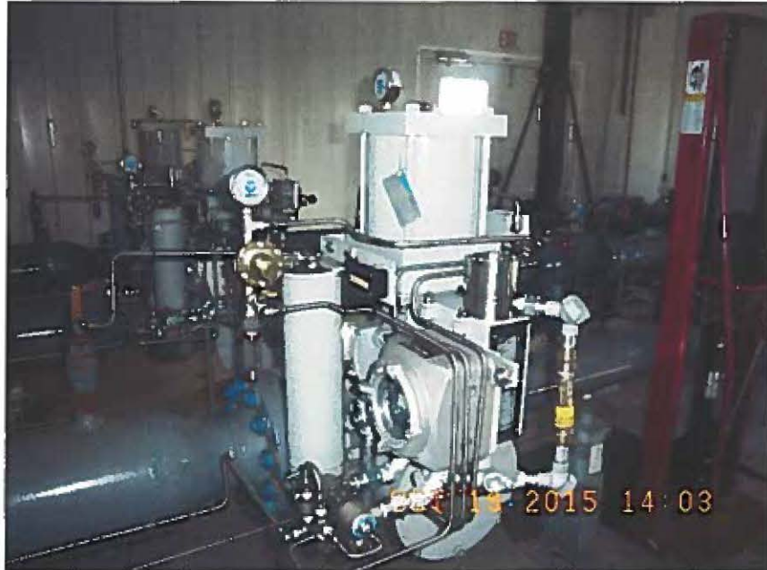
Regulator Runs at Penile City Gate Station
