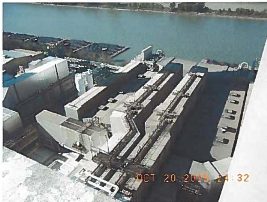
Unit 4 Precipitator at Ghent Generating Station
