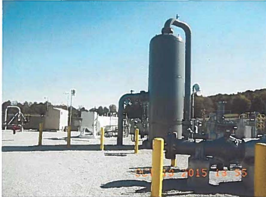
Separator and Odorant at Penile City Gate Station
