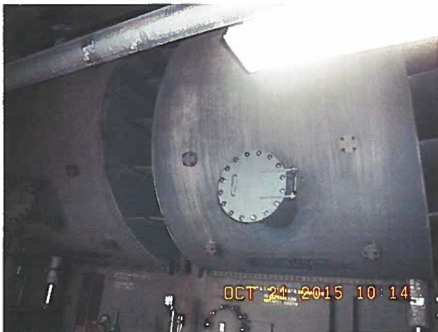
Condenser at Cane Run Unit 7
