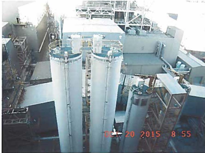
Carbon and Lime Silos at Brown Generating Station
