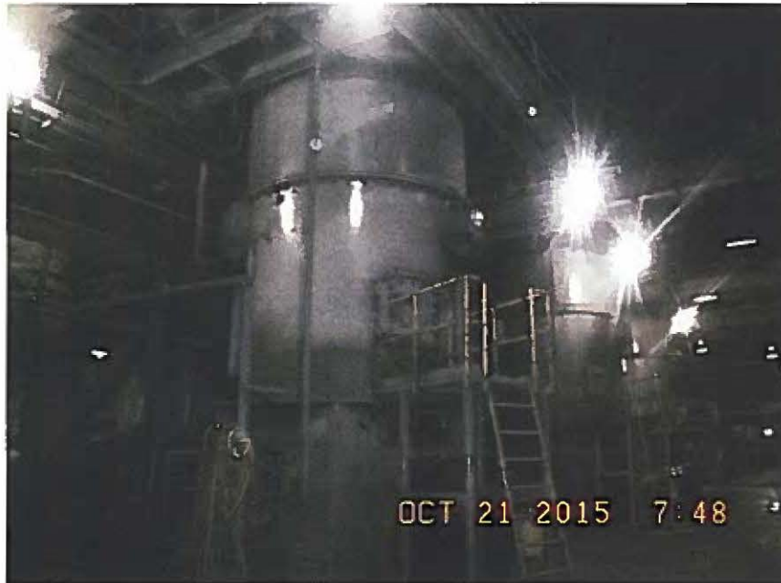
Unit 3 Pulverizers at Mill Creek Generating Station
