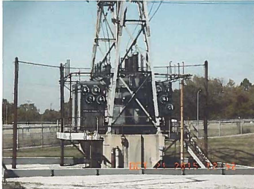
Transformer at Canal Substation
