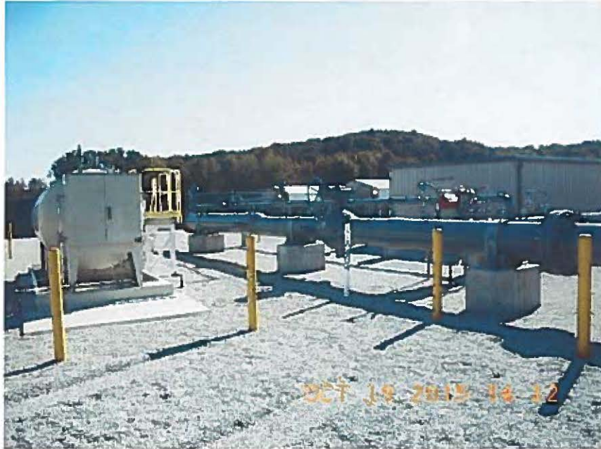
Odorant Tank and Piping at Cane Run City Gate Station
