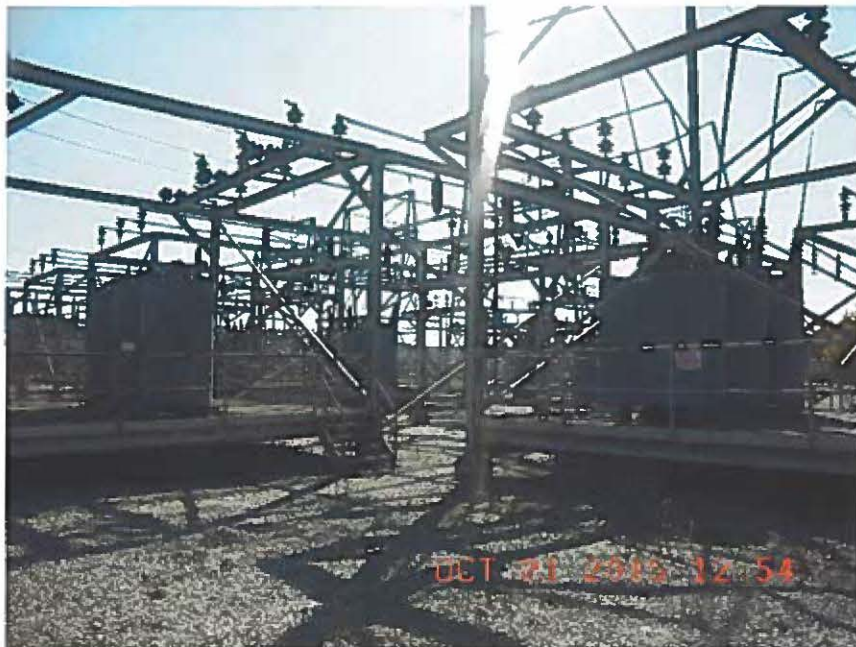
69KV Oil Breakers at Canal Substation
