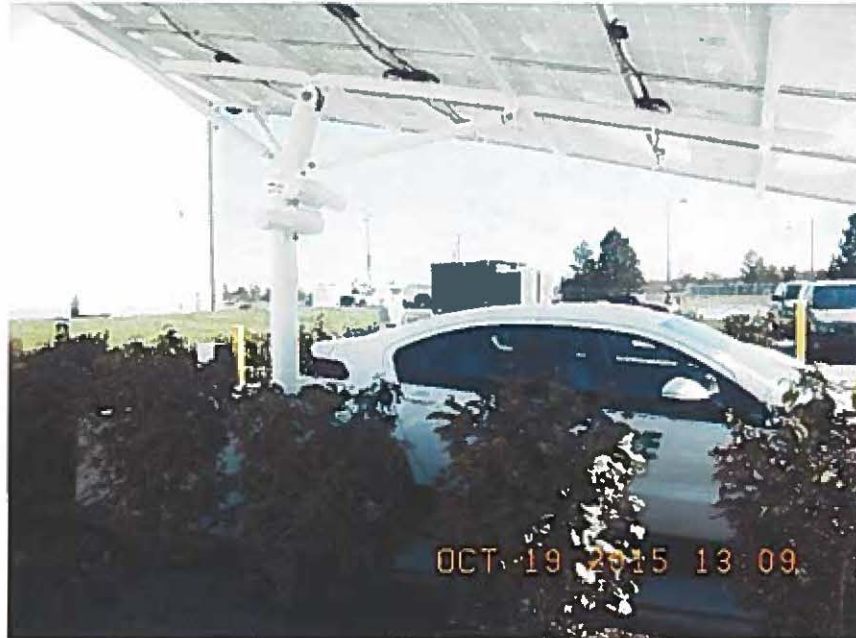
EU Charging Station at Auburndale Service Center
