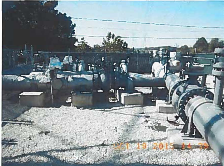
Regulator at Blanton Lane Regulator Station
