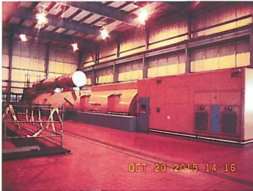
Unit 3 Turbine at Ghent Generating Station
