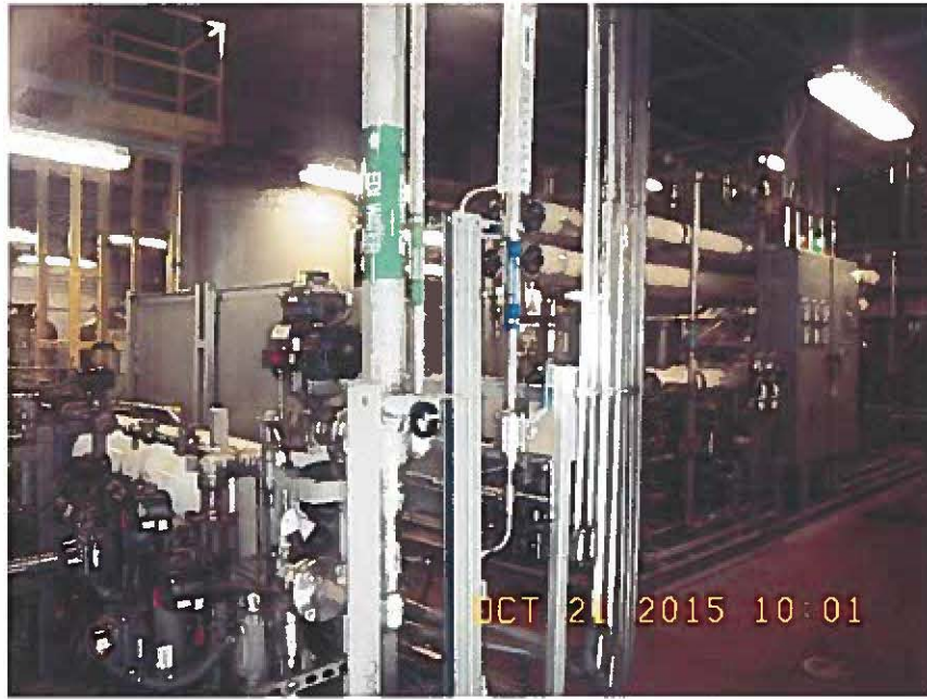
Reverse Osmosis at Cane Run Unit 7
