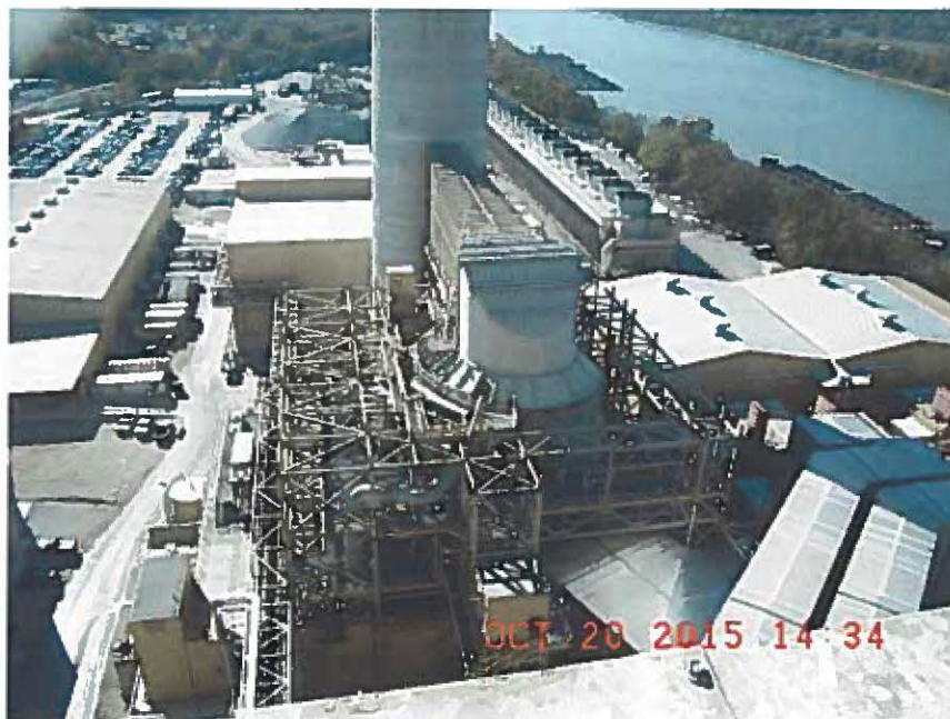
Unit 4 Scrubber at Ghent Generating Station
