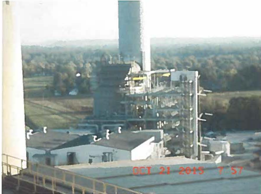
Unit 1 Scrubber at Mill Creek Generating Station
