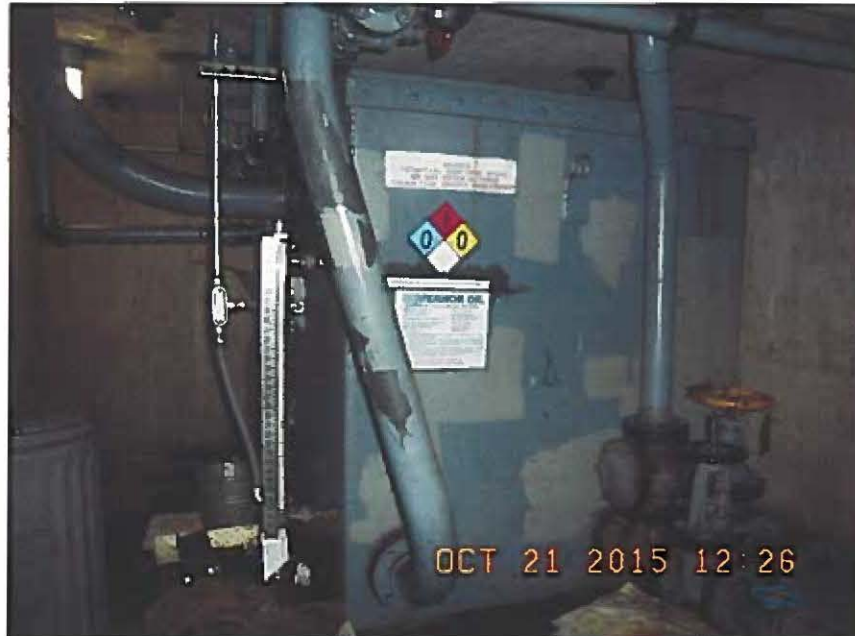
Oil Tank and Pump at Ohio Falls Hydro Plant
