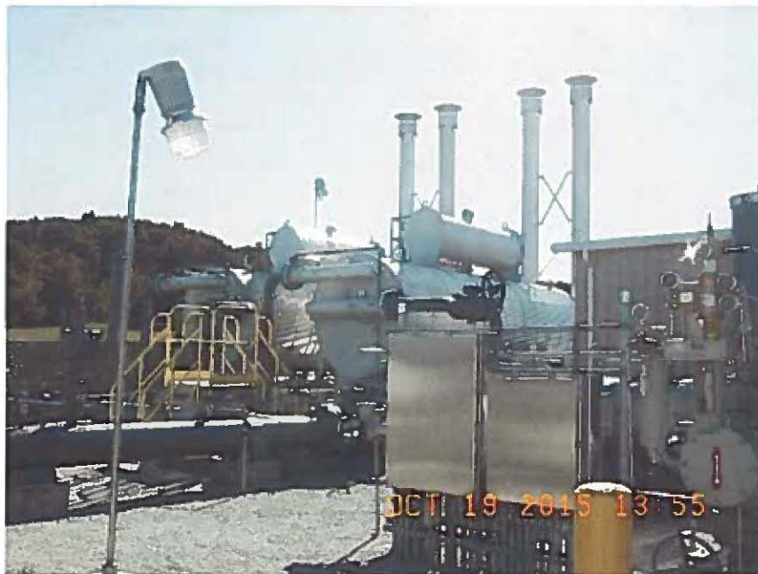
Heaters at Penile City Gate Station
