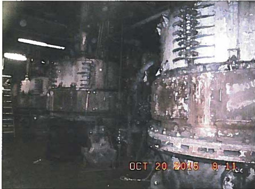
Unit 1 Pulverizers at Brown Generating Station
