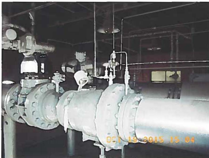
Regulator Runs at St. Helens Regulator Station
