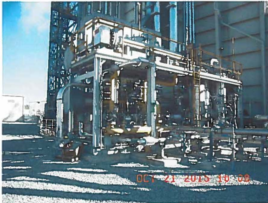
Heat Exchangers at Cane Run Unit 7 Generating Station
