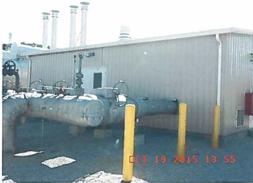
Regulator Building at Penile City Gate Station
