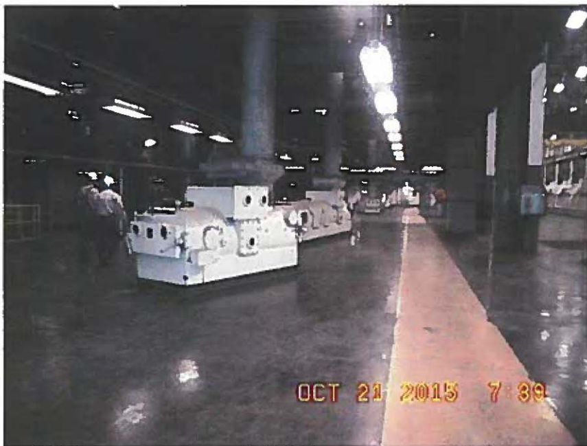
Coal Feeders at Mill Creek Generating Station
