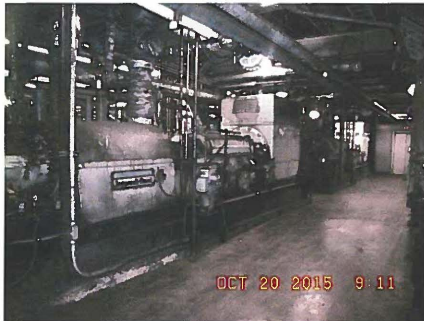
Boiler Feed Pumps at Brown Generating Station
