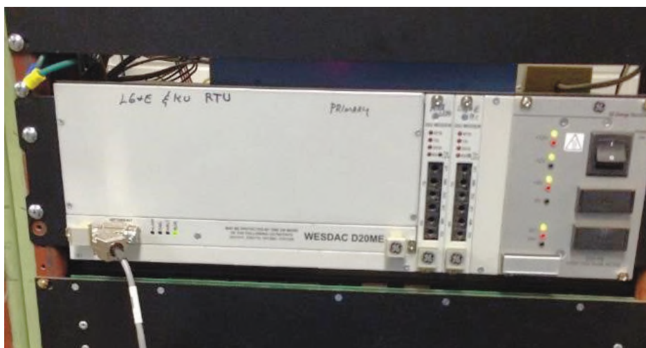
Figure 31: GE D20 remote terminal unit.
