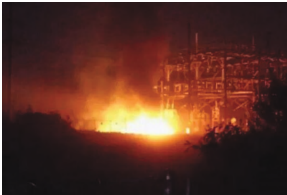
Figure 35: 69kV circuit breaker failure.
