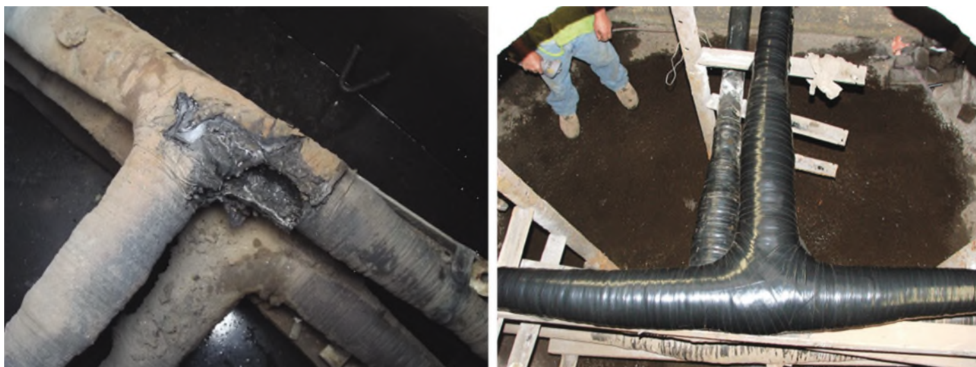
Figure 37: Example of a failed underground transmission splice.
