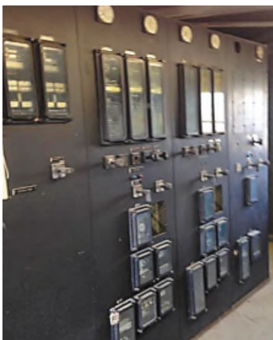
Figure 29: Electro-mechanical relay panels.
