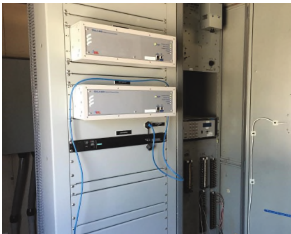
Figure 33: Tesla digital fault recorder.
