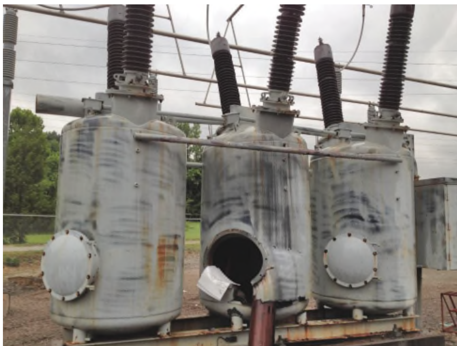
Figure 14: Example of a failed circuit breaker with oil release.
