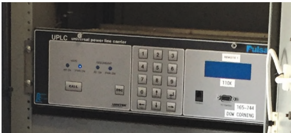
Figure 32: Power line carrier set.
