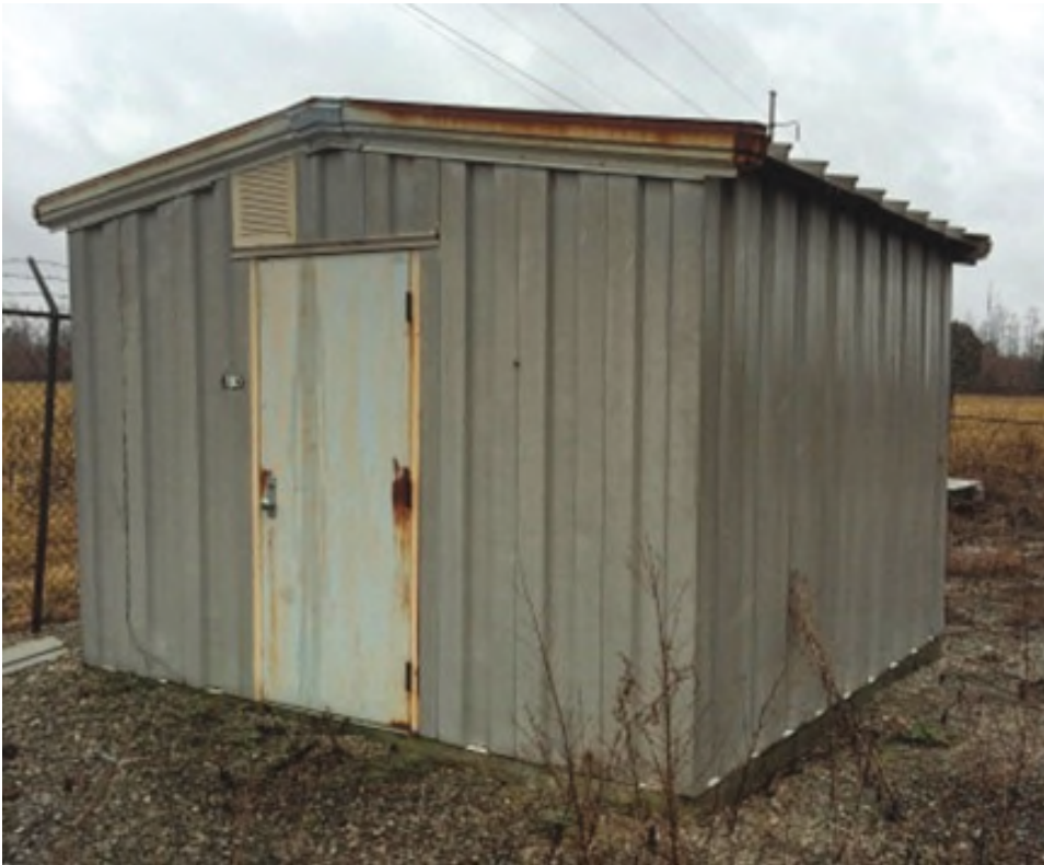
Figure 28: Example of an old control house that needs to be replaced.
