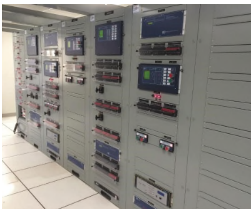
Figure 30: Microprocessor relay panels.
