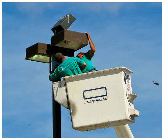
Figure 2-2. Replacement of lamps typically requires the use of a bucket truck, which can be costly
