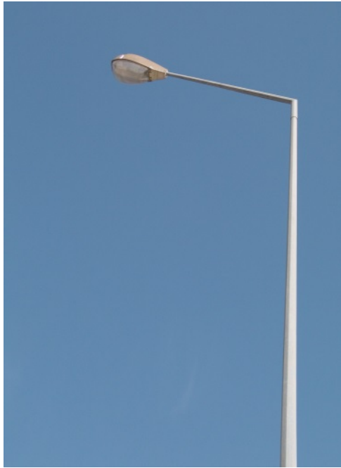
Figure 1-4. Example of a cobrahead-style street light
