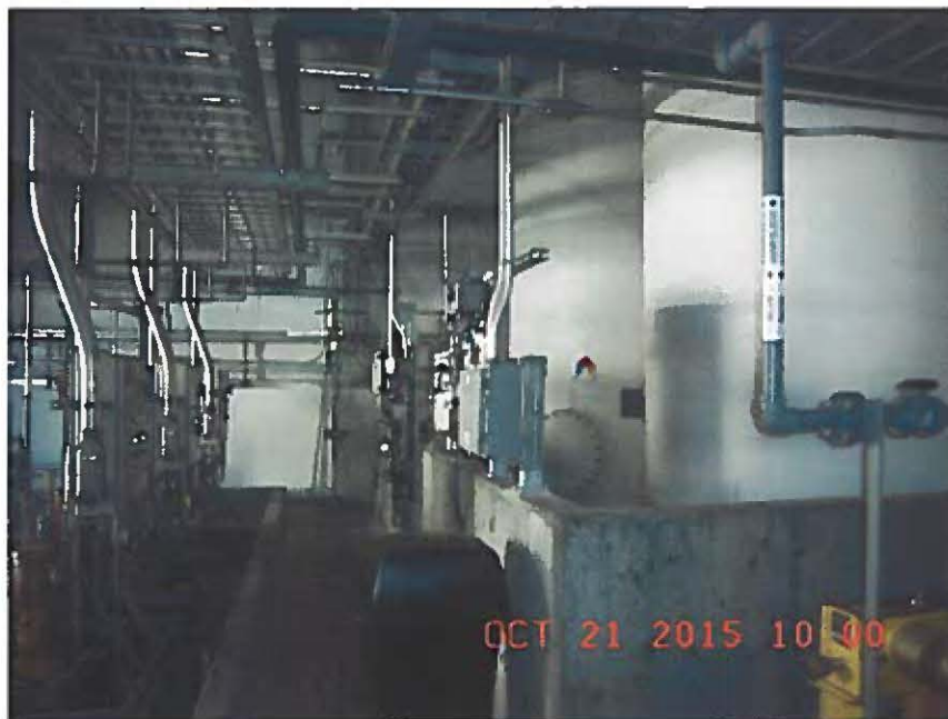
Chemical Treatment at Cane Run Unit 7
