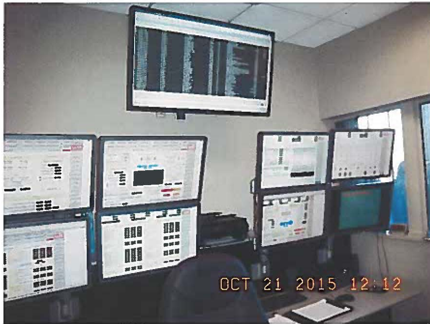
Control Room at Ohio Falls Hydro Plant
