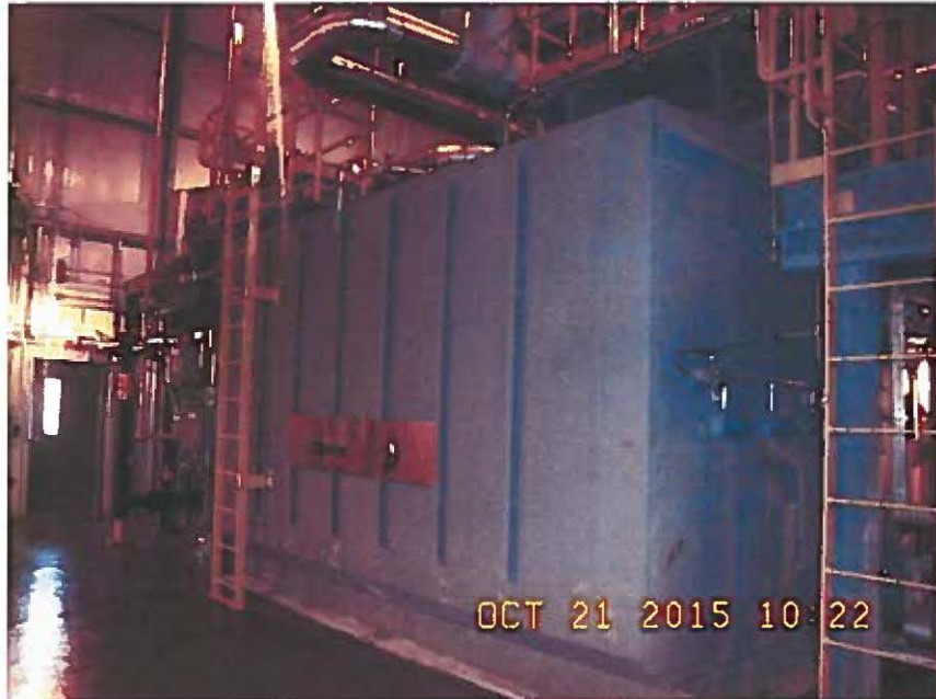
Auxiliary Boiler at Cane Run Unit 7 Generating Station
