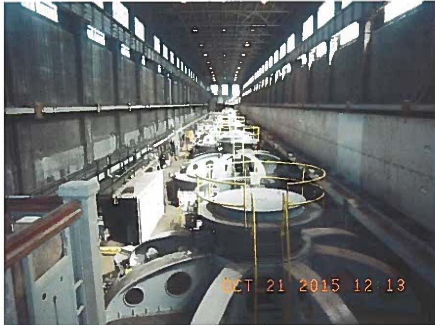
Generators at Ohio Falls Hydro Plant
