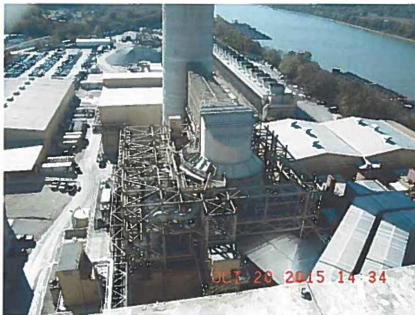
Unit 4 Scrubber at Ghent Generating Station
