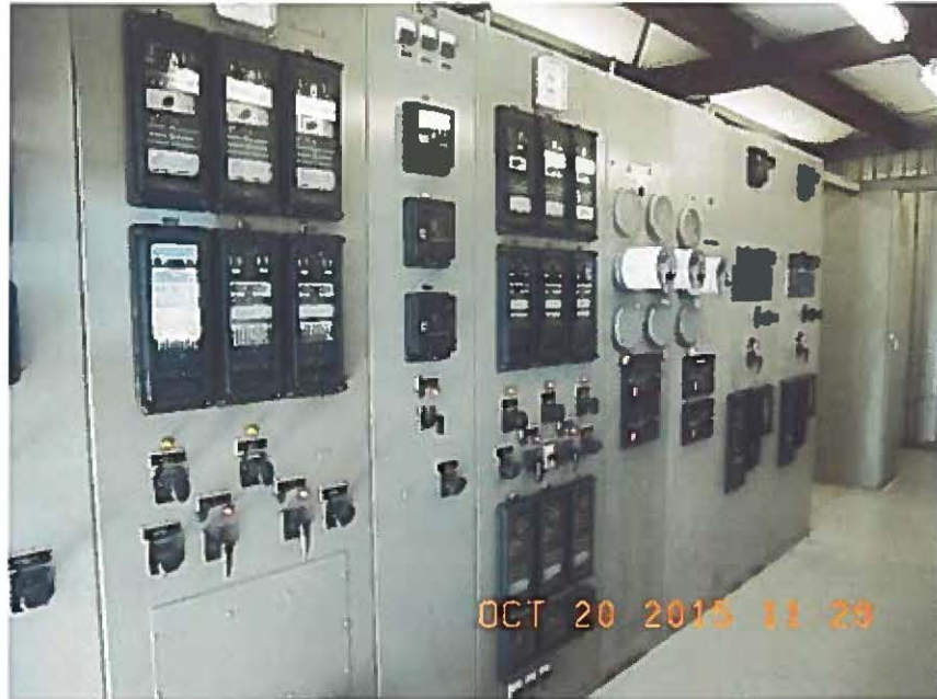
Relays at Toyota North Substation
