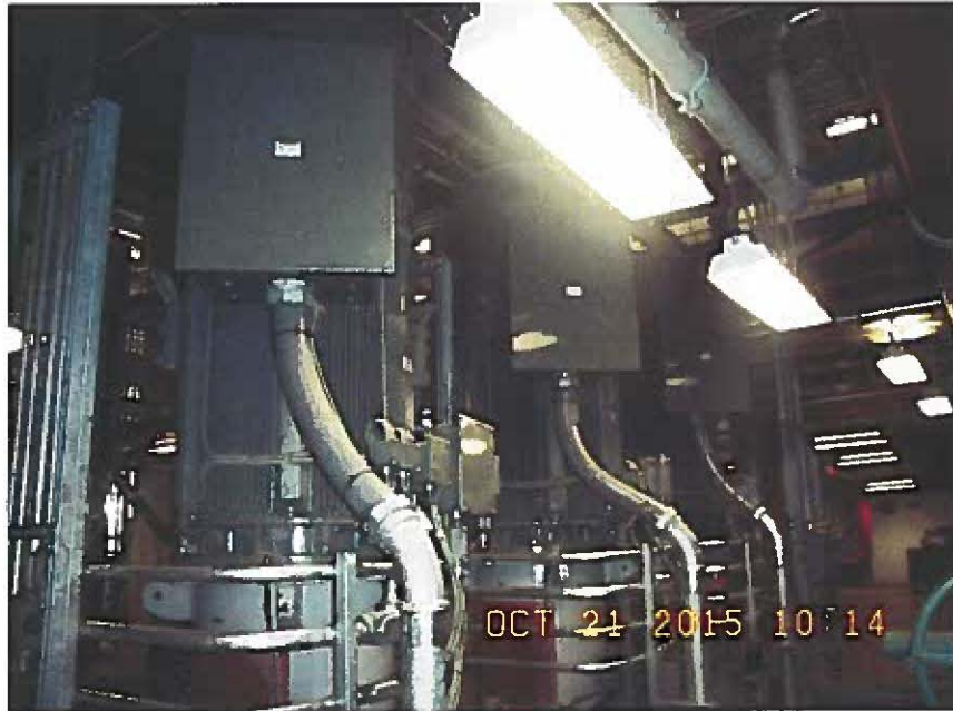
Condensate Pumps at Cane Run Unit 7
