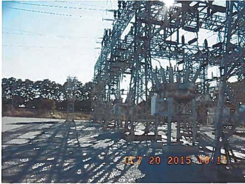
Capacitor Bank and SF 6 Breakers at Higby Mill Substation
