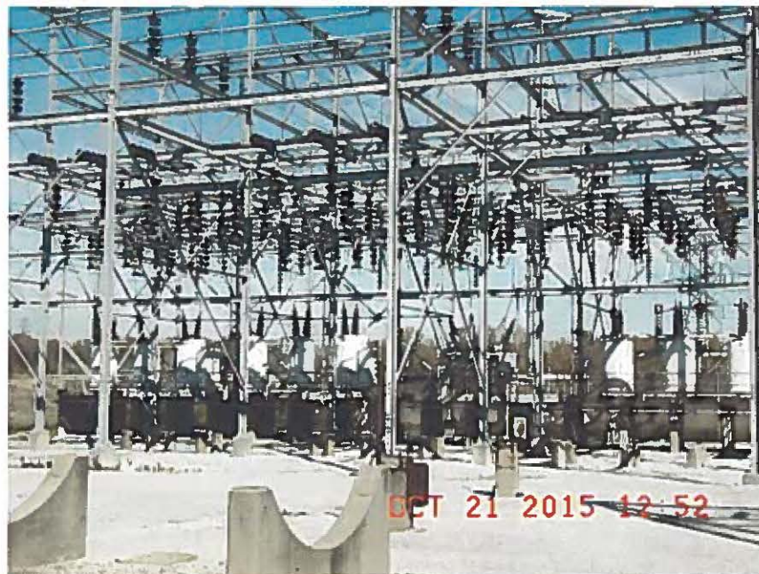
138KV Oil Breakers at Canal Substation
