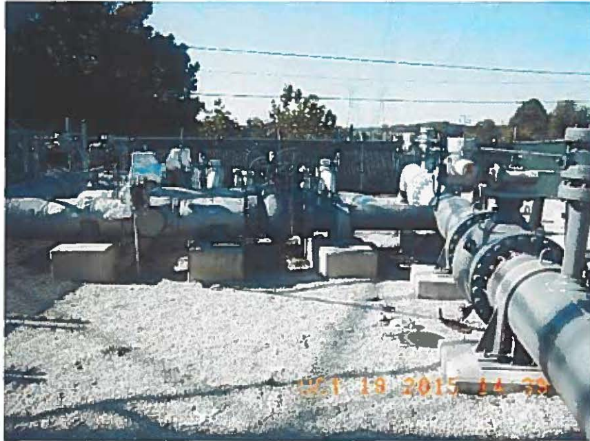
Regulator at Blanton Lane Regulator Station
