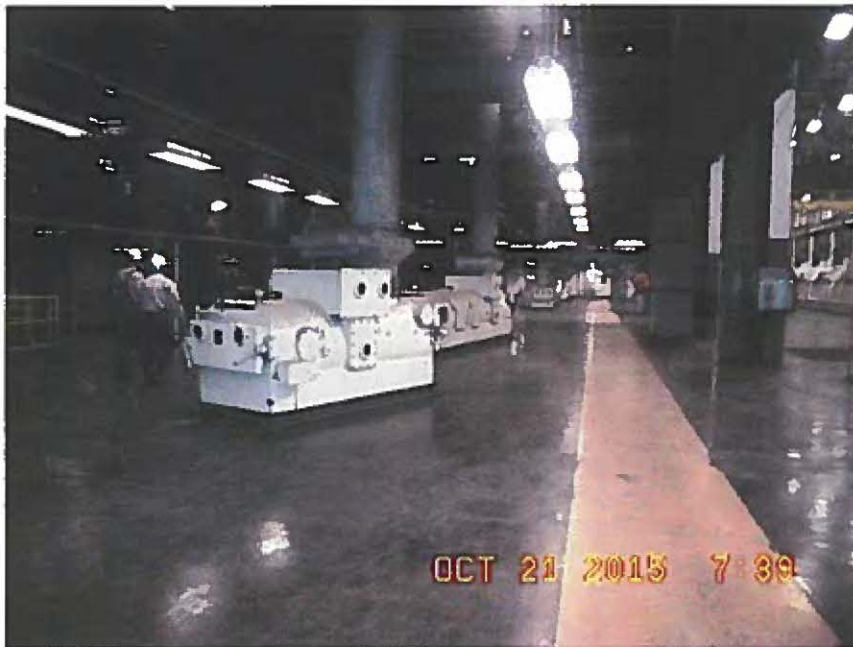
Coal Feeders at Mill Creek Generating Station
