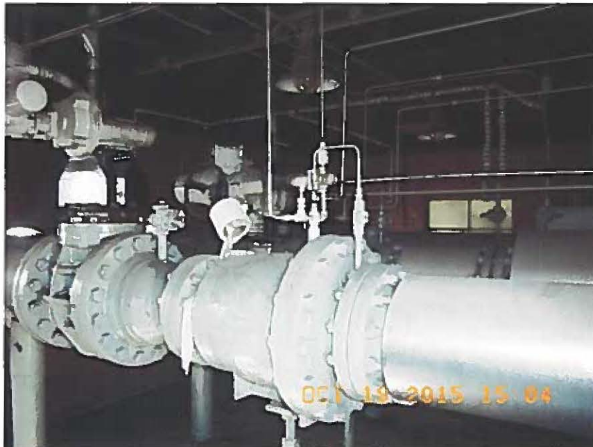
Regulator Runs at St. Helens Regulator Station
