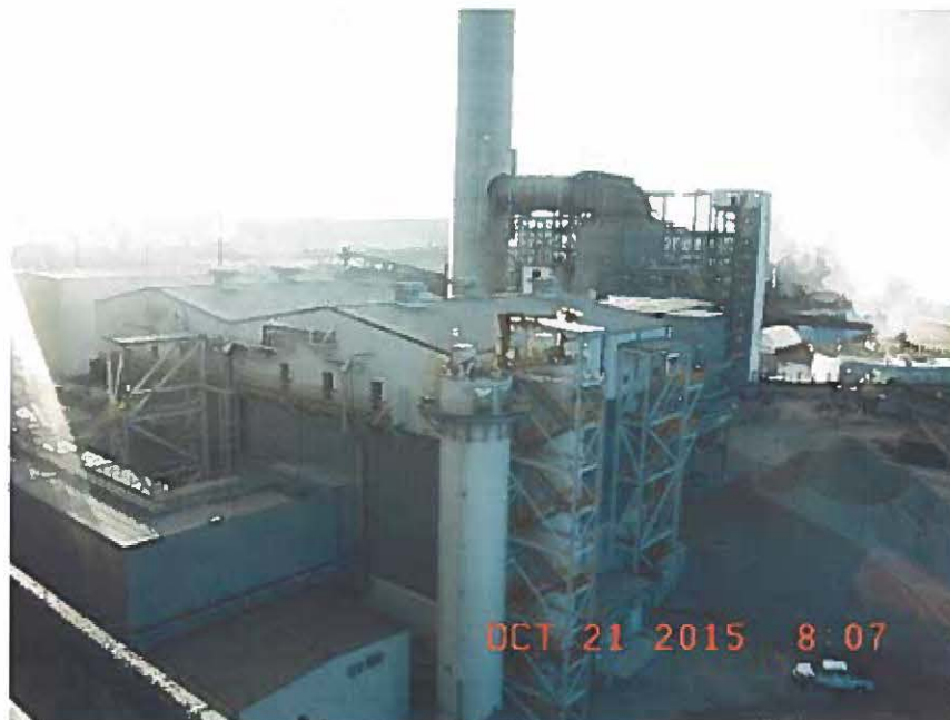
Unit 4 Scrubber at Mill Creek Generating Station
