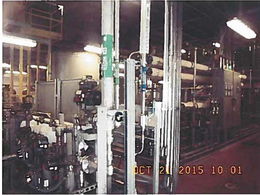
Reverse Osmosis at Cane Run Unit 7
