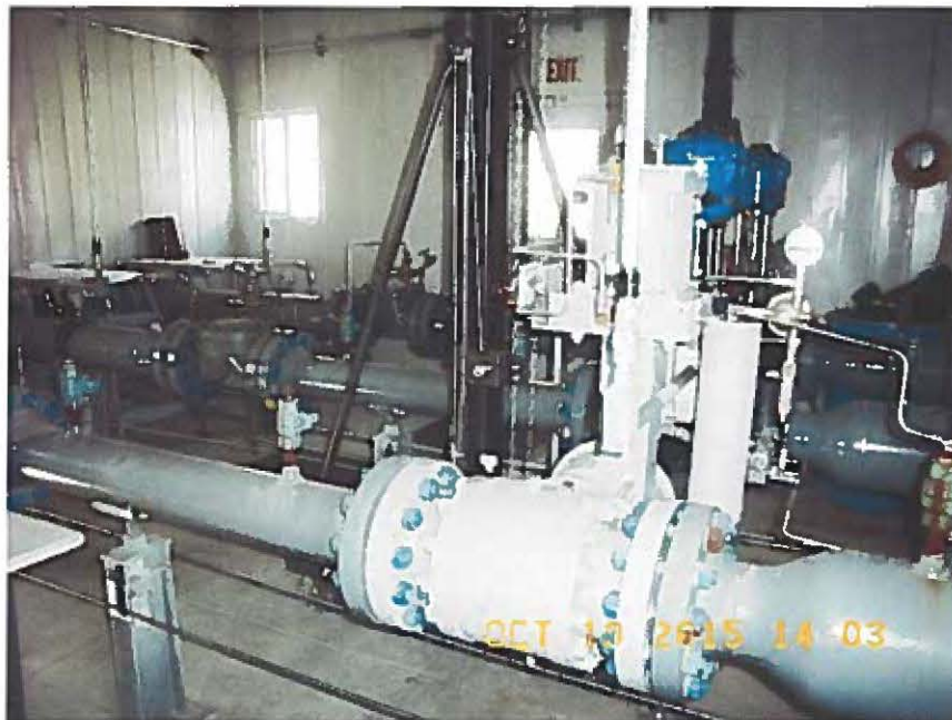
Regulator Runs at Penile City Gate Station
