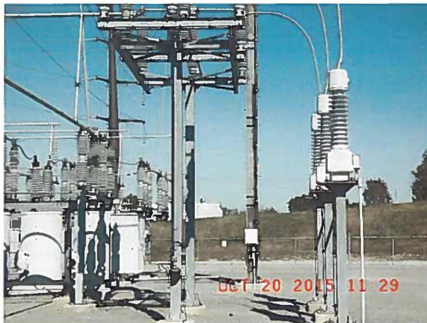
Potential Transformers at Toyota North Substation
