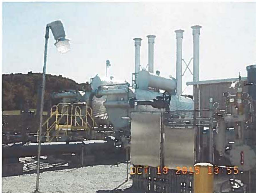
Heaters at Penile City Gate Station
