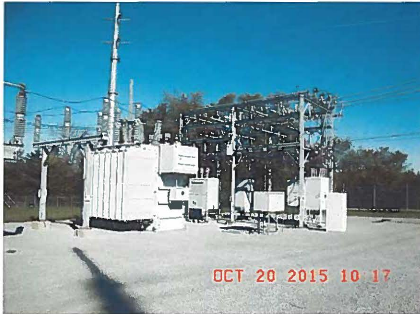
Transformer and Vacuum Breakers at Higby Mill Substation
