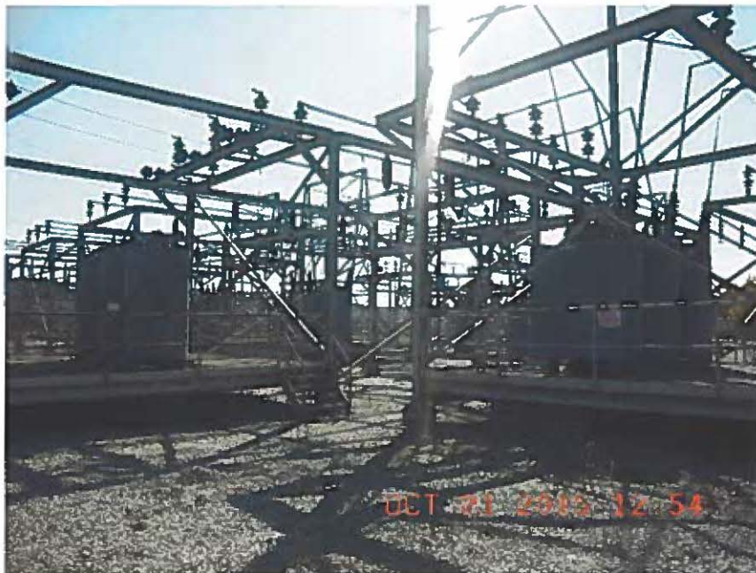
69KV Oil Breakers at Canal Substation
