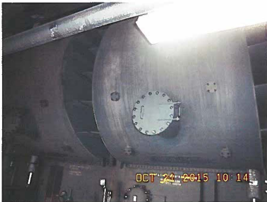
Condenser at Cane Run Unit 7
