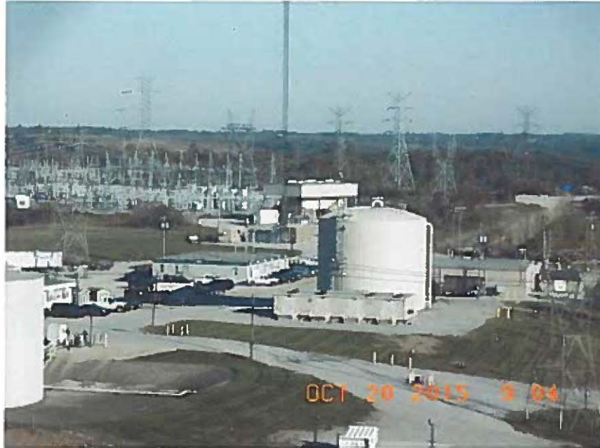
Ammonia and Water System at Brown Generating Station
