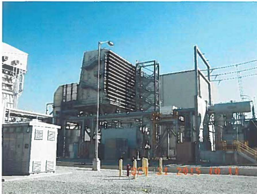
Air Inlet at Cane Run Unit 7 Generating Station
