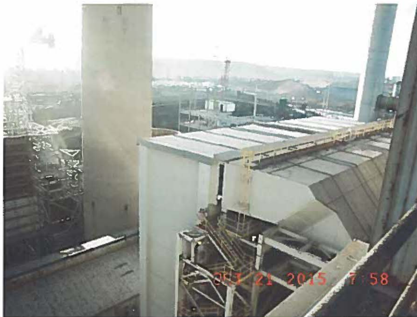
Unit 3 SCR at Mill Creek Generating Station
