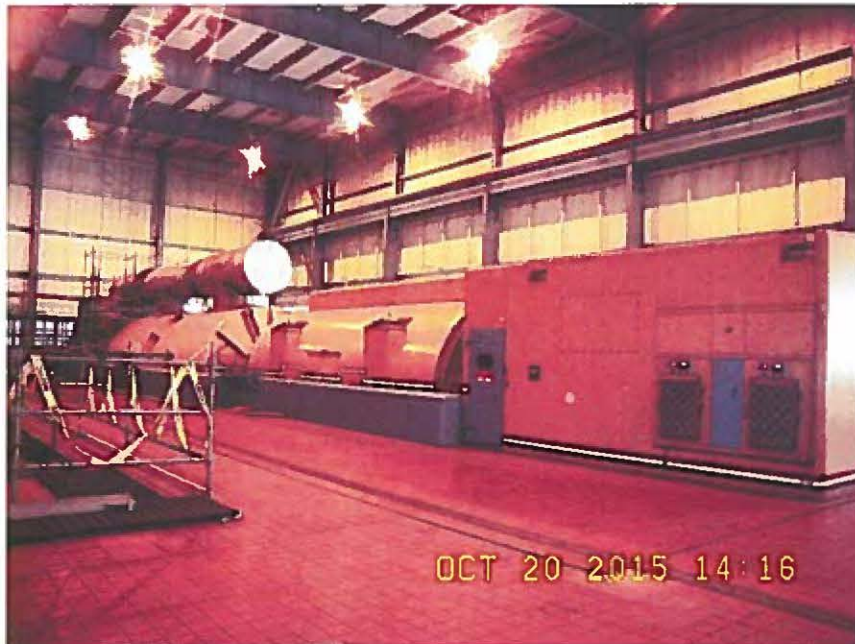
Unit 3 Turbine at Ghent Generating Station
