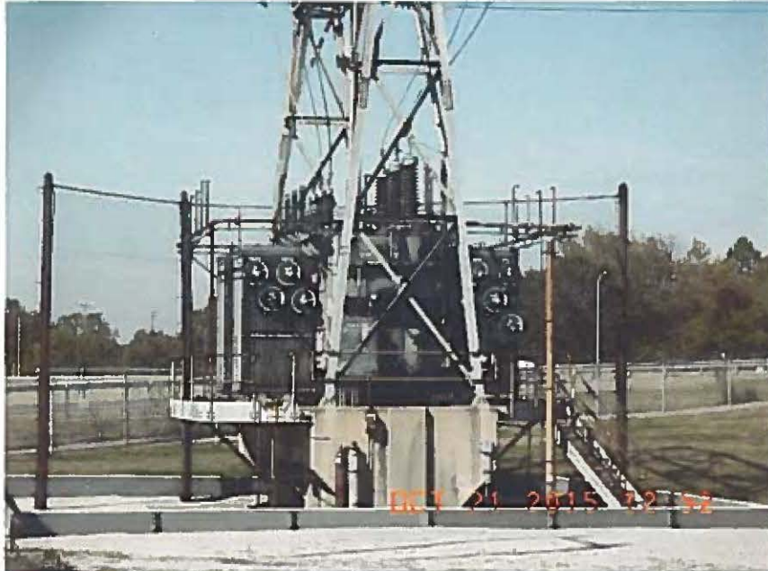
Transformer at Canal Substation
