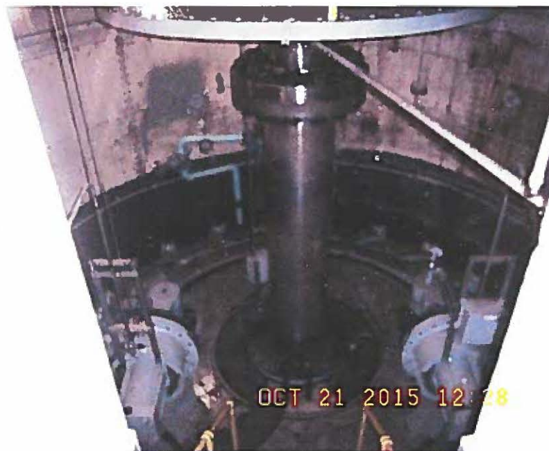
Unit 1 Turbine Shaft at Ohio Falls Hydro Plant
