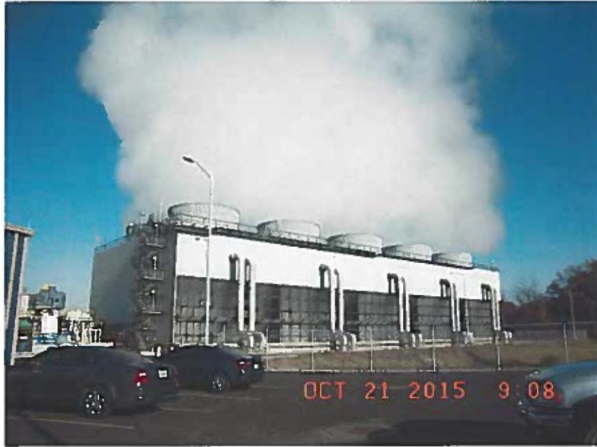
Cooling Tower at Cane Run Unit 7 Generating Station
