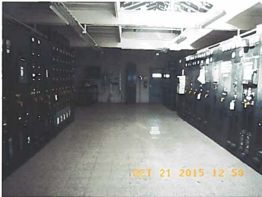
Relays at Canal Substation
