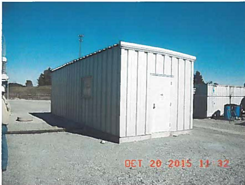
Control Building at Toyota North Substation
