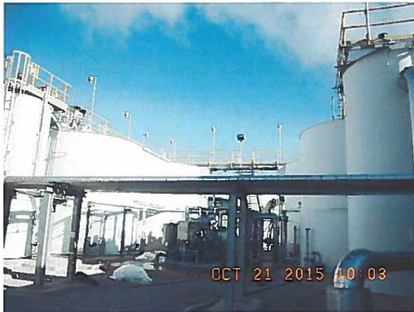
Water Clarifiers at Cane Run Unit 7
