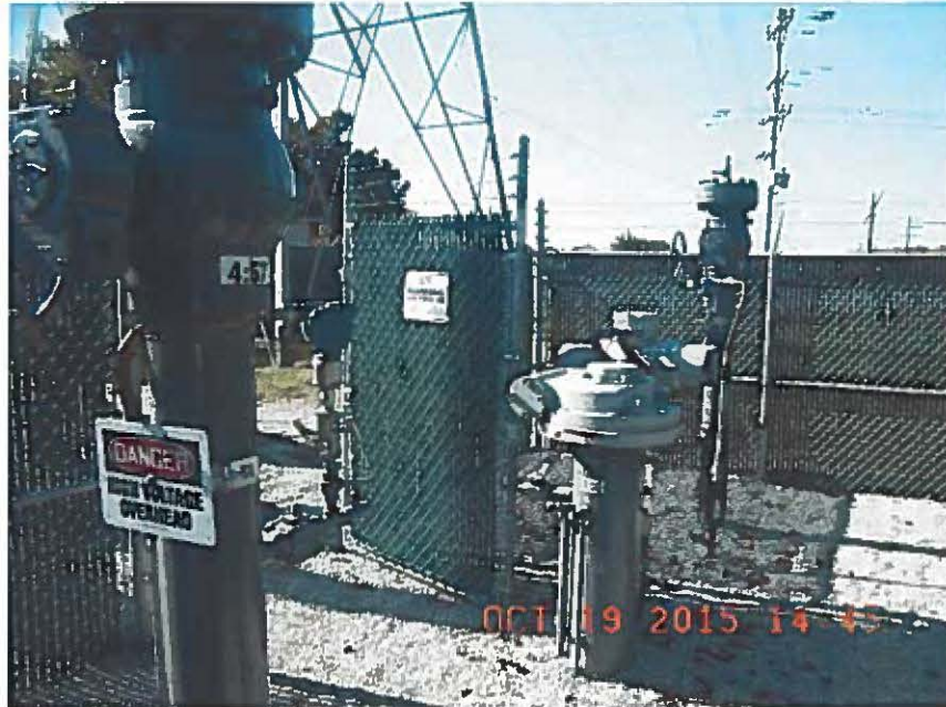
(Electric) Cane Run 7 Regulator and Valve Next to Blanton Lane Station
