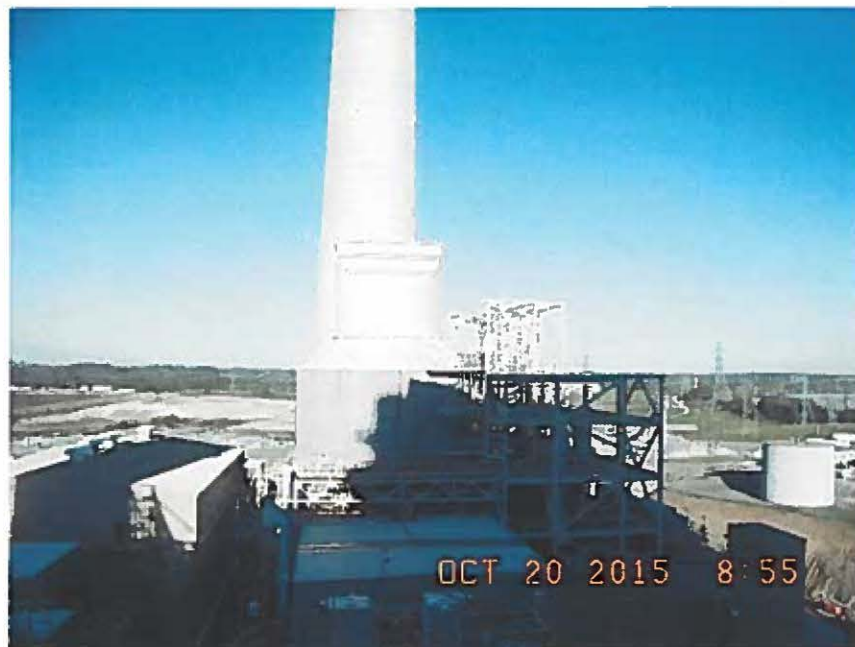
Scrubber at Brown Generating Station
