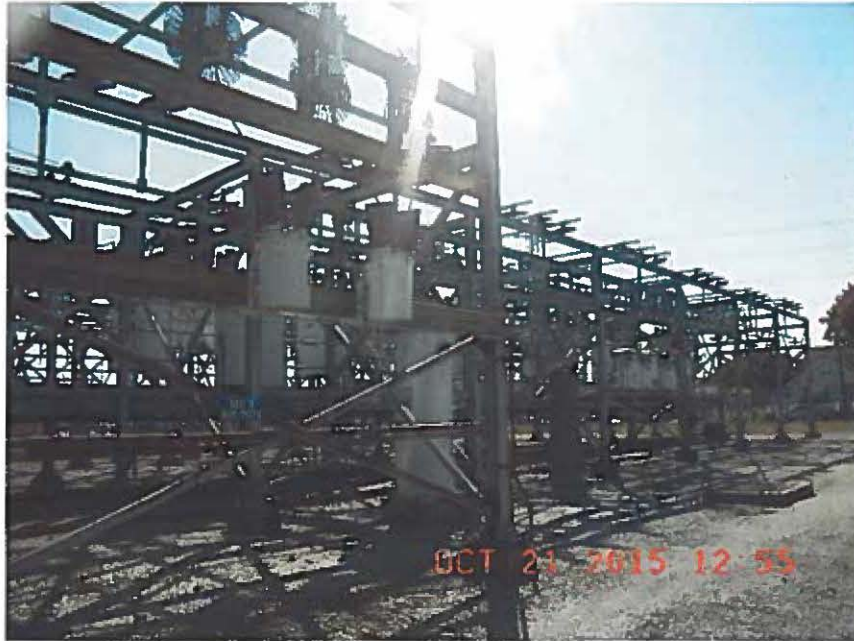
14KV Breakers at Canal Substation
