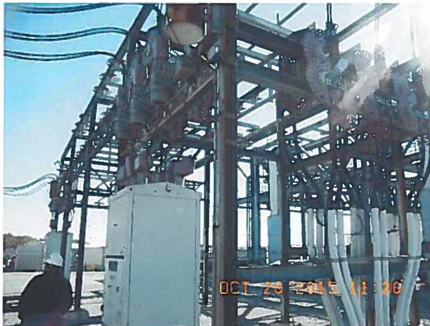
Vacuum Breakers at Toyota North Substation
