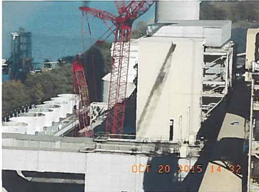
Unit 1 Scrubber at Ghent Generating Scrubber
