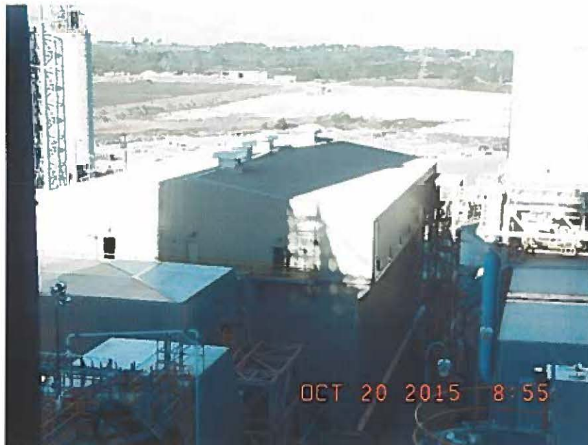
Baghouse at Brown Generating Station
