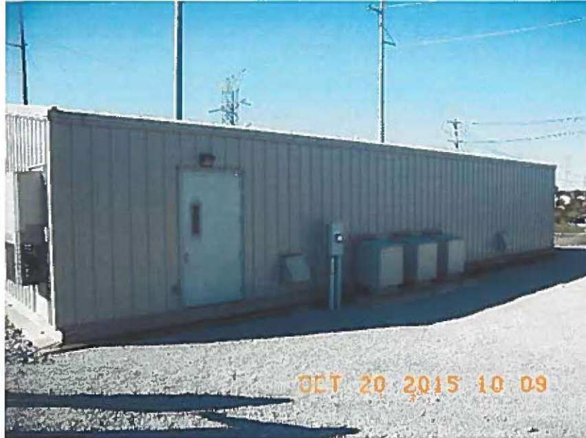
Control Building at Higby Mill Substation
