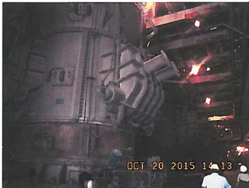
Pulverizers Unit 4 at Ghent Generating Station
