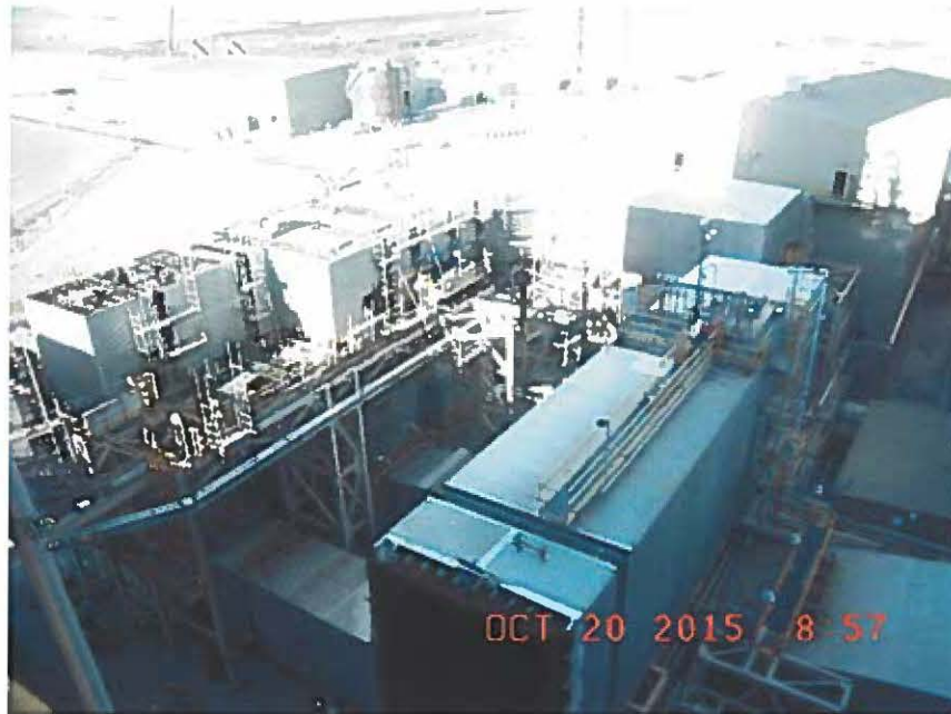
Air Exhaust/ID Fan at Brown Generating Station
