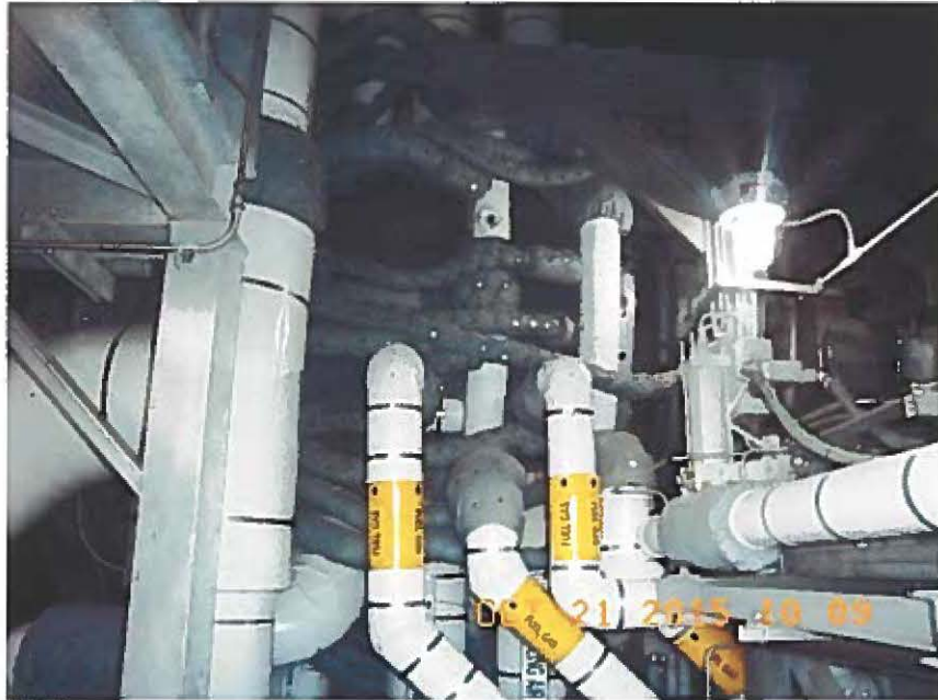
Gas Turbine at Cane Run Unit 7
