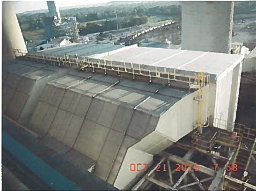
Unit 2 SCR at Mill Creek Generating Station
