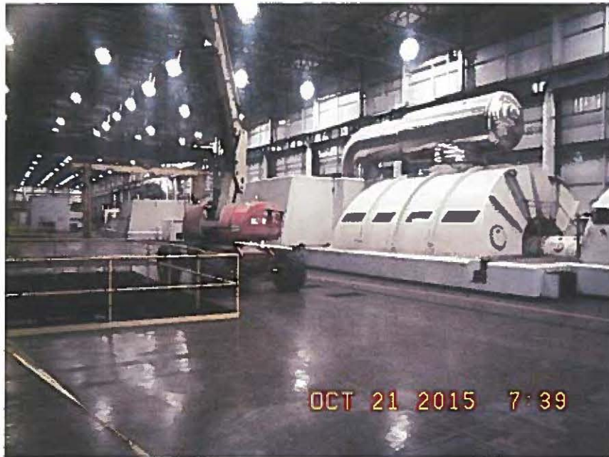
Units 1 & 2 Turbines at Mill Creek Generating Station
