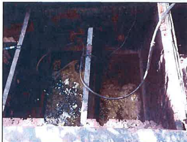
Chlorine contact chamber
