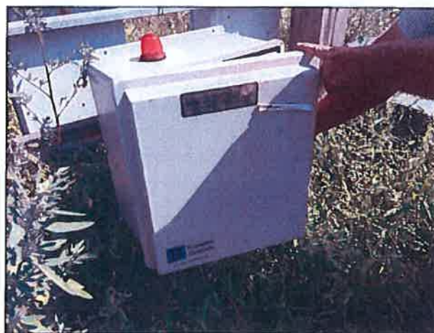
Control panel without lock
