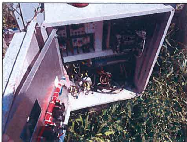
Inside control panel
