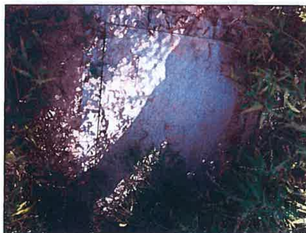
Lift station lid without lock
