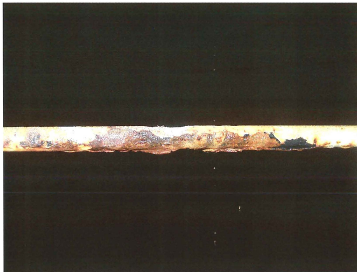
Photo shows the second ladder rung that is also severely deteriorated and should be replaced. The cross section of the rung has been reduced by corrosion.
