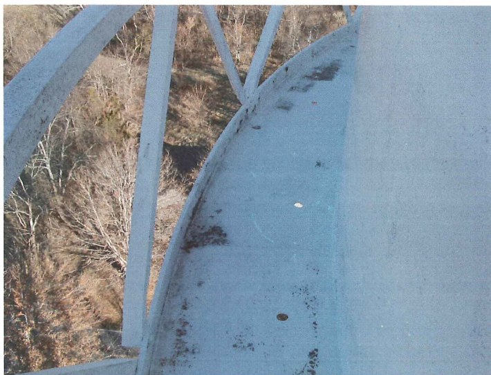
Photo shows scattered corrosion cells on the northwest section of the balcony.
