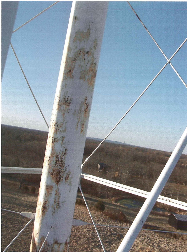
Photo shows the upper panel section of the 36" diameter riser pipe. The brittle coating is delaminating to the steel substrate.
