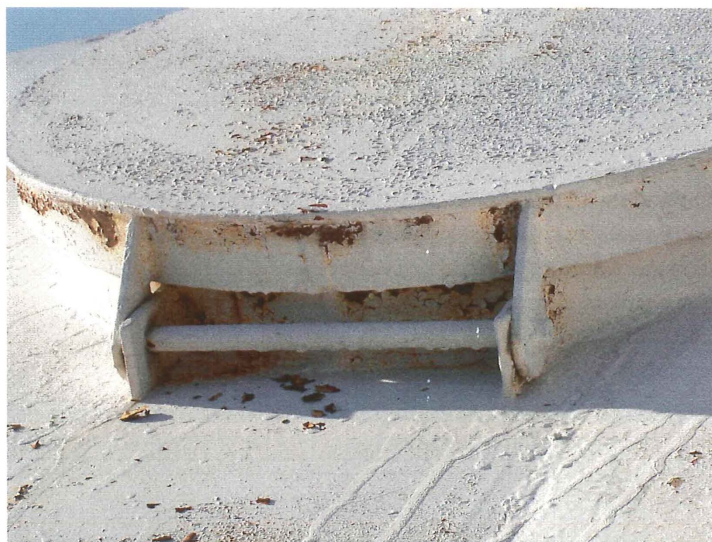
Photo shows the roof access hatches hinge. The hinge is structurally sound. The hatch opens and closes properly.
