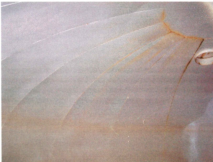
Photo shows the east section of the upper knuckle and the roof finger panels. The white epoxy coating is stained but continues to protect the steel substrate.
