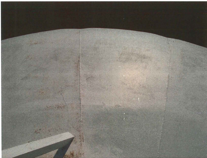
Photo shows the east section of the roof. The brittle coating exhibits poor intercoat cohesion.
