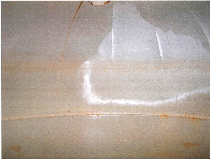
Photo shows the south section of the upper knuckle. Minor rust is visible along the painter's ring located at the top of the shell.
