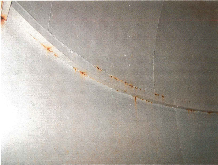
Photo shows the northeast upper shell and the painter's ring. Crevice corrosion is active.
