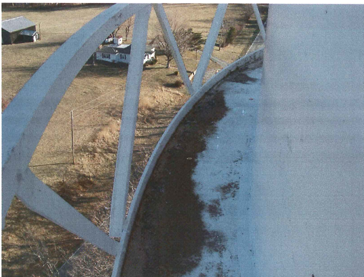
Photo shows total coating failure on the north section of the balcony. Additional drain holes need to be drilled.
