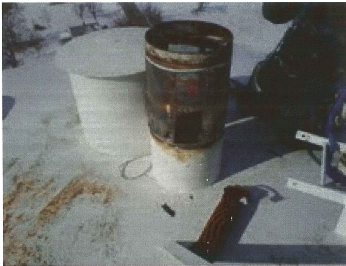
Photo shows the vent cover removed. The screen has been damaged. Insects can freely enter the tank. A new 24" diameter vent pipe should be installed.
