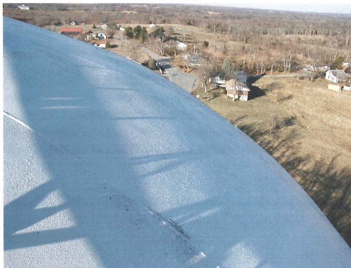
Photo shows the middle section of the north upper knuckle. The coating is brittle and has reached the end of its life cycle.
