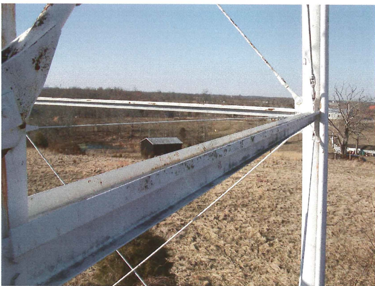
Photo shows the north lower strut. The strut is properly aligned. The protective coating is in poor condition.
