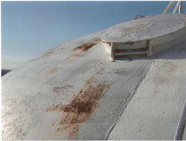
Photo shows an area of blotchy corrosion directly beneath the access hatch.
