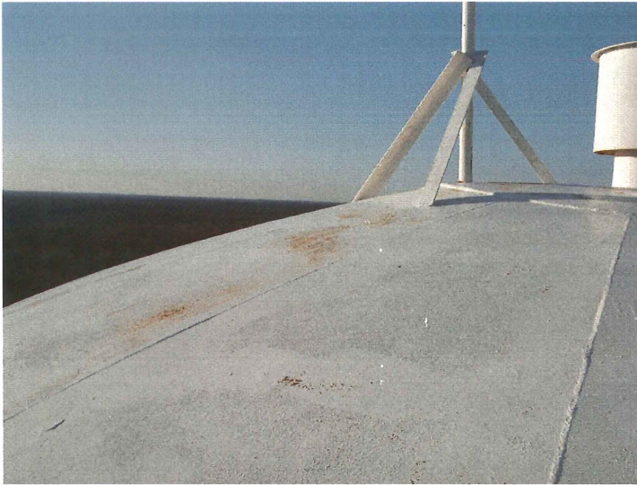
Photo shows the east roof finger panels. The white finish coat has started to fail.
