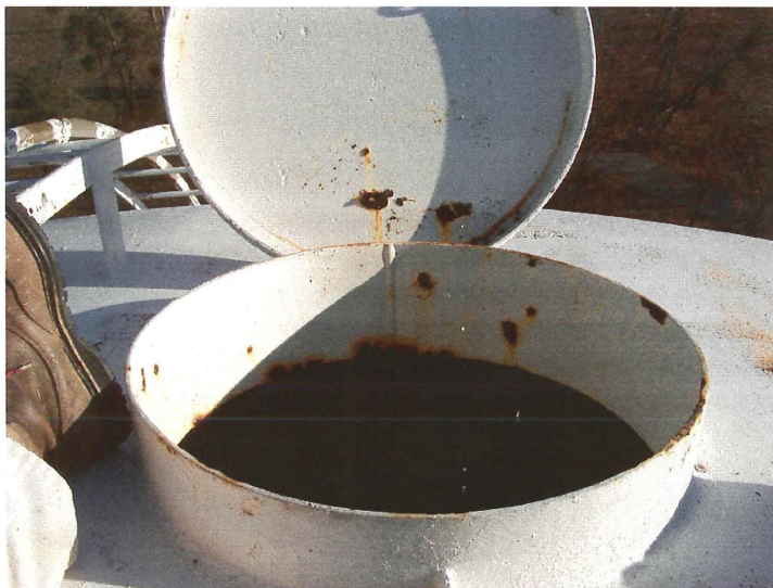
Photo shows the inside of the access hatch. Active corrosion cells are present on the frame. The interior ladder is not close to the hatch making access difficult.
