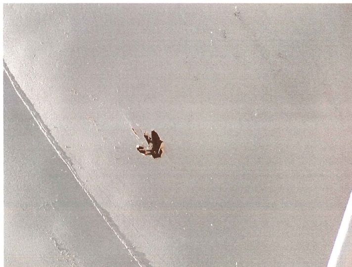
Photo shows a close-up of the delaminated spot on the east lower knuckle.
