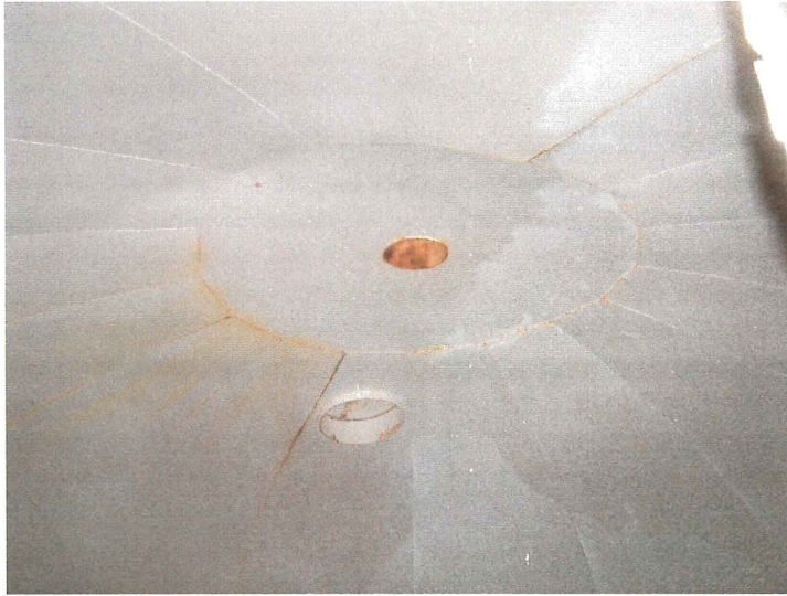
Photo shows an overall view of the roof. The 12" diameter roof vent is visible in the center of the roof cap plate. The 24" diameter secondary access hatch is also visible. Crevice corrosion is active along the lapped roof panel seams.
