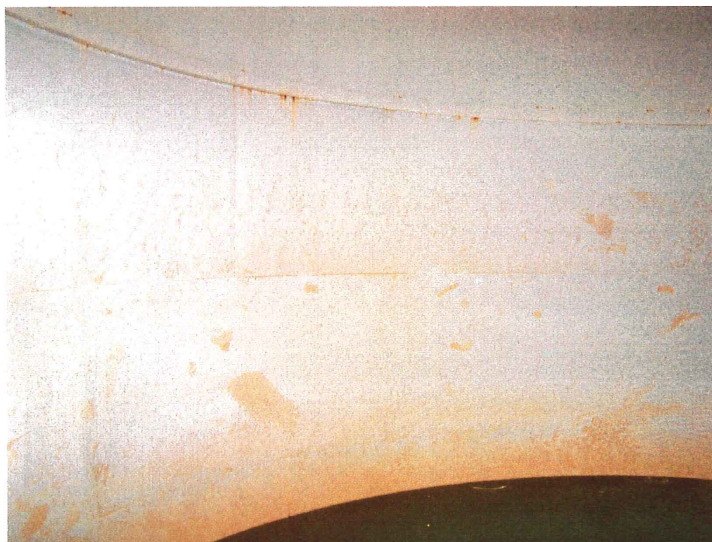
Photo shows the southeast section of the shell. The brown areas are stains. Rust creepage was noted along the skip-welded painter's ring.
