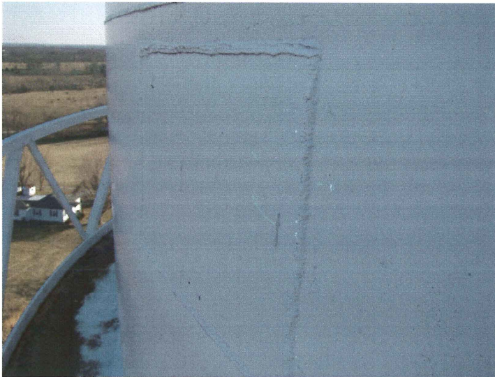
Photo shows the patch plate on the northwest lower shell. The horizontal welds inside the tank are covered with rust.
