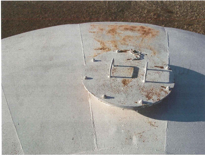
Photo shows the south section of the roof and the 24" diameter secondary roof hatch. The roof finger panel beyond the hatch is covered with active corrosion.
