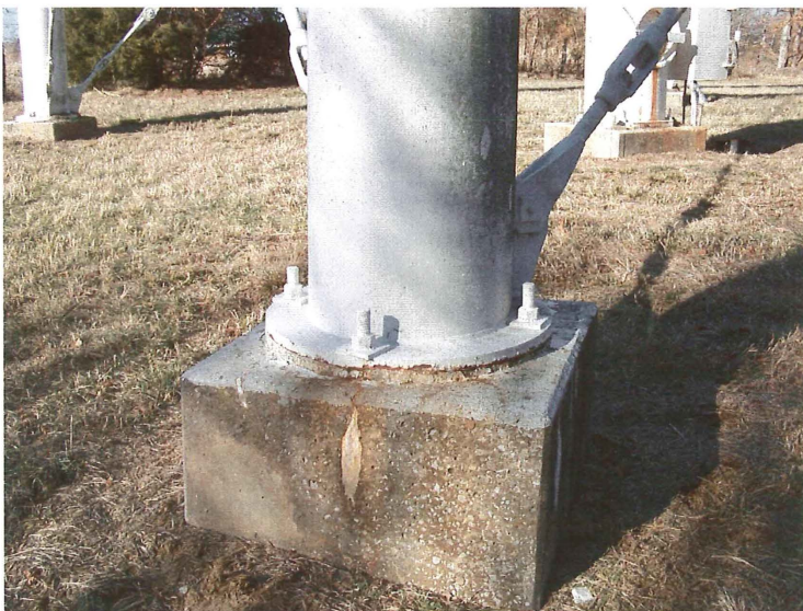
Photo shows the base of the southeast leg. Minor rust is visible along the column flange to grout interface. Each 24" diameter leg has four 1¼" anchor bolts. The anchor bolts are in sound condition.
