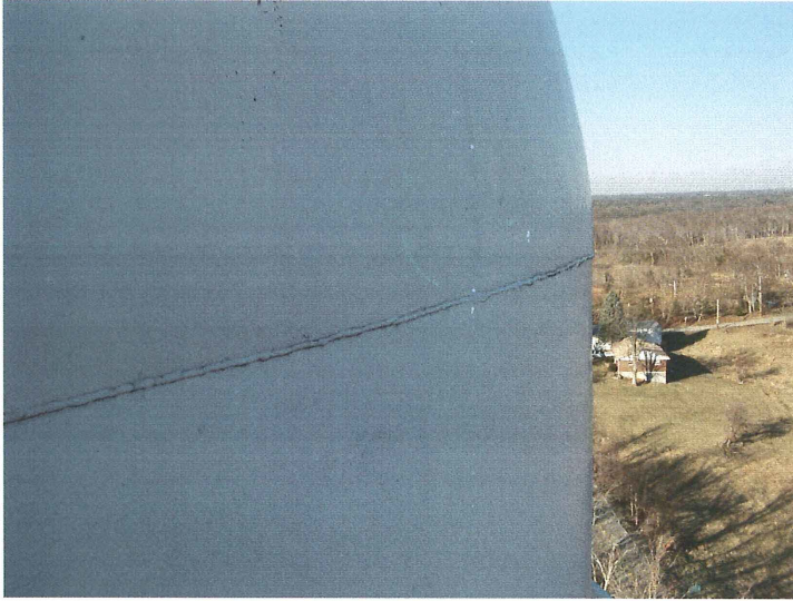
Photo shows the upper knuckle to shell weld seam. All welds were structurally sound.
