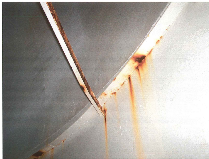
Photo shows active crevice corrosion along the bottom side of the painter's ring angle. The skip-welded angle should be sealed with caulk following the application of the finish coat of epoxy.
