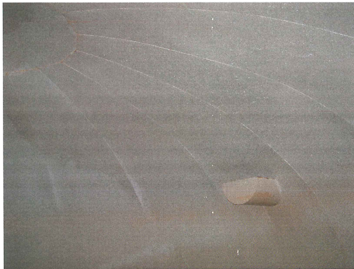
Photo shows the west section of the roof finger panels and the upper knuckle. The overflow weir trough is visible. No significant corrosion was noted.
