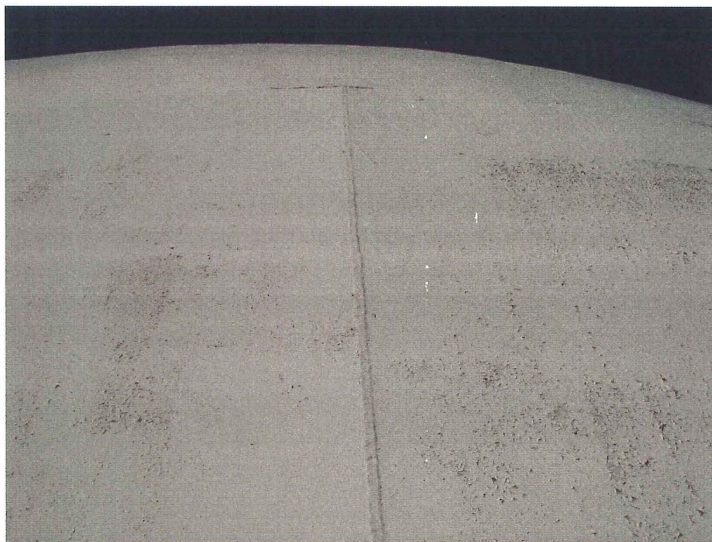
Photo shows a vertical weld on the south upper shell. The finish coat is brittle and has checked.
