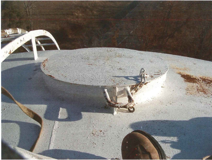
Photo shows a closer view of the 24" diameter roof access hatch. The hatch has a lockable hasp. The hatch was not secured with a lock.
