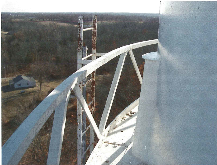
Photo shows the northeast section of the balcony where the leg ladder attaches. An opening should be cut into the handrail so that a climber can step through safely.
