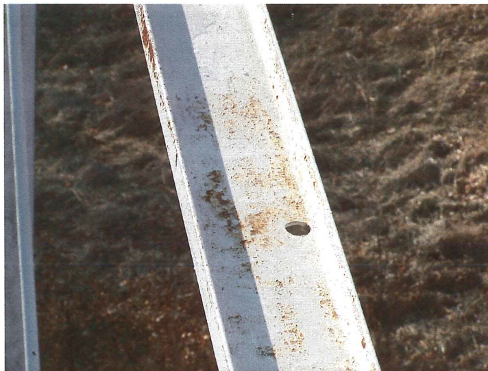
Photo shows blotchy corrosion on the topside of the upper 8" channel.
