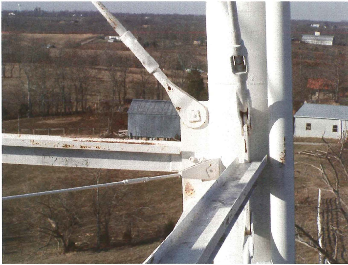
Photo shows the northwest leg at the upper strut level. The 6" overflow pipe is attached to the leg. The coating is starting to fail on all tank members.
