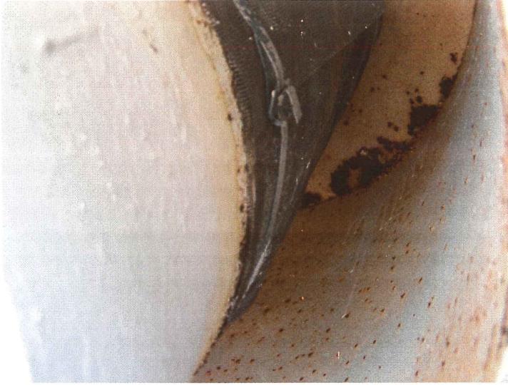
Photo shows the insect screen inside the vent cover. The screen is secured with a stainless steel aircraft clamp. The coating inside the vent cover has started to fail.
