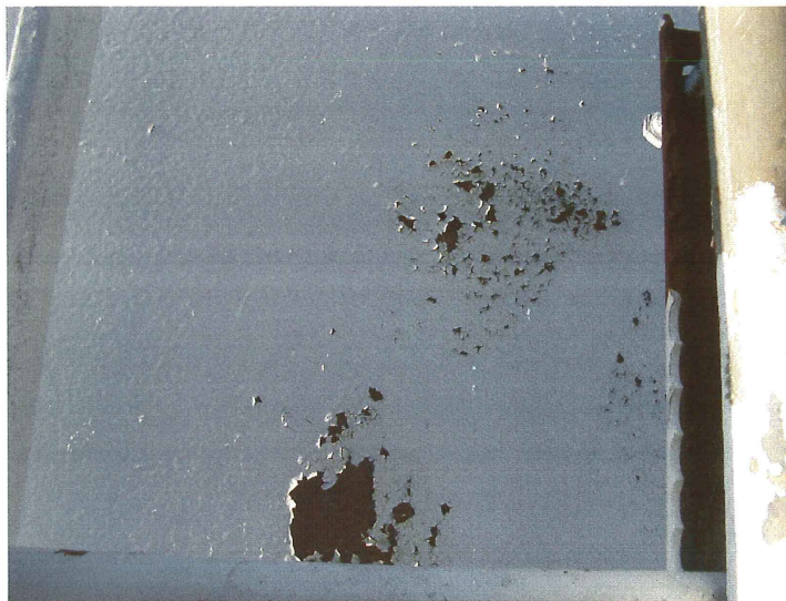
Photo shows corrosion cells on the upper shell behind the ladder.
