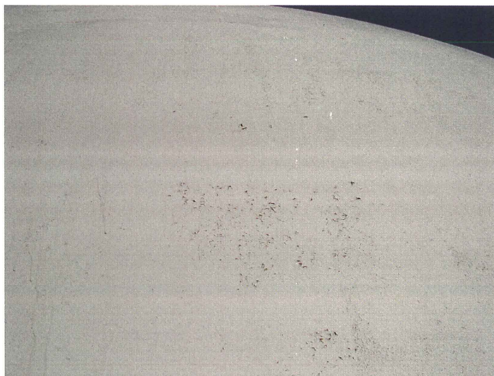
Photo shows the west upper shell. The checked sections are starting to delaminate.
