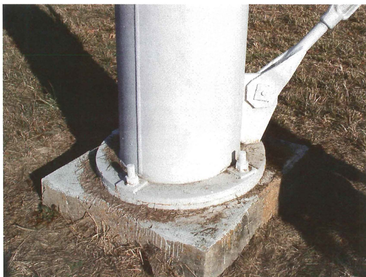
Photo shows the base of the southwest leg. The anchor bolts and concrete are in sound condition.
