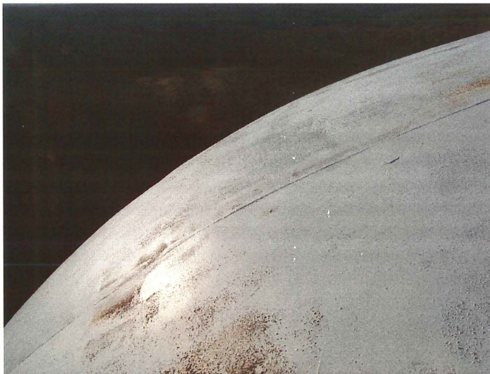
Photo shows the middle section of the northeast upper knuckle. The tank has been previously overcoated. The finish coat has checked and has allowed rust to form.
