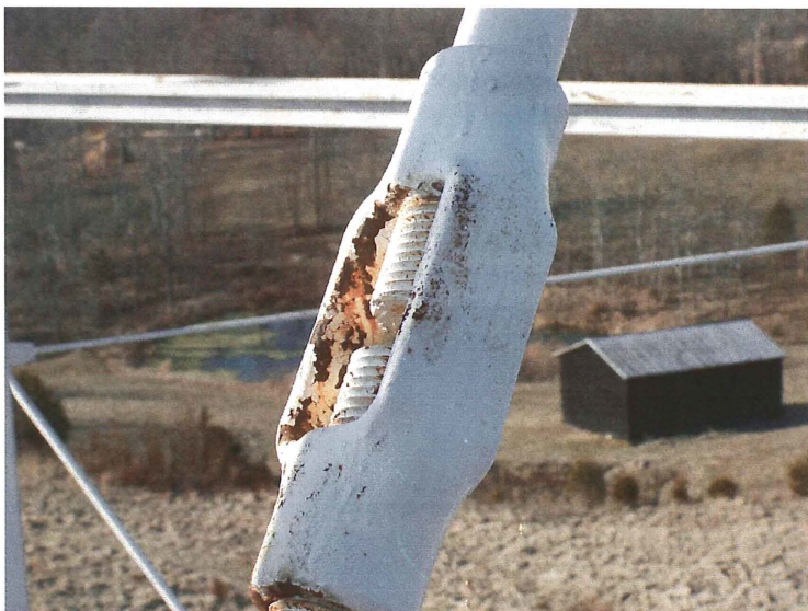
Photo shows active corrosion inside and upper panel windage rod turnbuckle.
