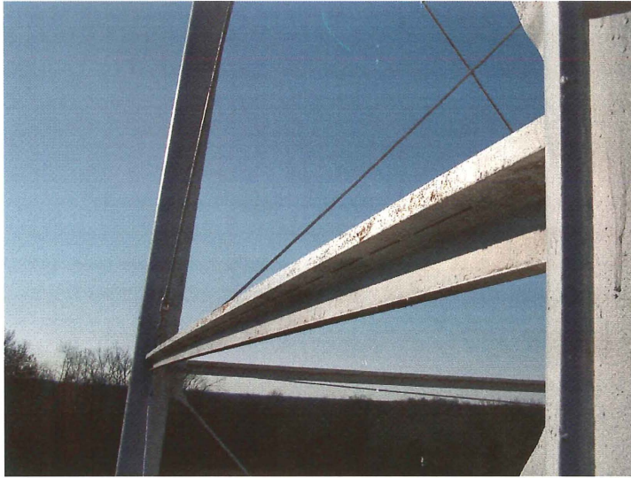
Photo shows the east lower channel strut. The brittle coating has checked and is starting to delaminate.
