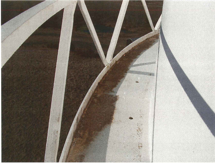
Photo shows the south section of the balcony. The balcony is 24" wide and has a 42" tall handrail.
