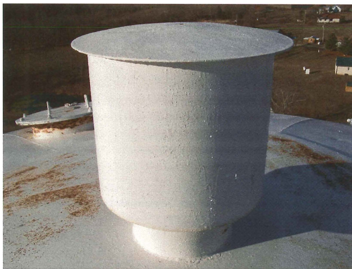
Photo shows the cover for the 12" diameter vent pipe. The bolt that secures the cover is missing. Active corrosion is visible on the roof cap plate.
