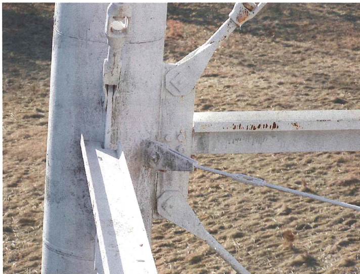
Photo shows the southeast leg at the upper strut level. The struts, windage rods and the riser stay rod connect at this point. All connections appear sound.
