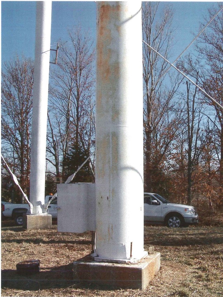
Photo shows the west side of the lower section of the riser pipe. The coating no longer protects the steel.
