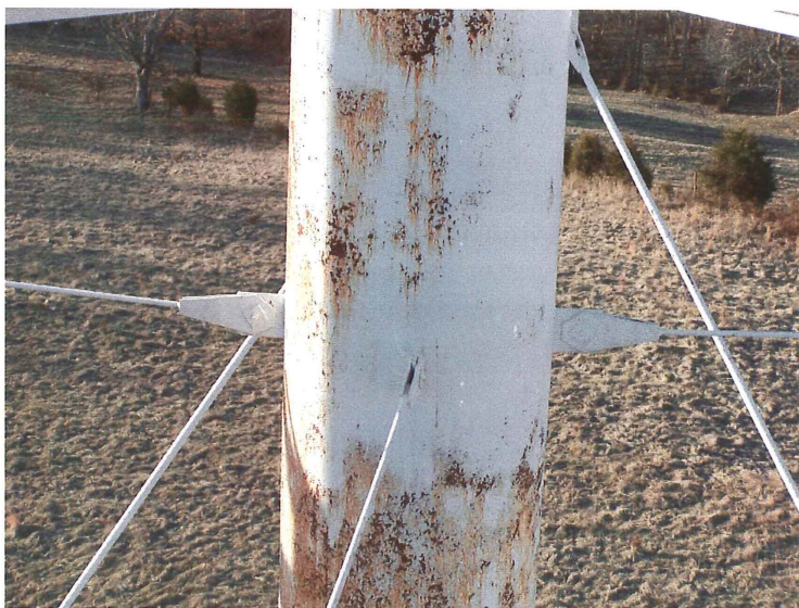
Photo shows the riser pipe at the upper strut level. The riser stay rod connections appear sound..
