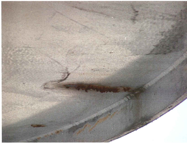
Photo shows a spot on the underside of the north balcony where the coating has delaminated.
