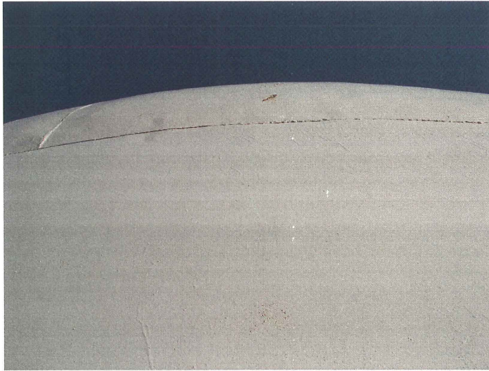
Photo shows the west upper shell. The coating continues to protect the steel substrate but has lost all gloss.
