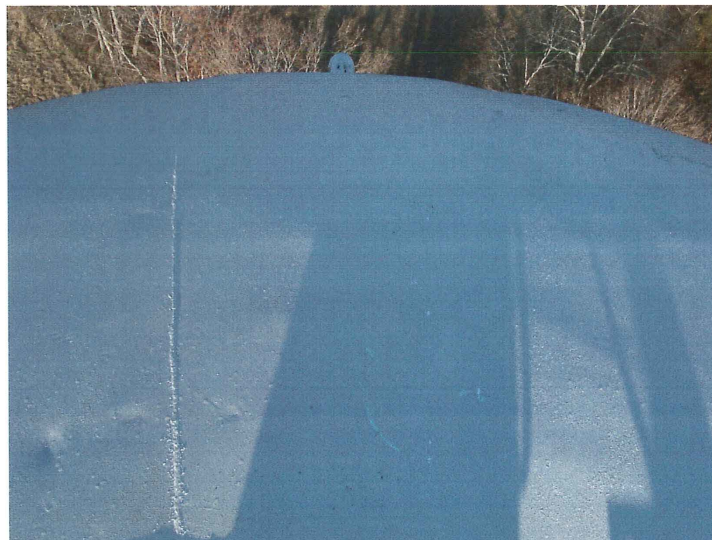
Photo shows the northwest section of the roof. The white finish coat has lost its gloss and is very brittle.
