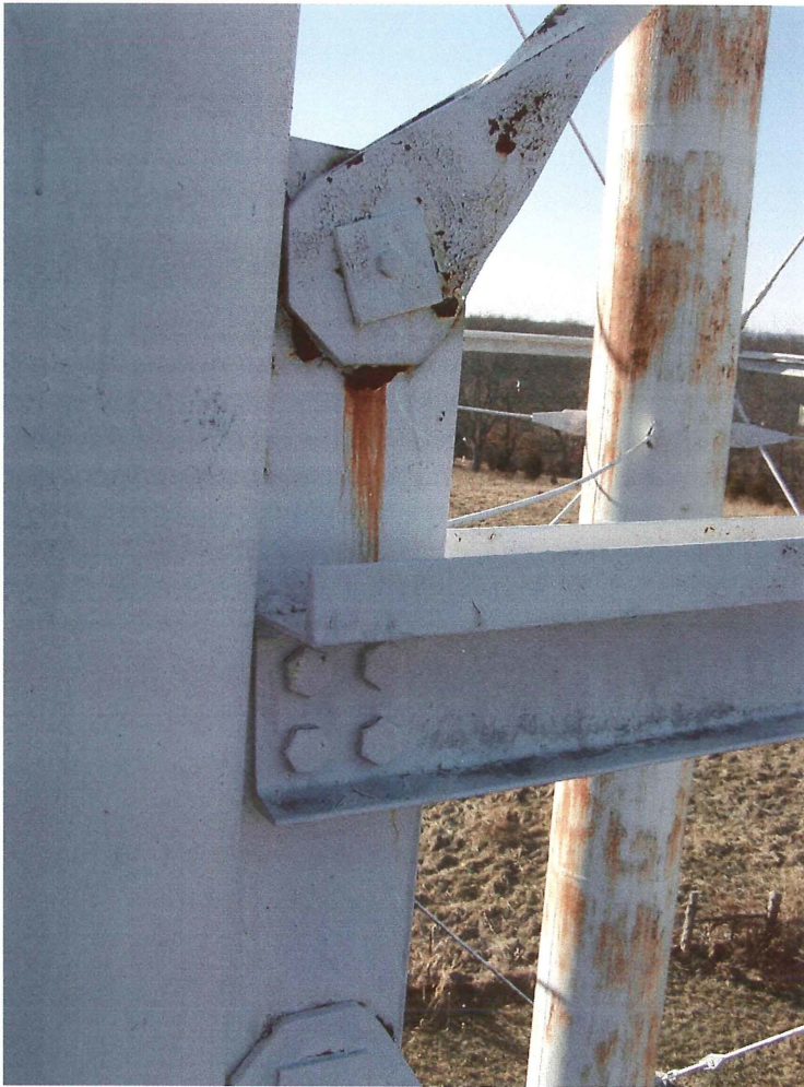
Photo shows the lower north strut at the point where it connects to the northeast ladder leg. The bolted and pinned connections appear sound. Crevice corrosion is visible at the pinned windage rod connection.
