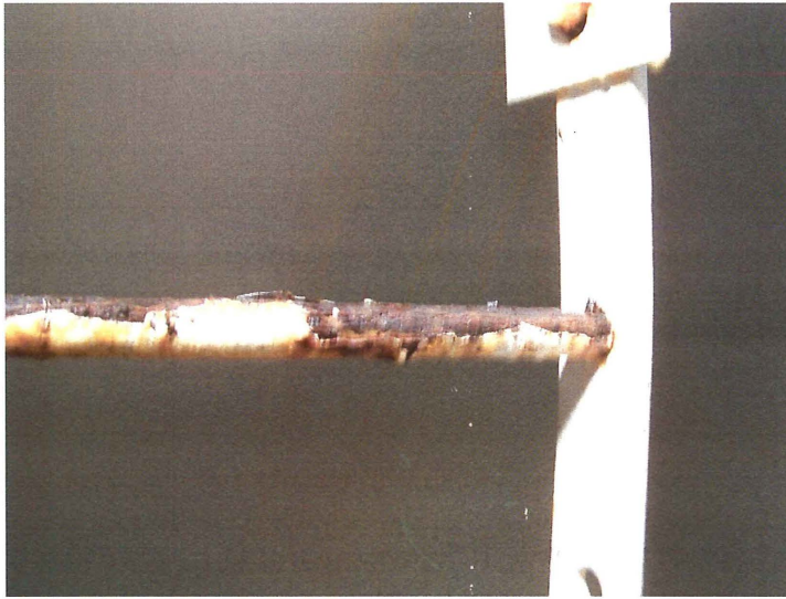
Photo shows the top ladder rung that is severely deteriorated and should be replaced.
