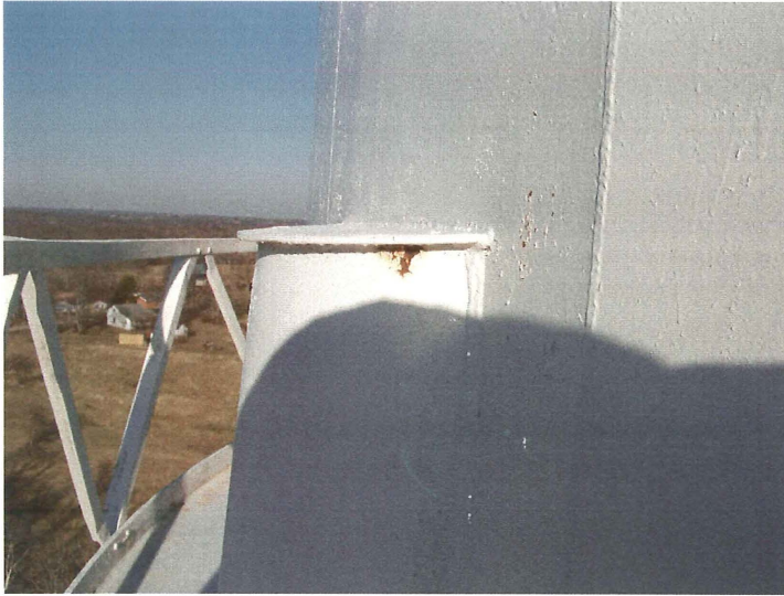
Photo shows minor rust under the post head cap plate.
