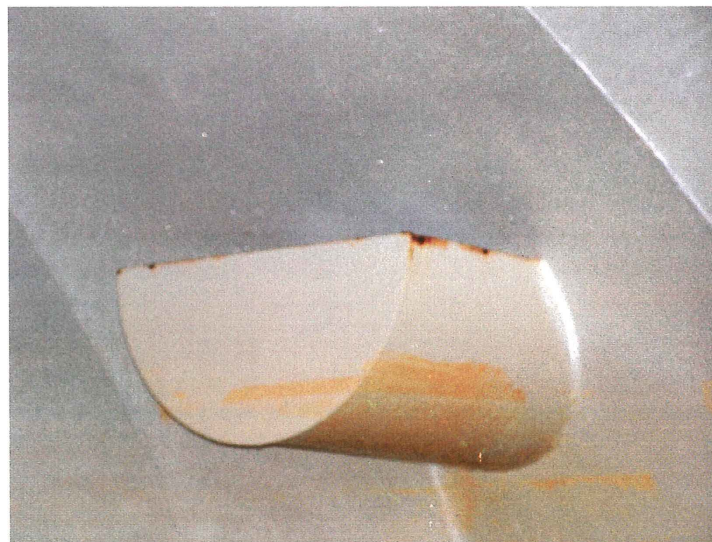
Photo shows a close-up of the weir trough. The epoxy coating is failing along the edges.
