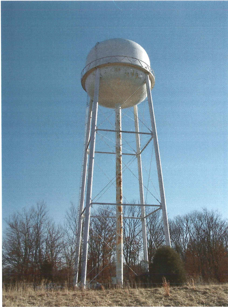
Photo shows an overall view of the west side of the tank. The tank has three panels and two struts. The overflow pipe runs down the northwest leg.
