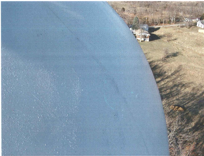
Photo shows the lower section of the north upper knuckle. No active corrosion was noted.
