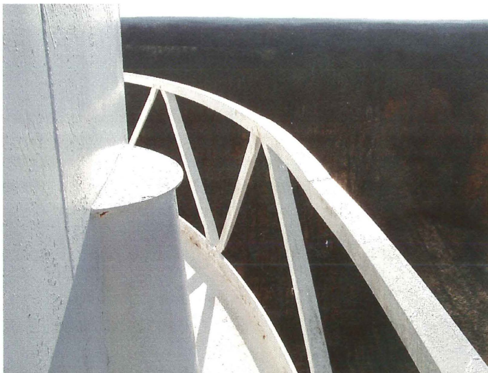
Photo shows the southwest section of the balcony. The handrail is bent slightly inward at this point.
