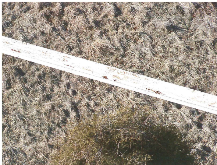
Photo shows the middle section of the west lower strut. The coating has failed in numerous areas especially along the edges.
