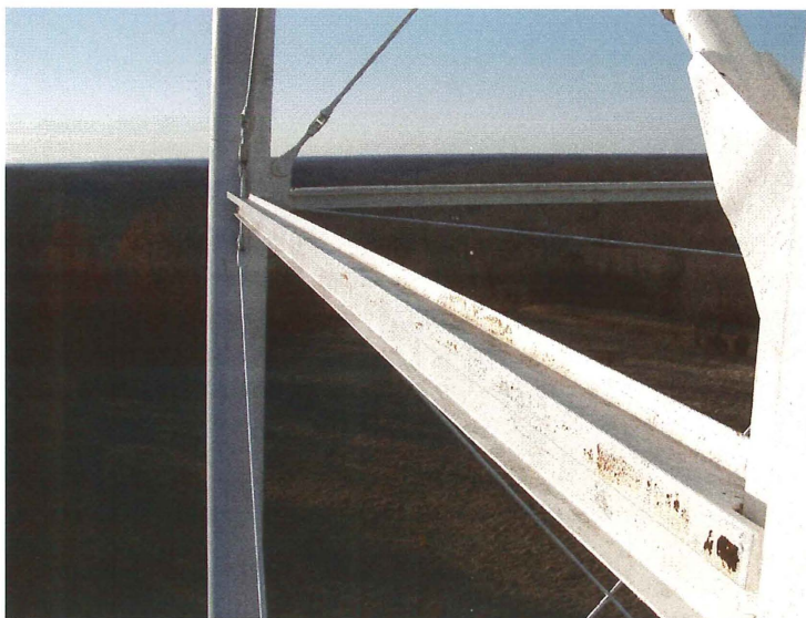
Photo shows the east upper strut. The strut is constructed of a 8" channel over a 6" channel to form a "T". All struts were properly aligned.
