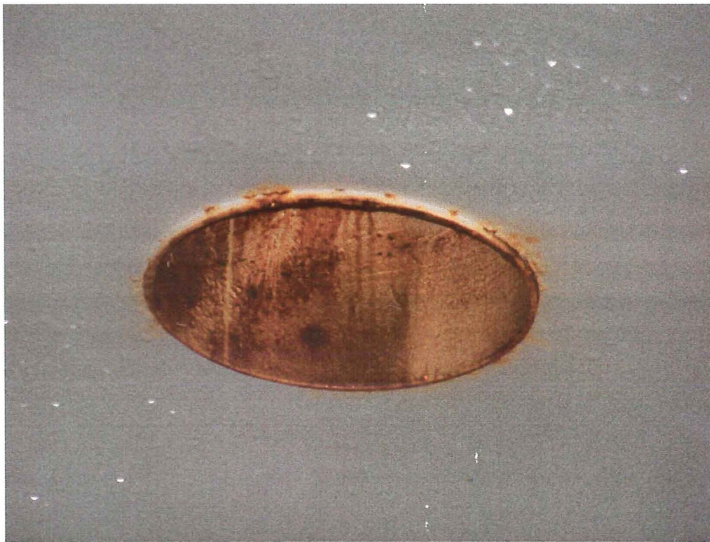
Photo shows a close-up of the 12" roof vent pipe. The interior surfaces are covered with blotchy corrosion.
