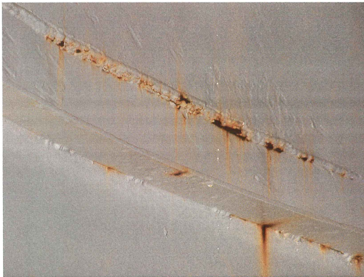
Photo shows a close-up of the area shown above. The white epoxy coating has failed along the sharp edges of the rough weld seam.
