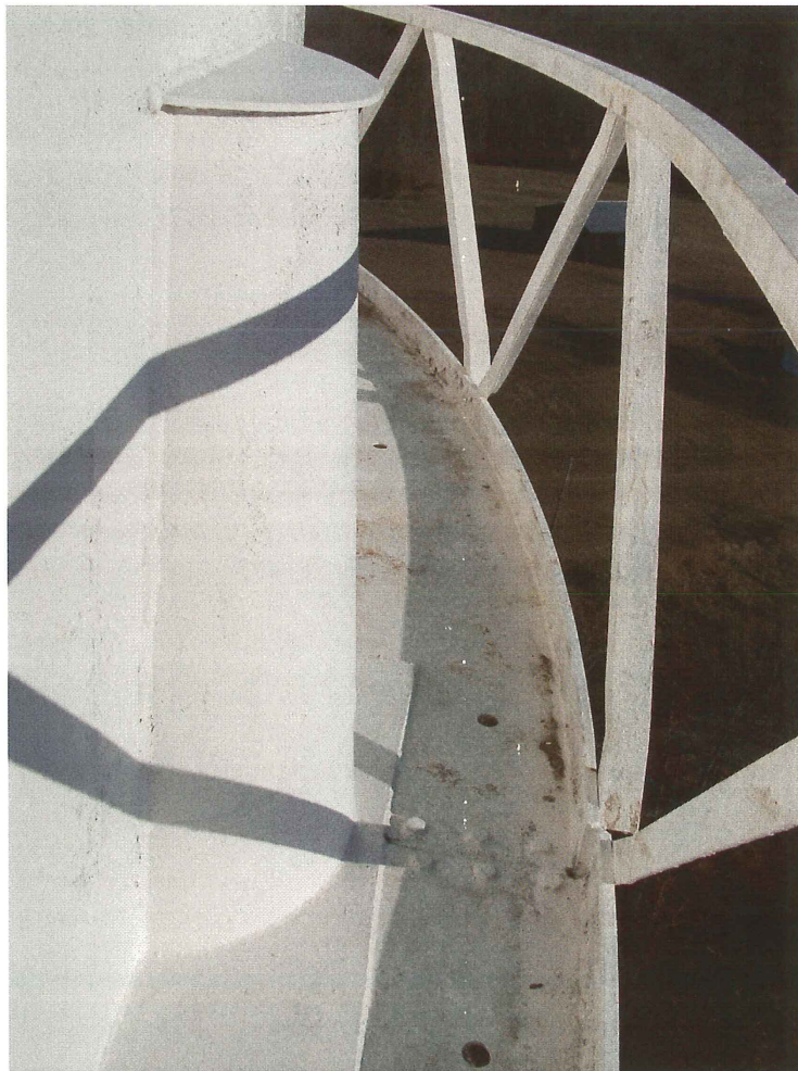
Photo shows a typical post head and sail plate where the leg attaches to the shell. All connections appear sound.
