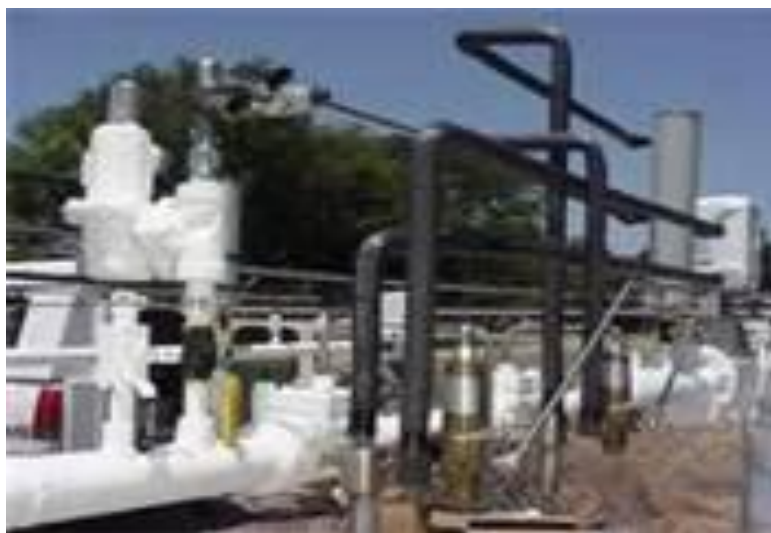
Typical Installation with Downstream Flow Control Regulator
