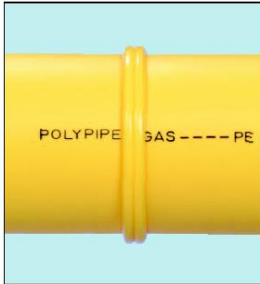
Melt bead too large due to excessive heating and/or over-pressurizing of joint.
