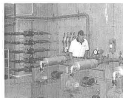
System Manager Richard Webber inspects the system's pulsator clarifier blowers. Alliance provided planning and management for the financing, design and construction of this new system, resulting in a capital savings of more than $1.5 million.
