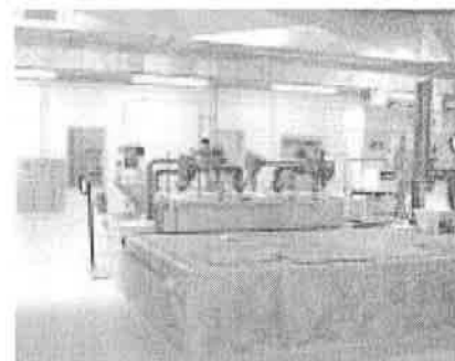
In 1999, Henry County Water Company constructed a new 2.4-MGD single pass pulsator flocculator/clarifier water treatment plant with dual-media gravity filtration.
