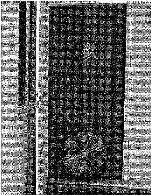
Researchers are evaluating the effect of air-tightening practices on blower-door air-infiltration rates to determine if adequate air is available for appliances.
