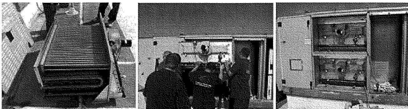
Condensing heating module (left) being installed (center) and with both modules in place in the DOAS (right).
