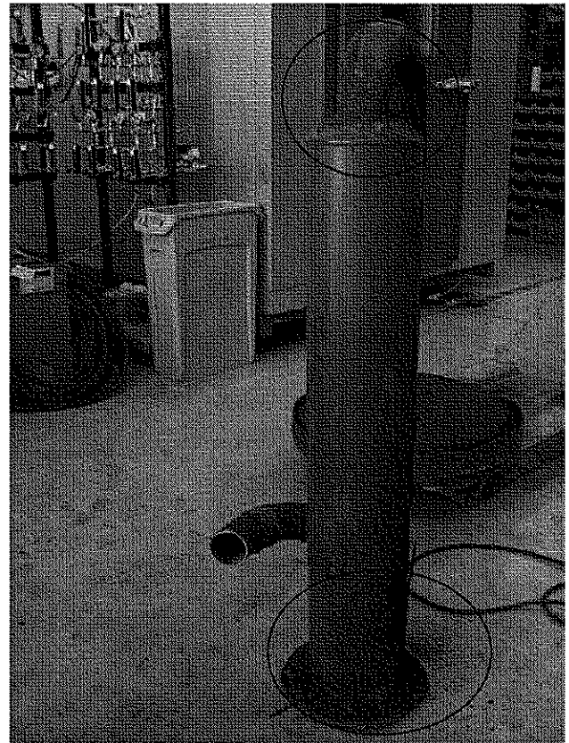
Heat exchanger shows signs of heavy usage; accelerated glass degradation (circled).
