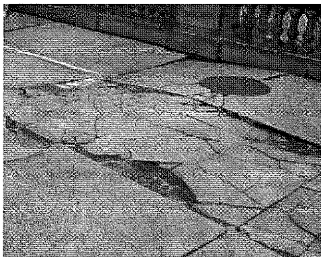
Frost heave formation at the pavement surface.
