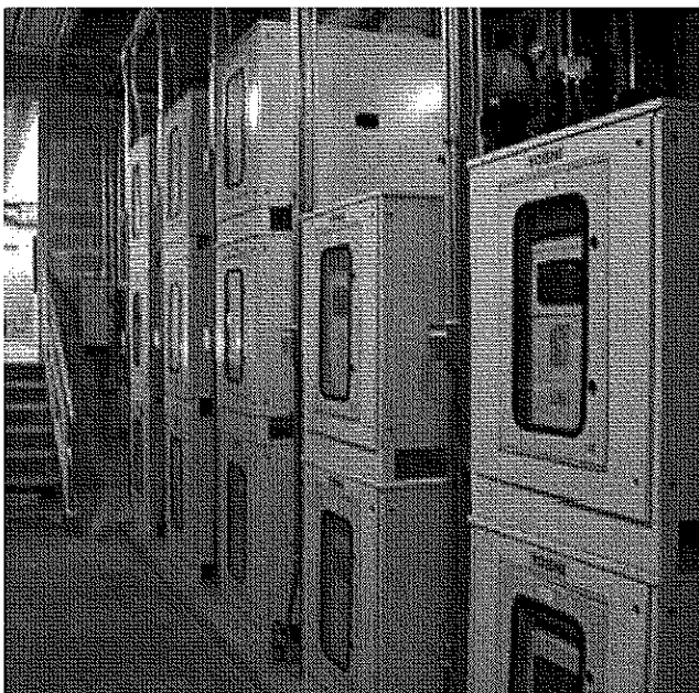
Chiller Link heat exchangers were used to retrofit the GHPs to an existing four-pipe hydronic HVAC system.
