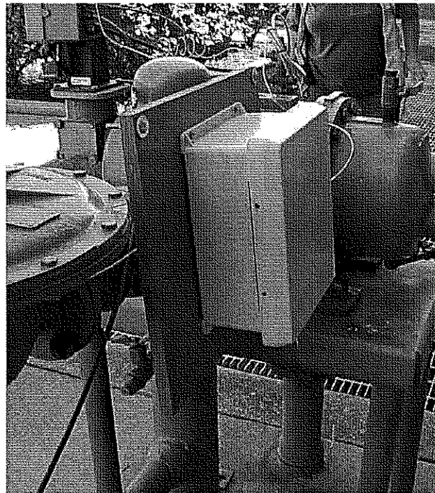
Prototype deployed at utility site.
