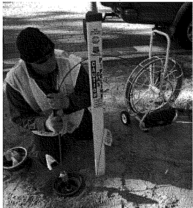
Line tracer system accessible through a valve box.
