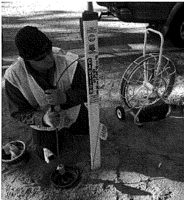
Line tracer system accessible through a valve box.
