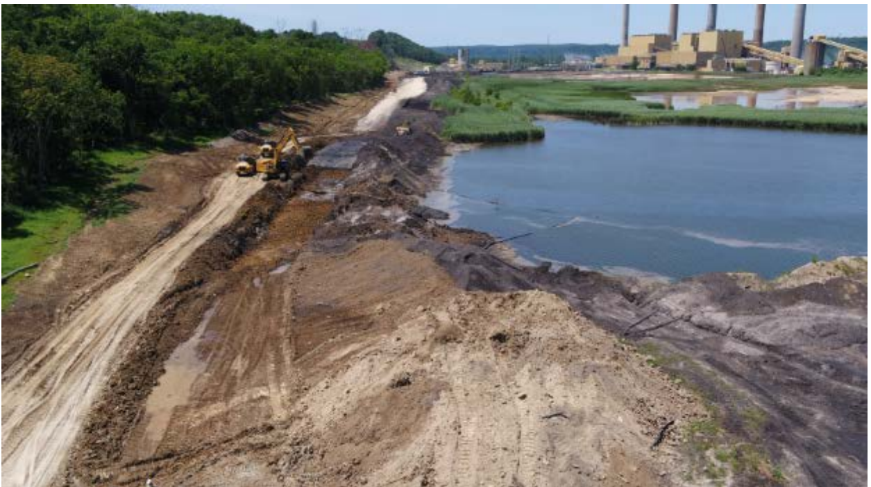
Ghent ATB #1 Cooling Channel – Looking West
