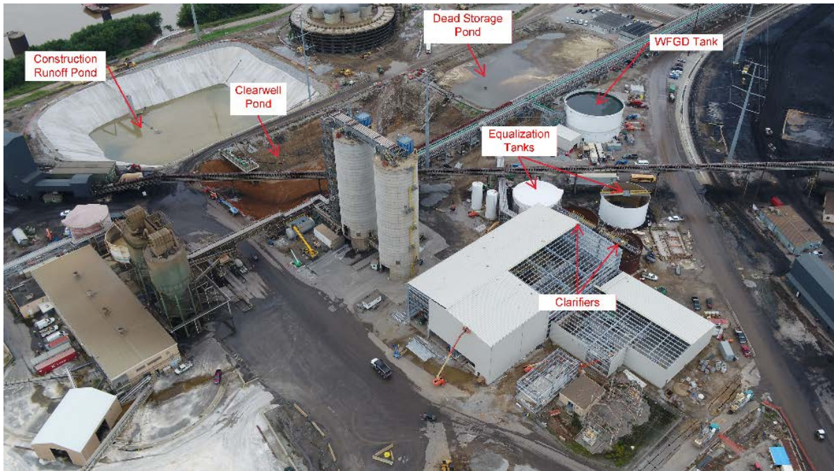
Mill Creek PWS Facility – Site View – October 2018
