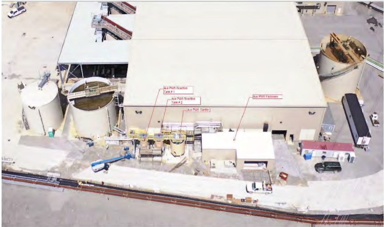
E.W. Brown PWS Treatment System – June 2019
