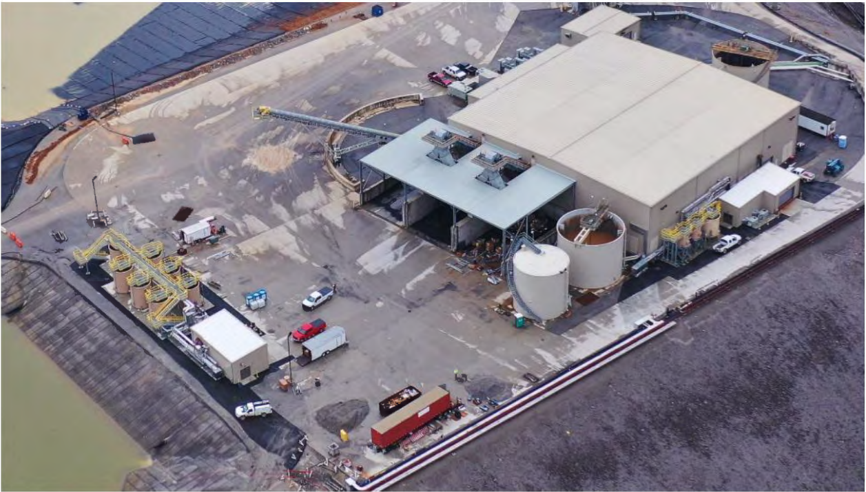
E.W. Brown Toe Drain and Coal Pile Runoff Treatment System – December 2019
