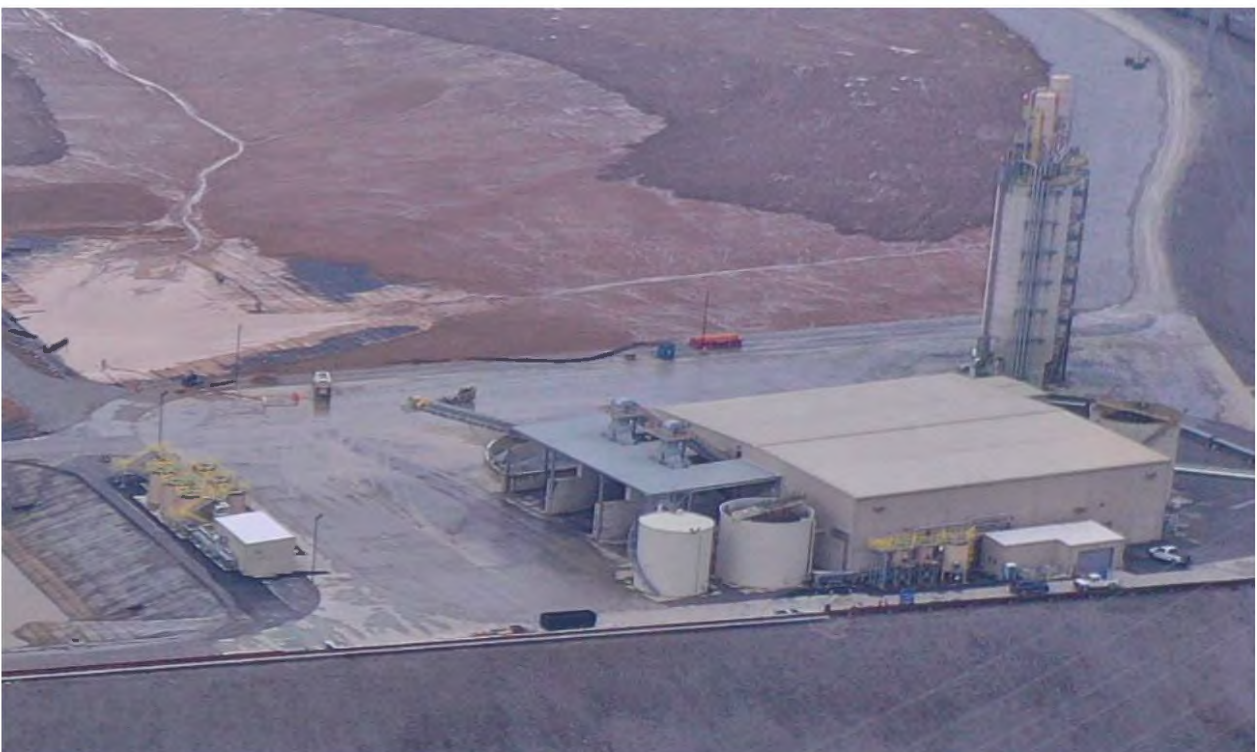
E.W. Brown Toe Drain and Coal Pile Runoff Treatment System – March 2020
