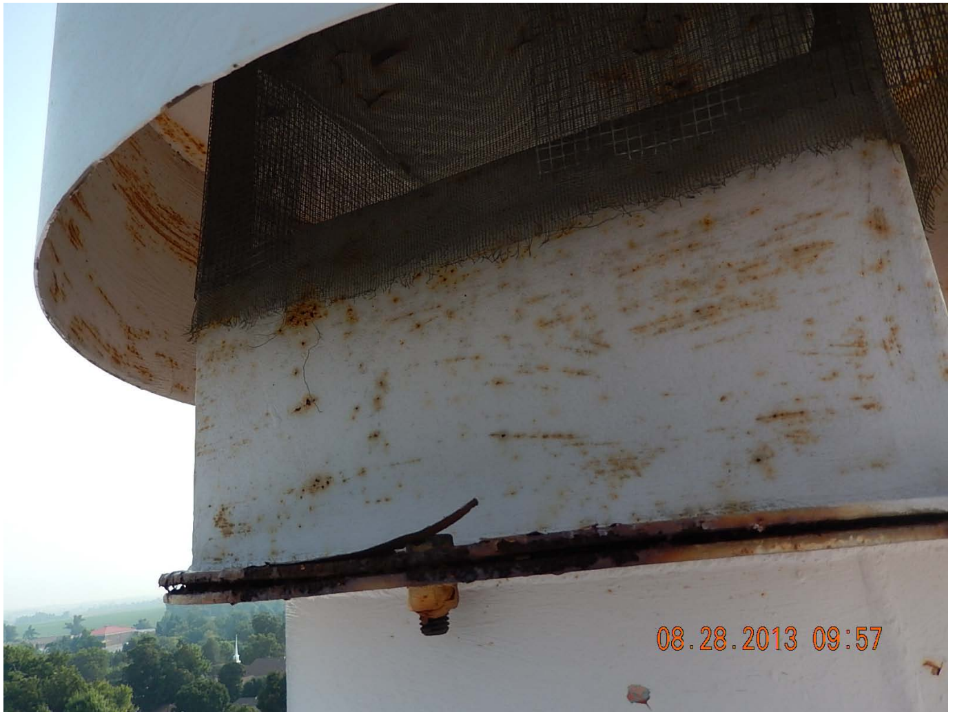
Vent screen and rust
