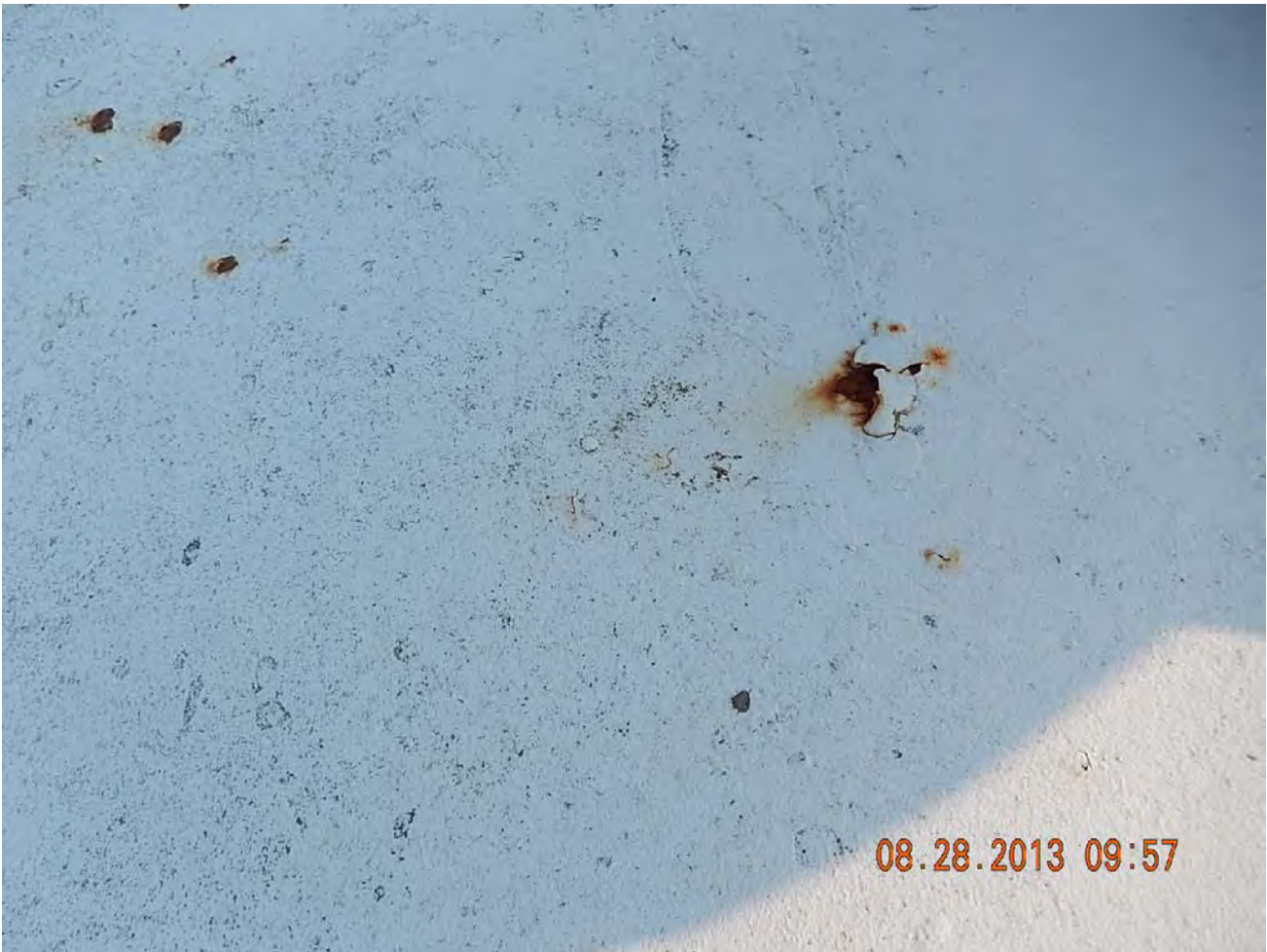
Small failures on roof
