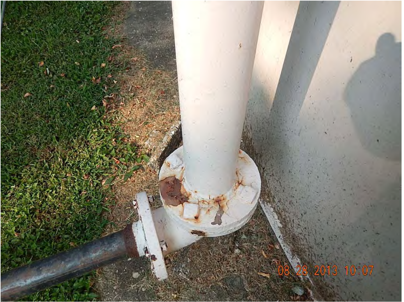
Same on overflow
