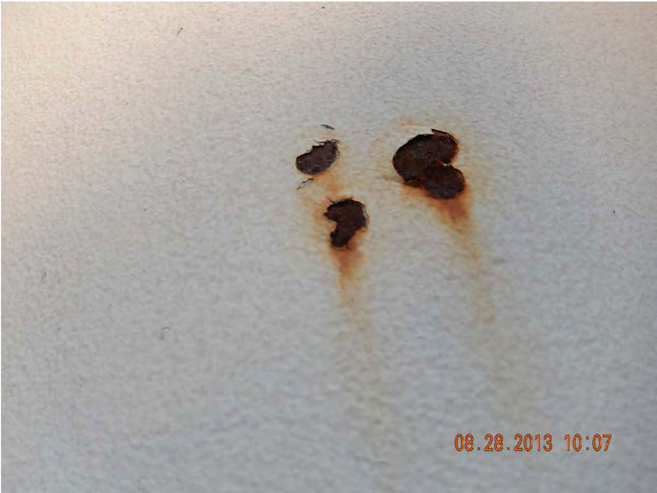
Tank sidewall coating failures
