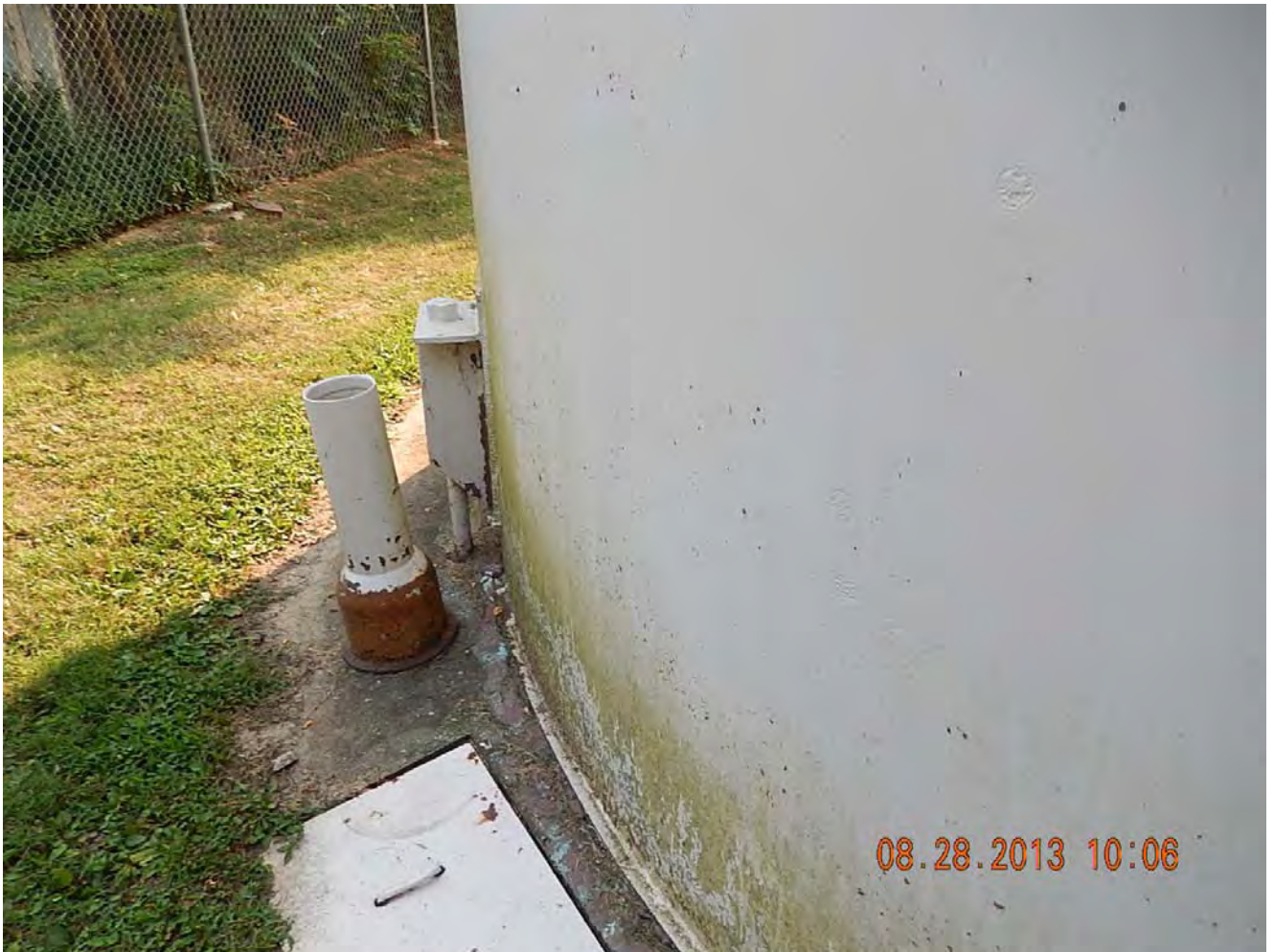
Tank to foundation note algae growth at base this is where tank sweats
