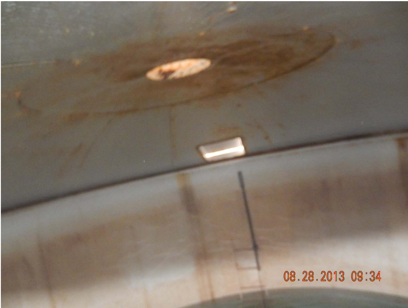
Interior roof and sidewall note rusting on both
