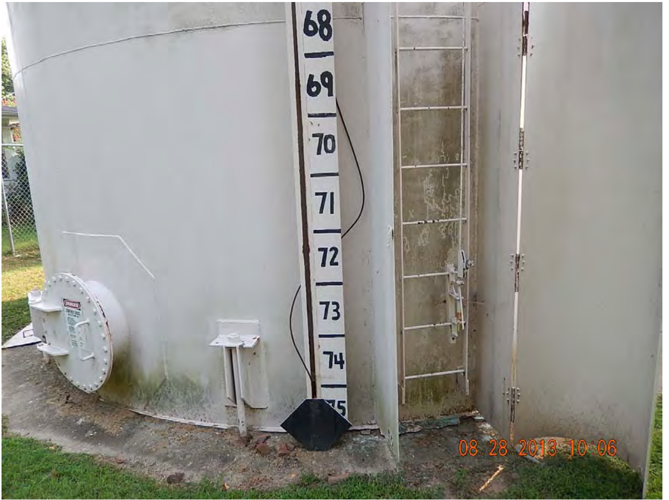
Ladder gate, water level indicator
