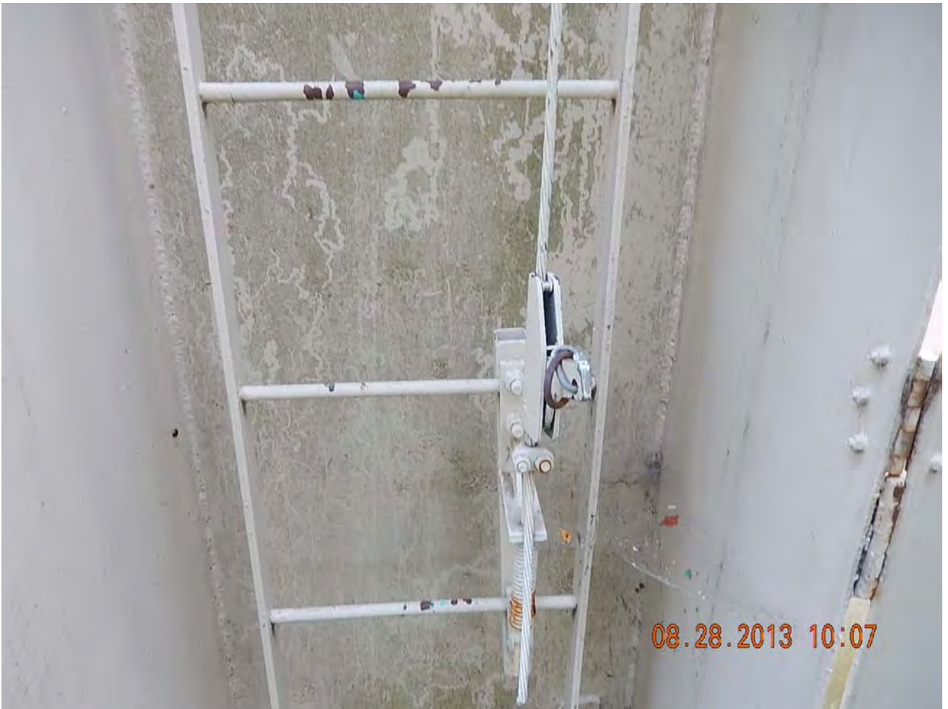
Tank ladder and safety climb
