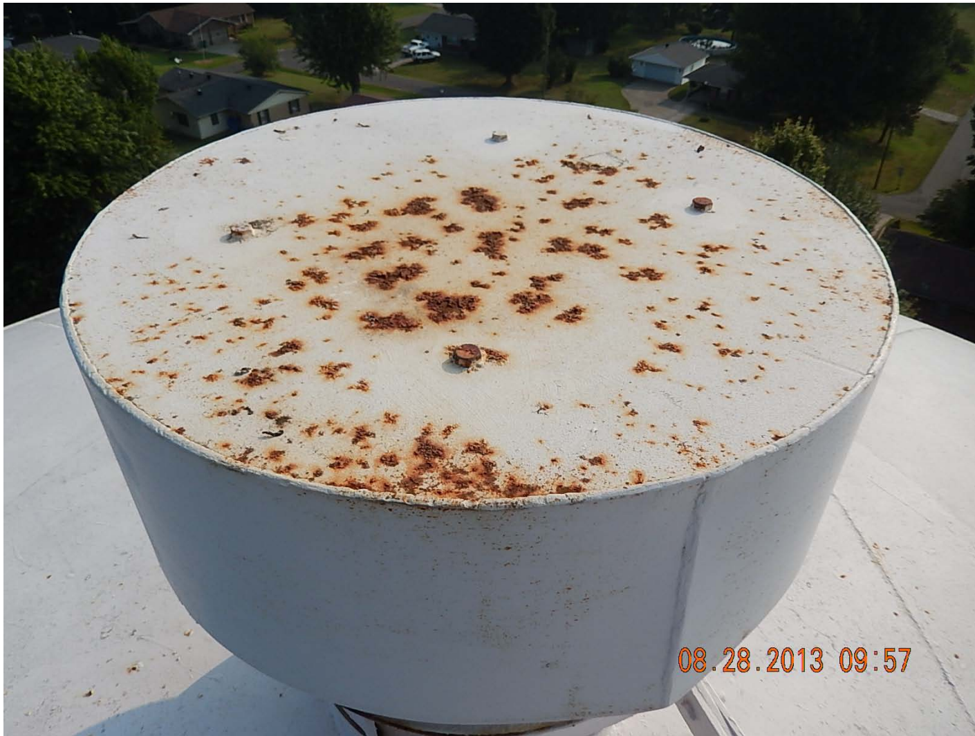
Roof vent failing coating
