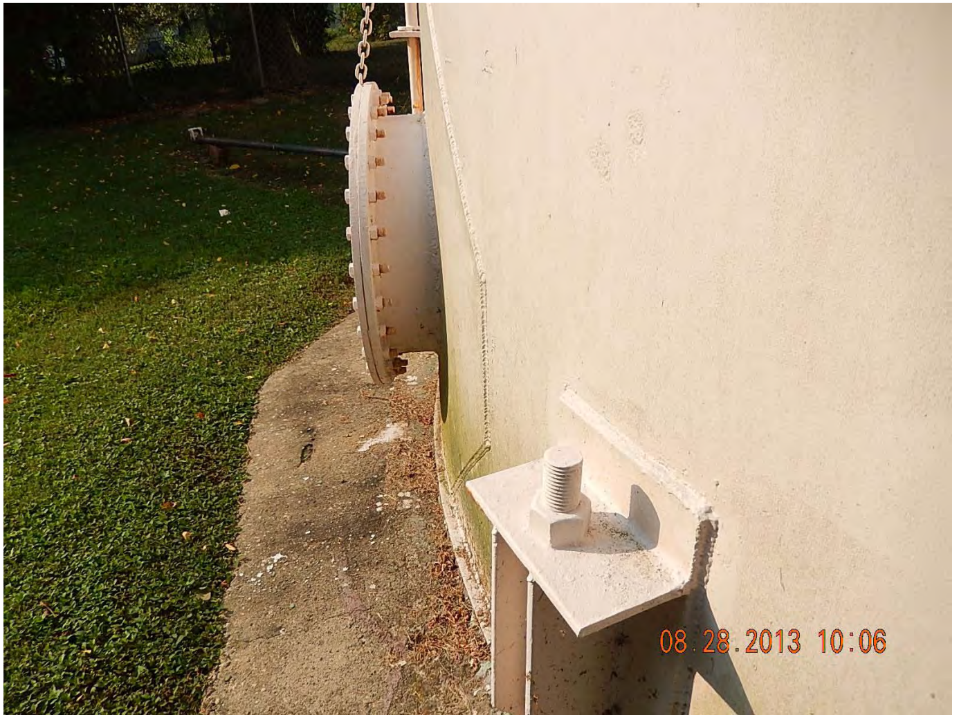
Lower manway, foundation
