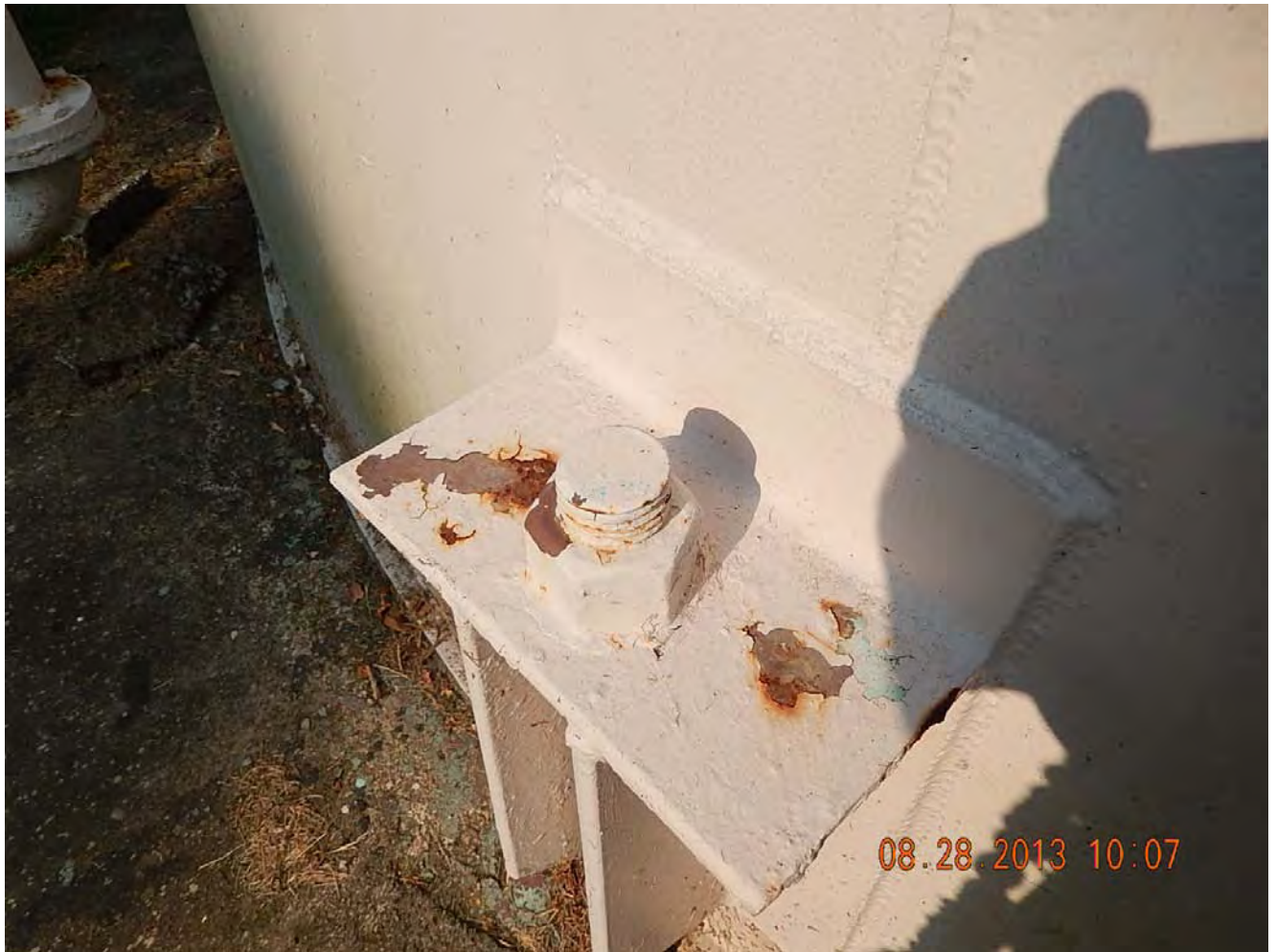
Coating failing on anchor bolt chair
