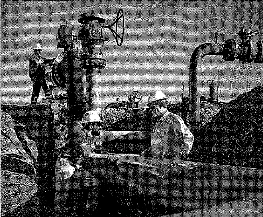
LEFT: Our strategy today is to invest in our infrastructure to ensure safe and reliable service. A major transmission project during fiscal 2013 was our 24-inch Line WX, being installed west of Fort Worth, Texas. It will help Atmos Pipeline-Texas supply the needs of local gas distribution utilities in the state.
