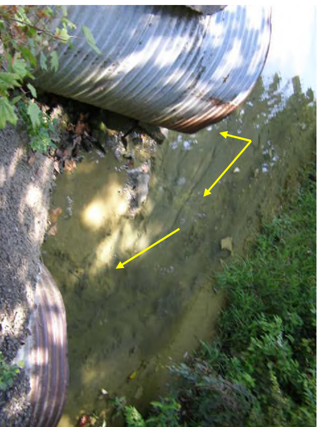
Spillway passes through two culverts under facility drive and enters Mill Creek. Note brownish grey sludge in waterway.
