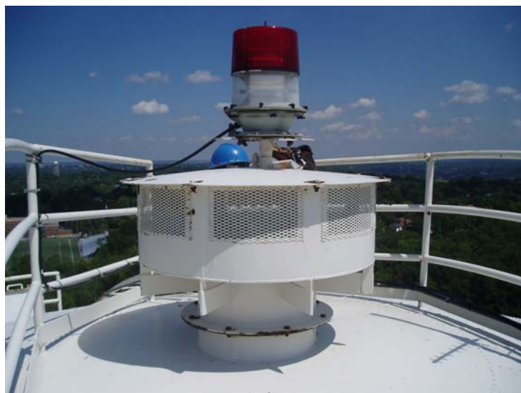
34) View of the roof vent and strobe light/beacon.
