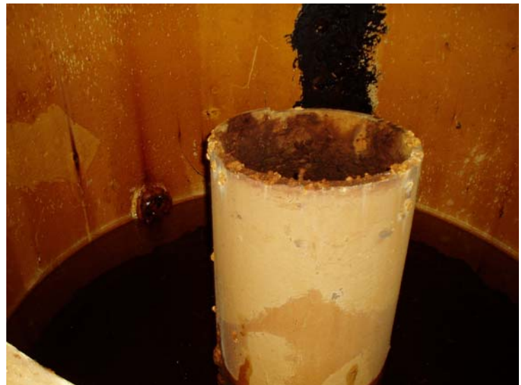
51) View of the fill pipe in the bottom of the riser.
