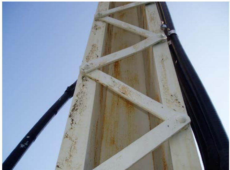
12) Rust bleed through and coating erosion inside of a leg column.
