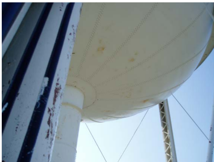
19) Rust bleedthrough on the bowl.
