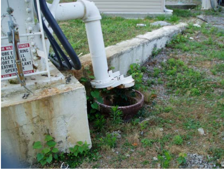
2) Minor foundation deterioration and view of the overflow pipe discharge area.
