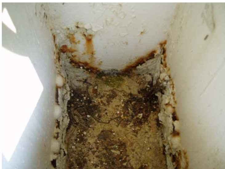
7) Corrosion at the base of a leg column.
