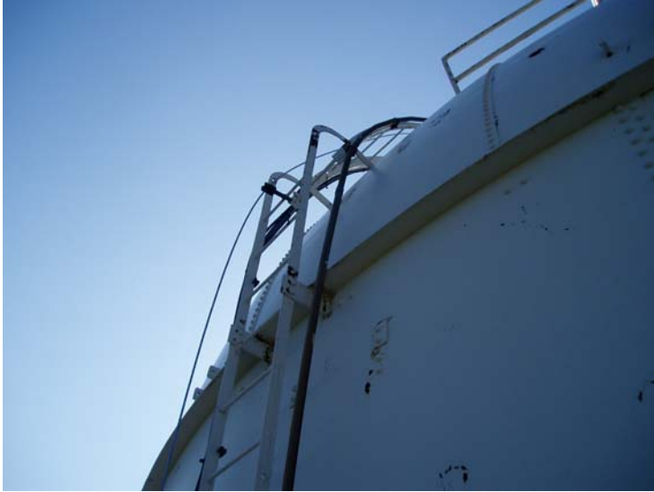
26) Spot coating breaks to substrate on the sidewall.
