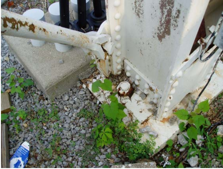
5) Coating deterioration at a leg base and sway rod.
