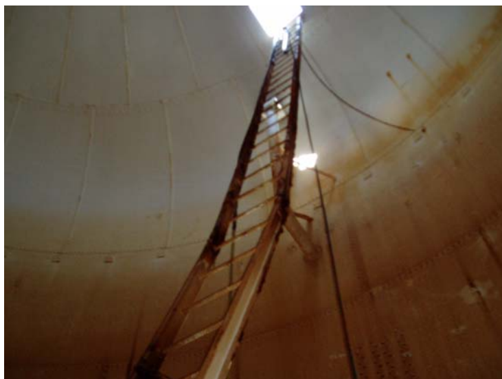
40) Heavy corrosion on the wet interior ladder. The siderails are very brittle. The fall prevention device is corroded and broken.
