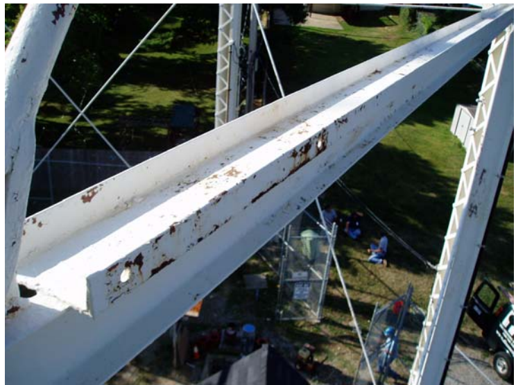
15) Typical coating breaks to substrate and corrosion on a strut.
