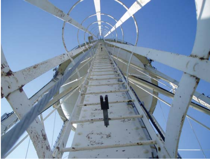
17) Coating breaks to substrate on the leg, leg ladder, and ladder cage.
