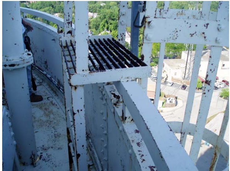
21) Coating breaks to substrate on the step-off platform, the balcony knee wall, and overflow pipe.
