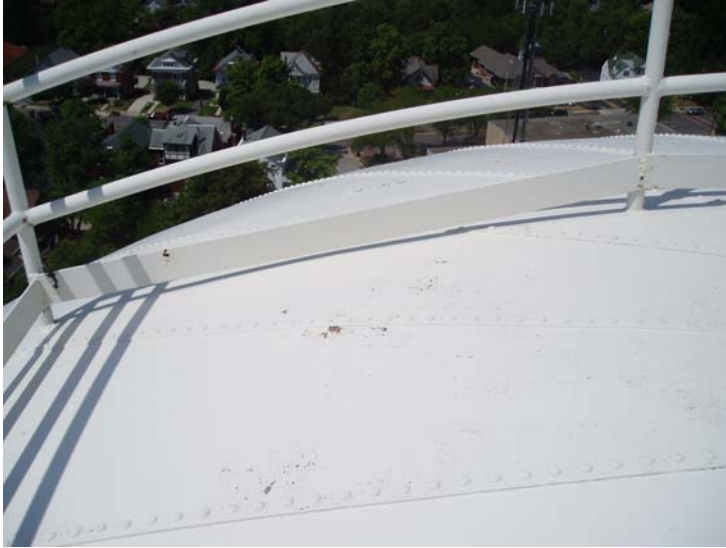
32) Coating breaks to substrate on the roof handrail.
