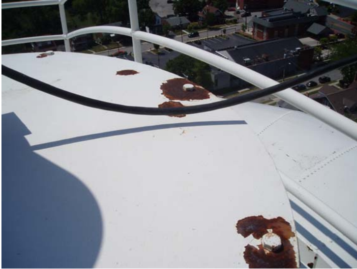
35) Coating breaks to substrate on top of the roof vent.
