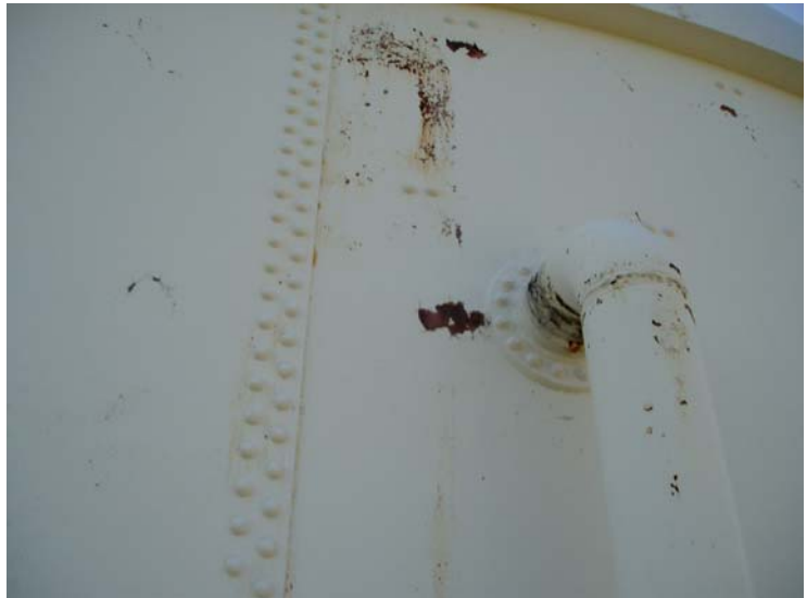
27) Coating breaks and coating erosion on the sidewall and overflow pipe.
