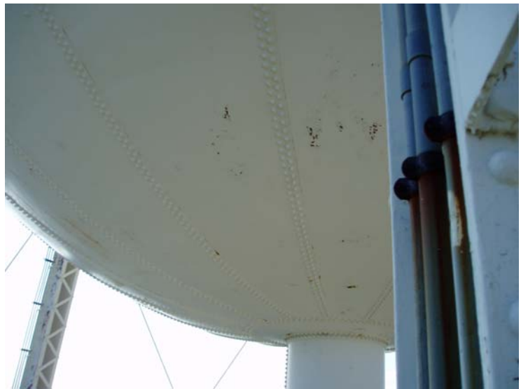
18) Coating breaks and rust undercutting on the bowl.
