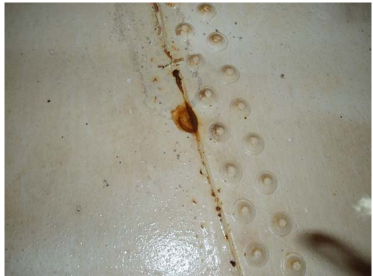
48) Spot coating break at a riveted seam on the floor.
