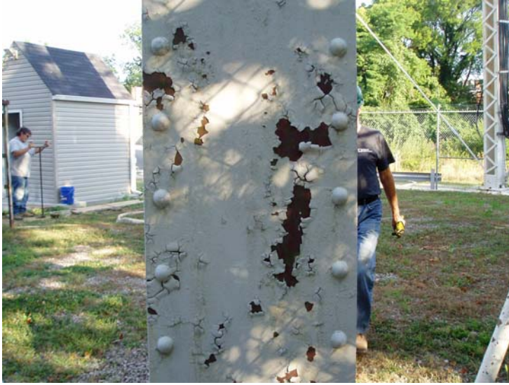
11) Extensive delamination and coating breaks to substrate on a leg. (typical)
