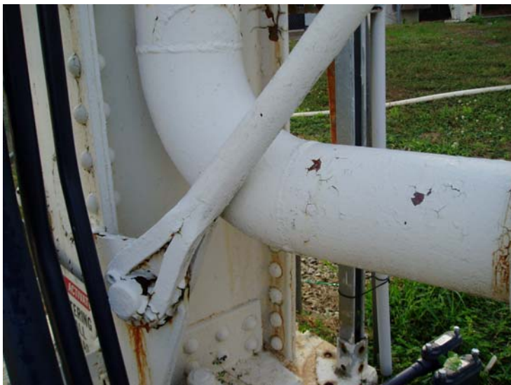
13) Coating deterioration on the overflow pipe and sway rod connection to the leg.
