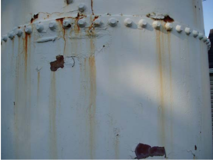
8) Spot coating breaks to substrate and rust staining on the riser.
