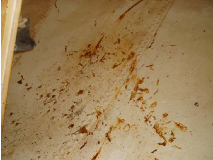
47) Coating breaks and coating damage around the wet interior ladder caused by deterioration of the ladder siderails.
