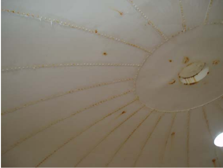
38) Rust bleedthrough at the riveted seams and previous spot repairs on the wet interior roof.
