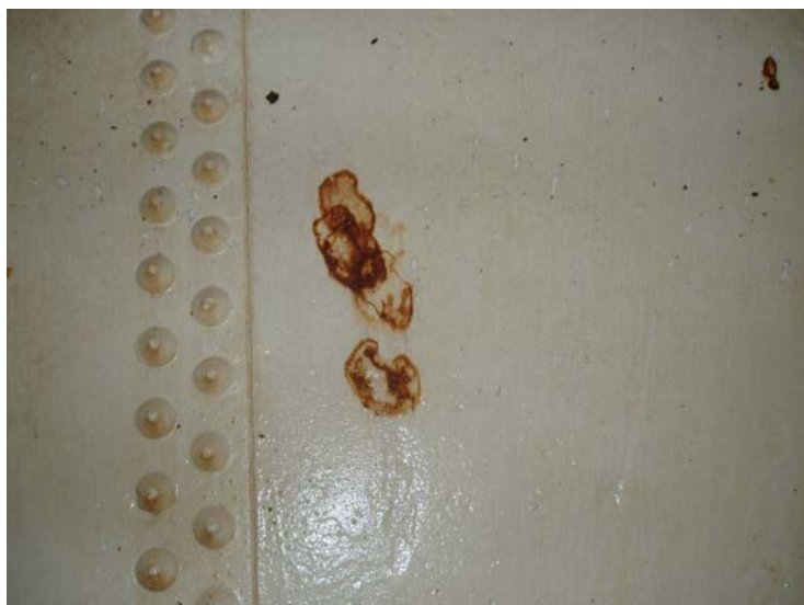
46) Active pitting on the floor.
