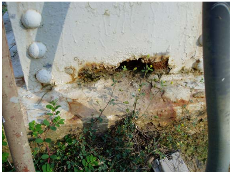
6) Steel corrosion at a leg base.
