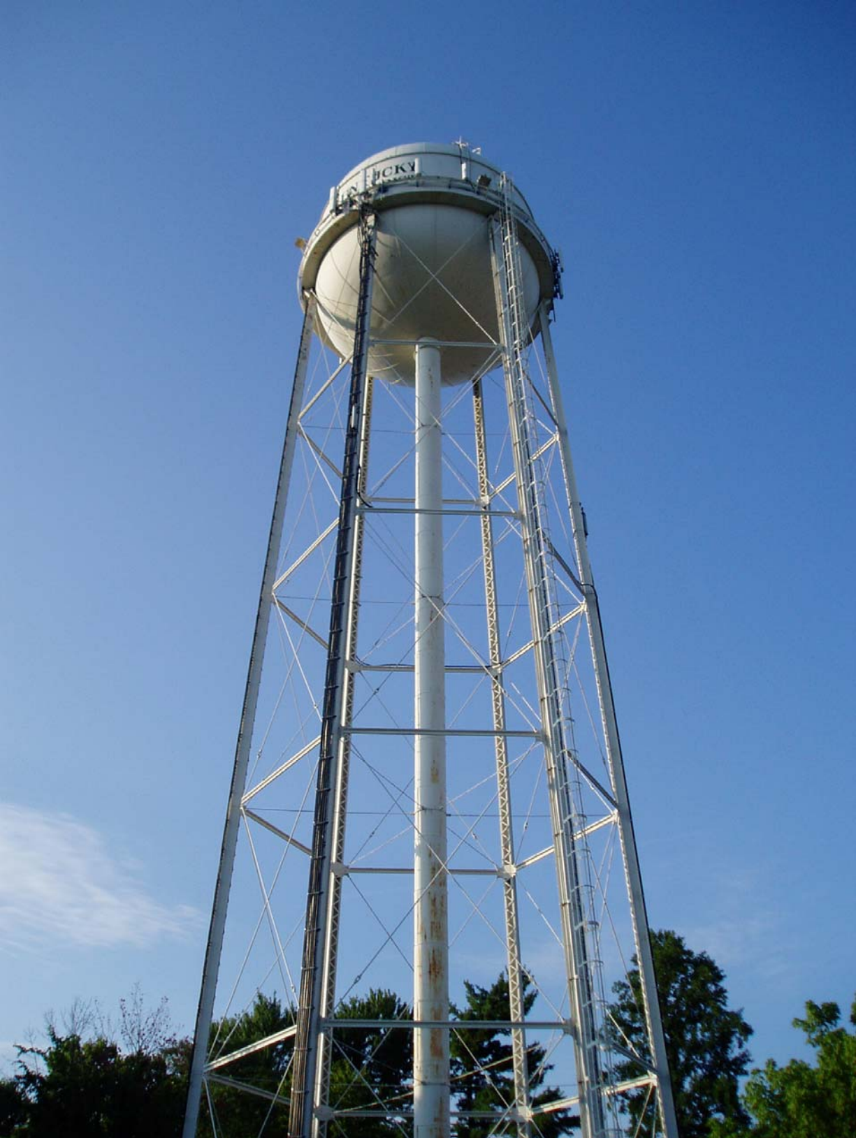
Northwest elevation view of the 275,000 gallon Lumley double ellipse water storage tank owned by the Northern Kentucky Water District in Fort Thomas, Kentucky.
