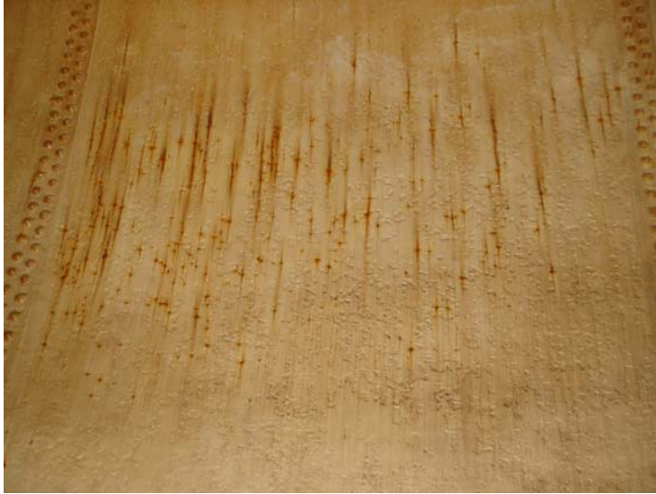
41) Numerous spot coating breaks and rust staining on the sidewall. Extensive pitting prior to the current coating.
