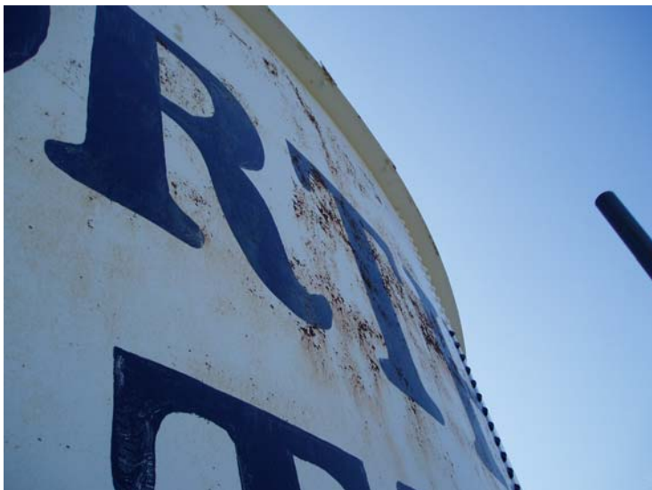
28) Coating erosion on the north sidewall.
