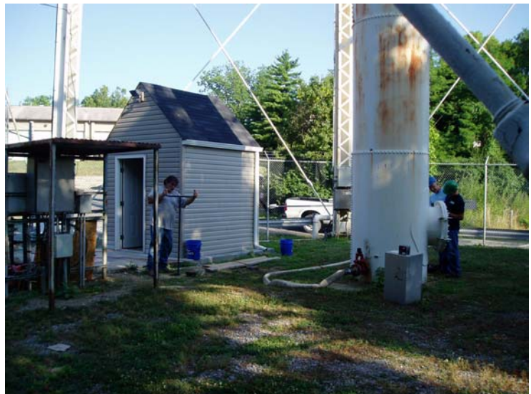
9) Extensive rust bleedthrough on the riser.
