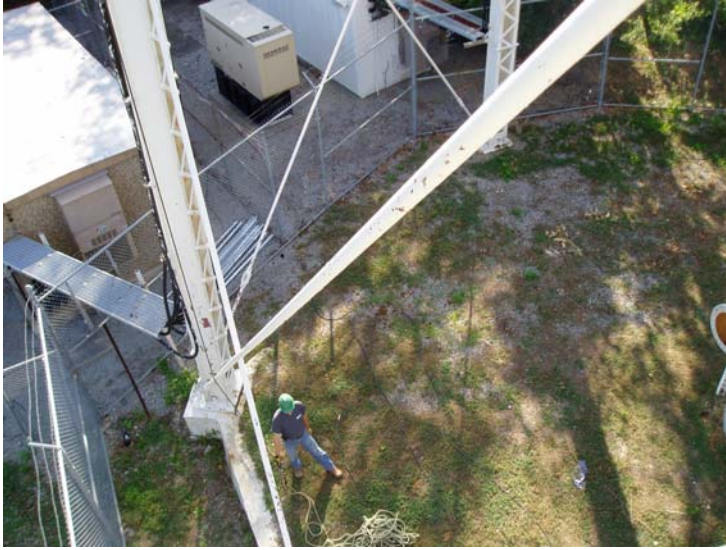
14) Coating breaks to substrate On asway rod.
