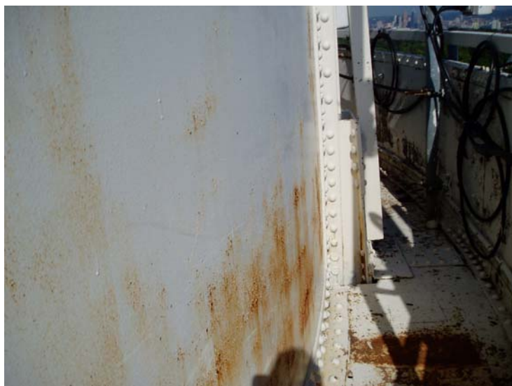
25) Rust bleedthrough and erosion of the sidewall coating.
