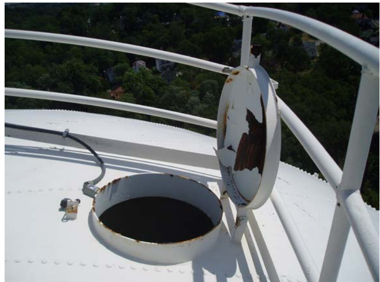
33) Delamination of coating on the ventilation hatch.
