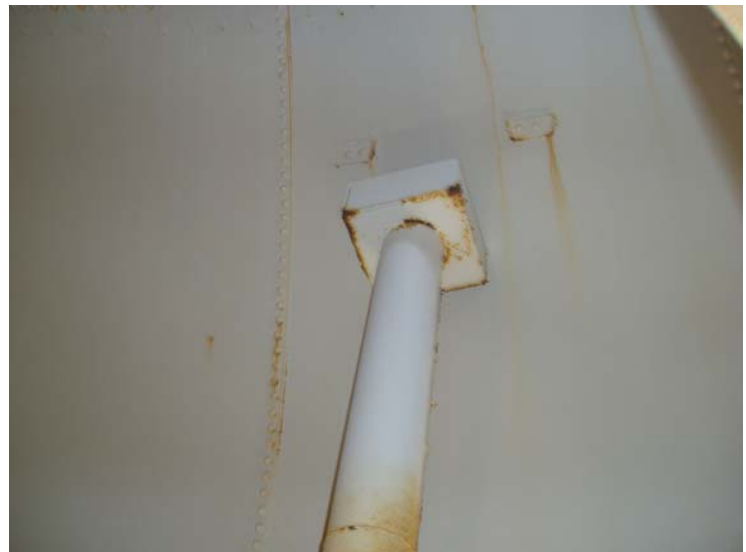
39) Rust bleedthrough on the overflow weir box and riveted seams.
