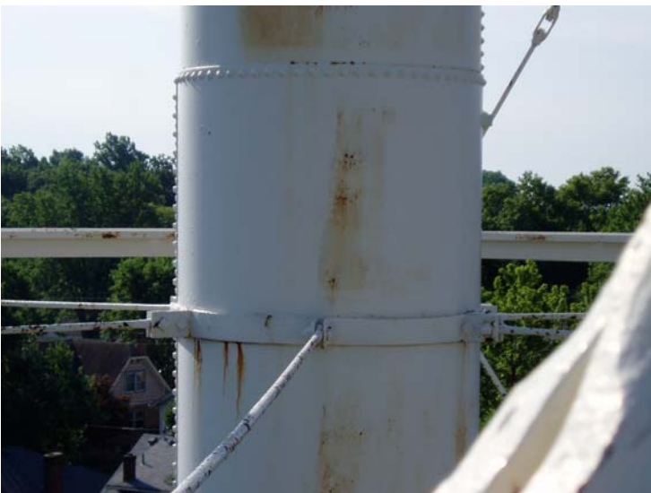
16) Corrosion and rust staining behind a riser tie band, and coating erosion on the riser.
