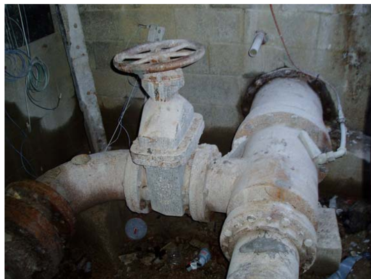
52) The pit piping has no coating remaining.
