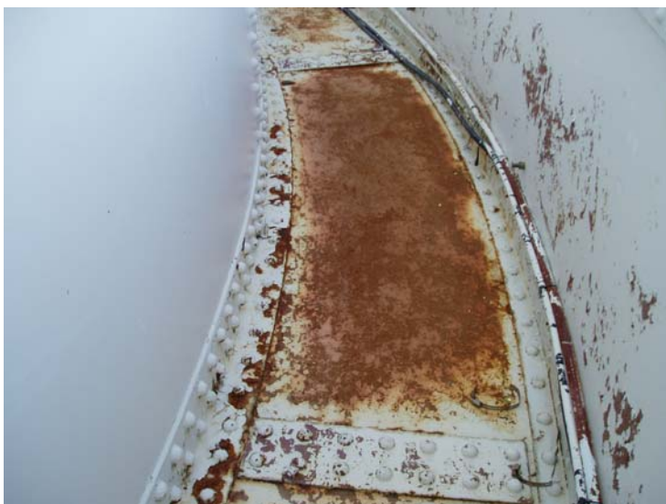
22) Rust bleed through and delaminations on the balcony floor. No drainage holes in this section.
