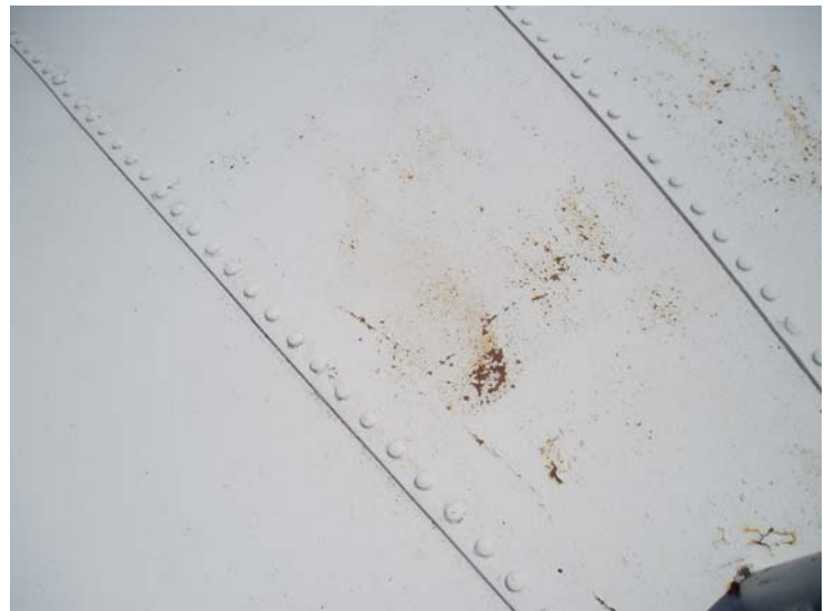
30) Coating erosion on the roof.
