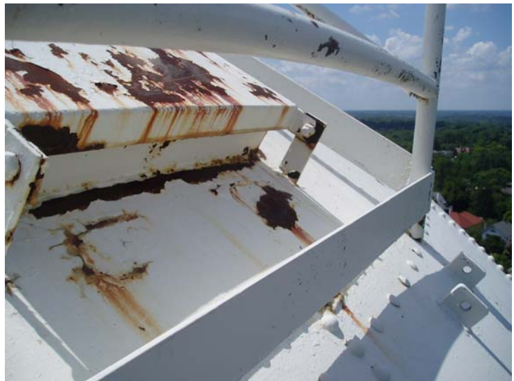
36) Corrosion and rust staining around the hatch to the wet interior.
