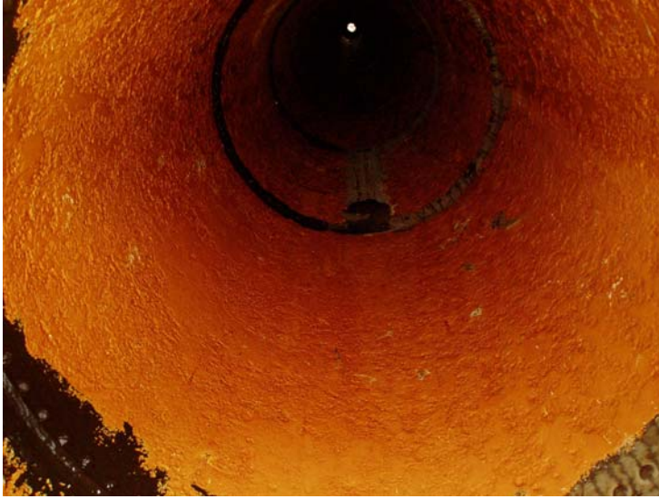
50) A tar like substance has been applied to part of the riser seams—other areas of the seams have exposed substrate.
