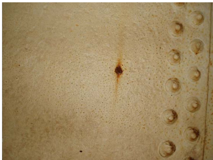
43) Active pitting on the tank sidewall.
