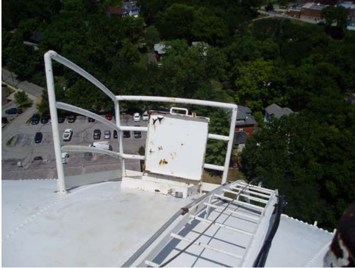
29) Coating breaks to substrate on the wet interior roof hatch.
