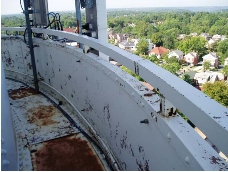
23) Extensive balcony coating deterioration.
