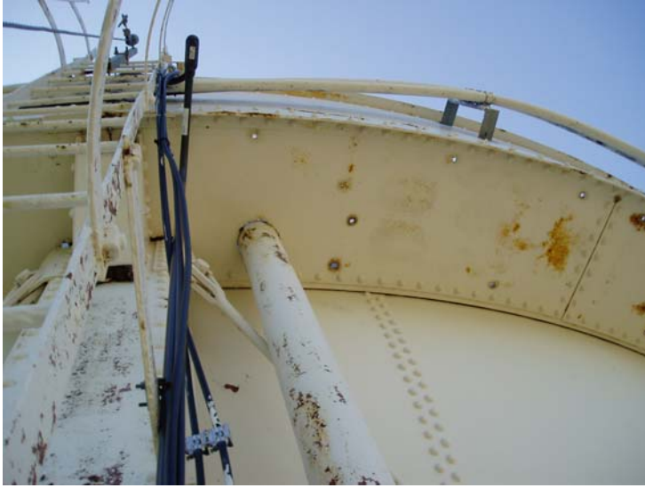
20) Coating erosion on the leg ladder, bowl, overflow pipe, and below the balcony floor.
