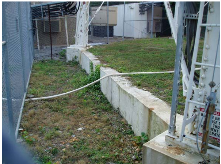
3) Minor foundation deterioration.
