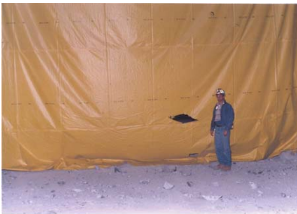
Figure 6. Fly rock damage in brattice cloth.
