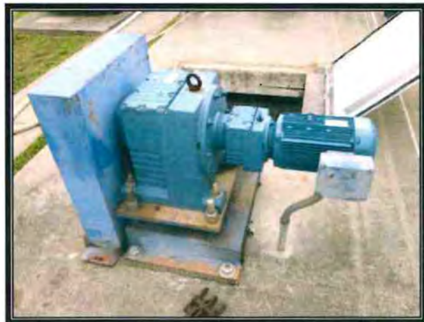
Photo 4 - Basin #1 Flocculator Drive (Typ.)
