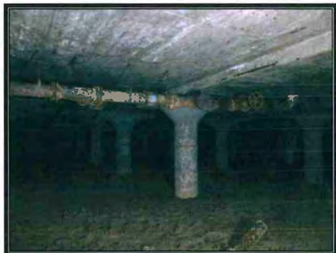
Photo 20 - Basin #2 / #3 Sludge Drain Lines (Typ.)
