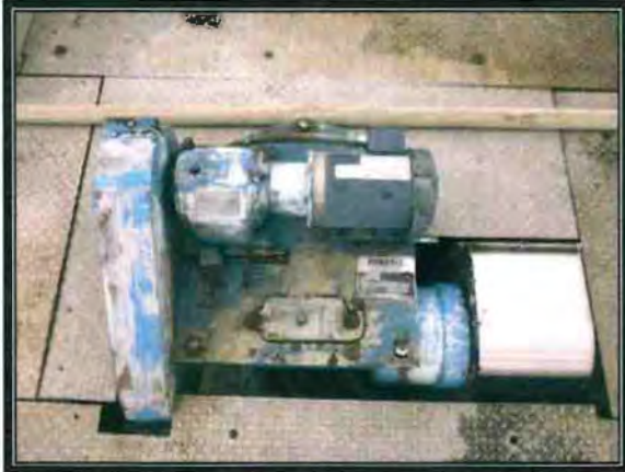
Photo 9 - Basin #1 Clarifier Sludge Rake Drive
