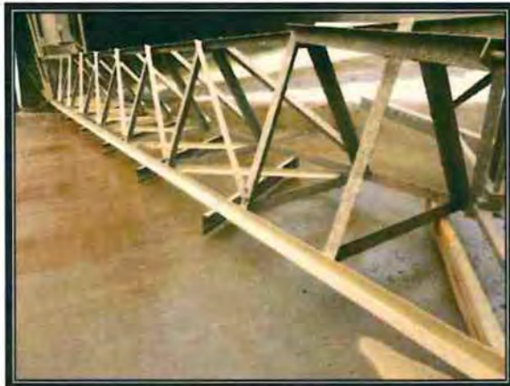
Photo 7 - Basin #1 Clarifier Sludge Rake Arm
