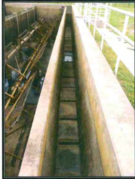
Photo 6 - Basin #1 Influent Flow Channel
