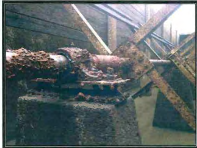
Photo 18 - Basin #2 / #3 Horiz. Flocculator Condition (Typ.)
