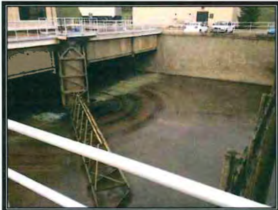
Photo 11 - Basin #2 / #3 Clarifier (Typ.)
