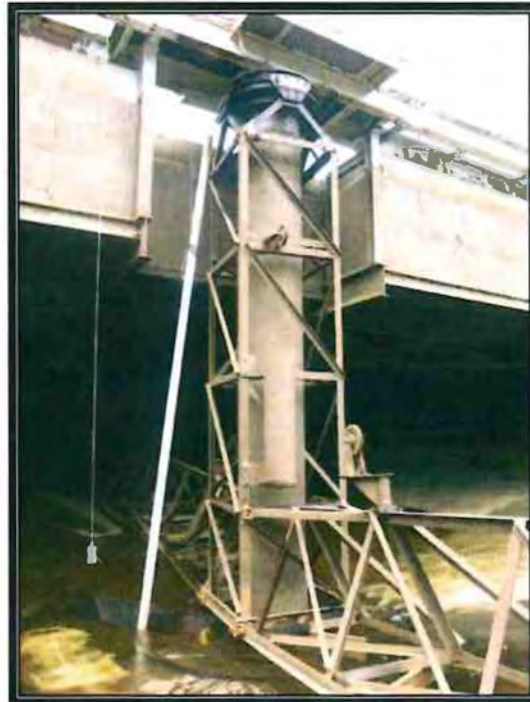
Photo 8 - Basin #1 Clarifier Sludge Rake
