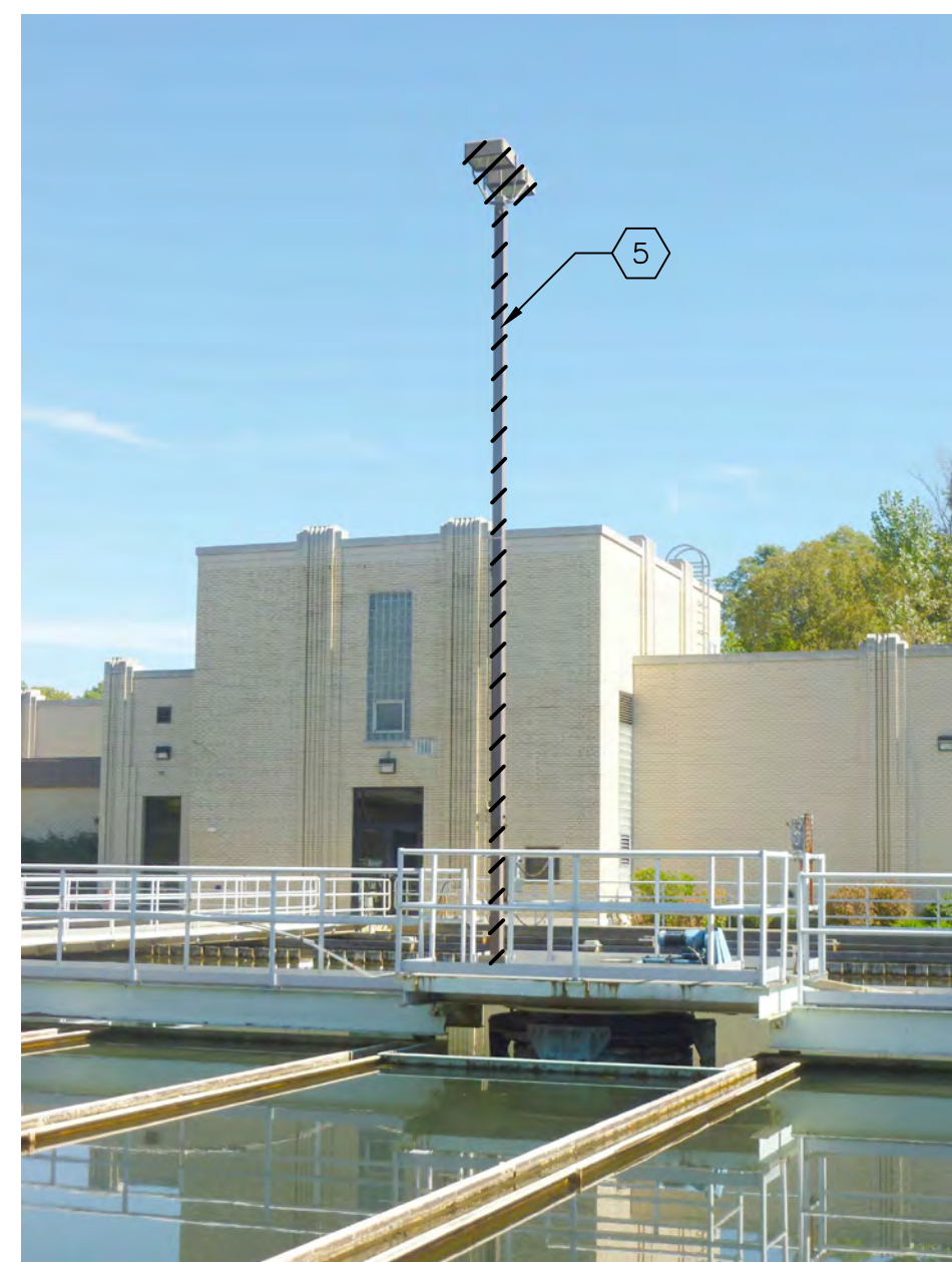
PHOTO 10 BASIN #3 CLARIFIER LIGHT POLE
