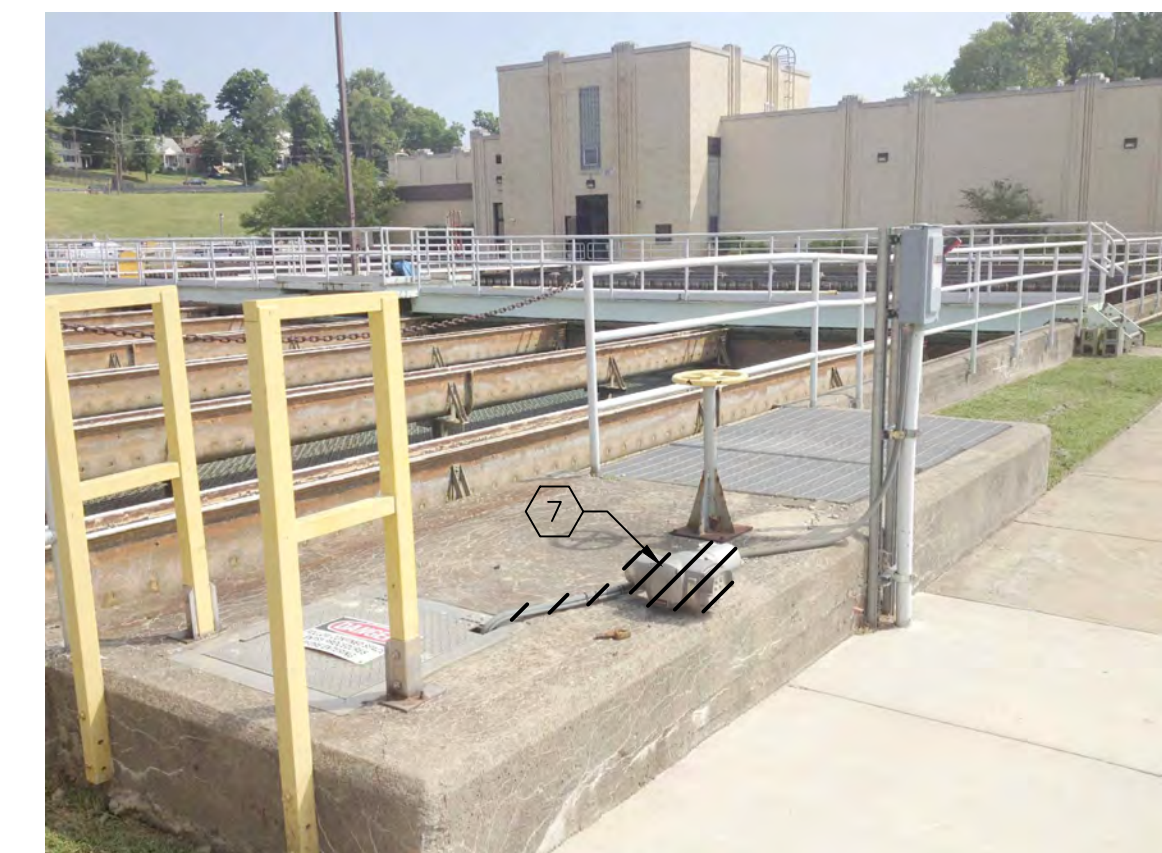
PHOTO 11 - BASIN #2 AND #3 (TYPICAL) 6" SLUDGE PLUG VALVE ACTUATOR CONTROLS
