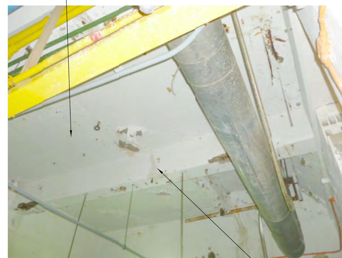
PHOTO #3 - AREA "B" TYPICAL CONCRETE CONDITION N.T.S. - PERFORM BEAM REPAIR METHOD B (2 BEAMS IN AREA "B")
