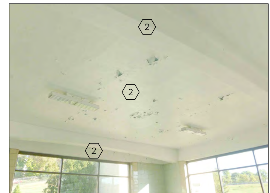
TYPICAL COATING CONDITION PHOTO 2 NTS
