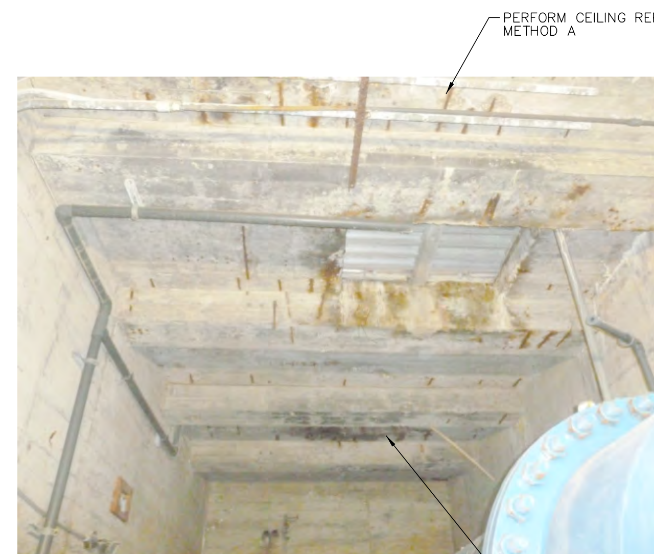
PHOTO #1 - AREA "A" TYPICAL CONCRETE CONDITION N.T.S. - PERFORM BEAM REPAIR METHOD A (TYP. AREA "A")
