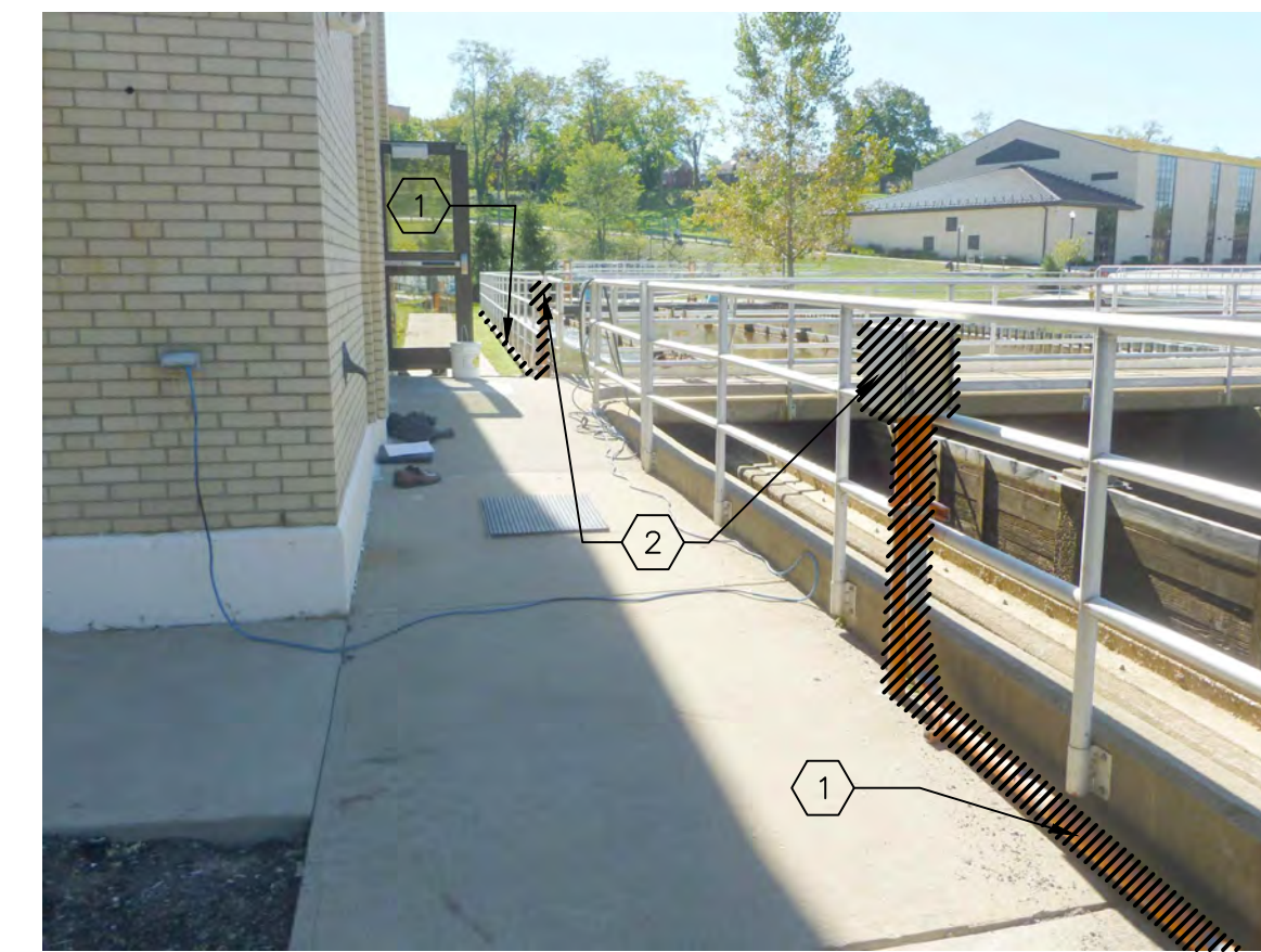
PHOTO 4 BASIN #2 CLAR. & FLOC. ELECTRICAL
