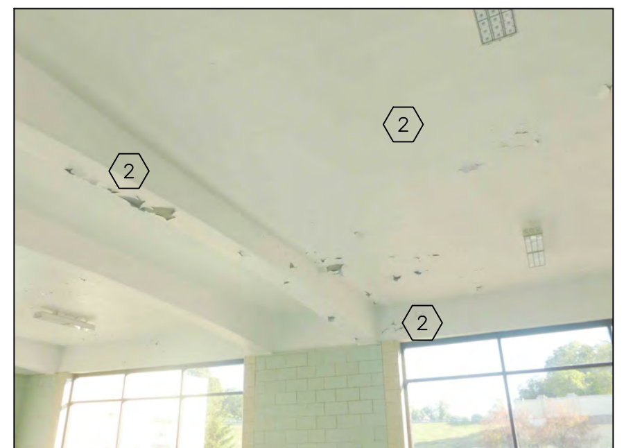
TYPICAL COATING CONDITION PHOTO 1 NTS
