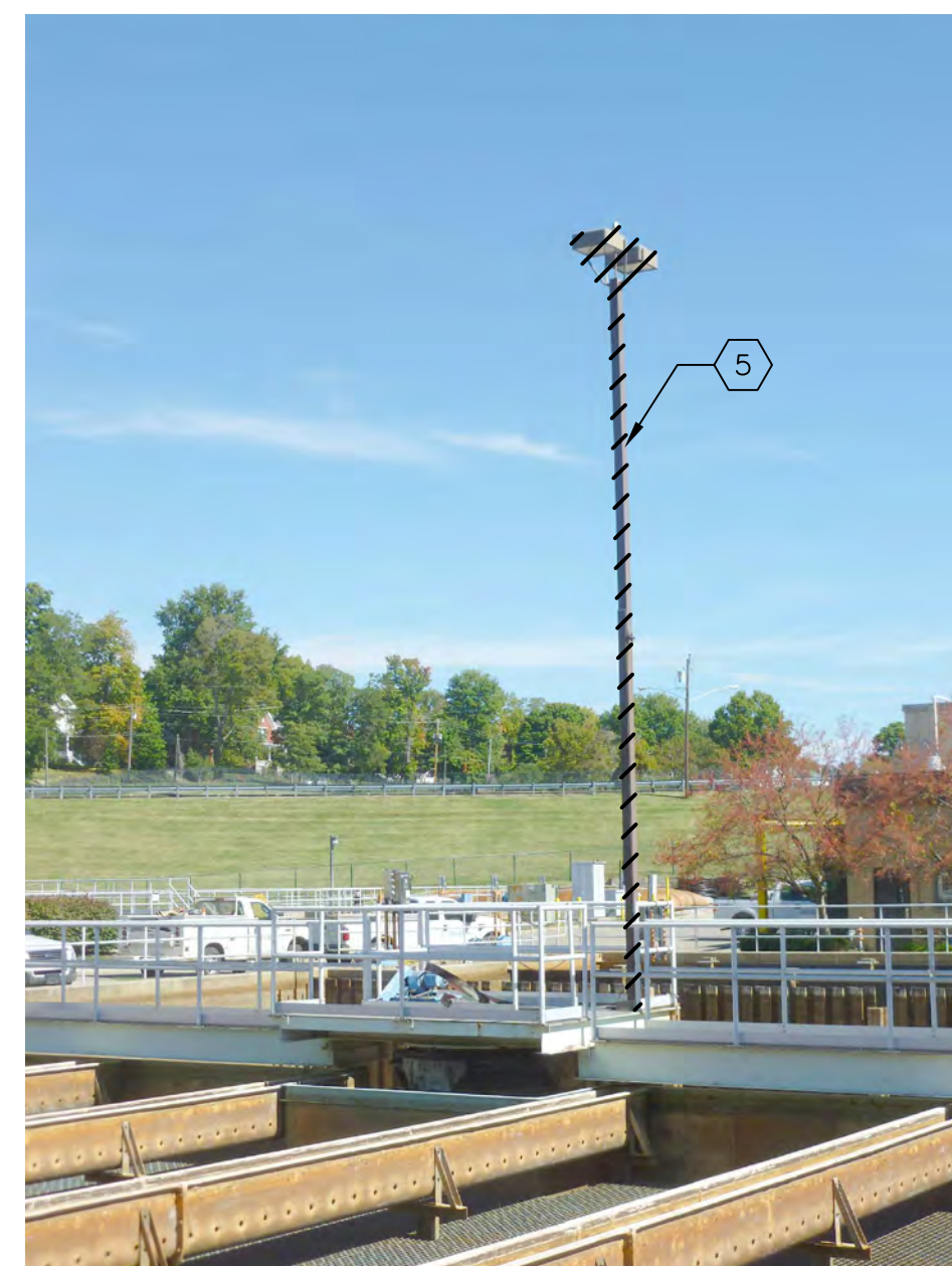
PHOTO 11 BASIN #2 CLARIFIER LIGHT POLE
