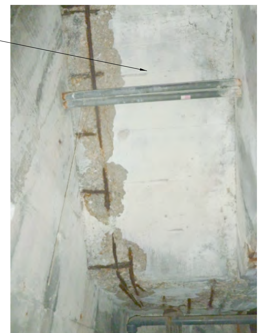
PHOTO #2 - AREA "A" STAIRWAY TYPICAL CONCRETE CONDITION N.T.S. - PERFORM CEILING REPAIR METHOD A
