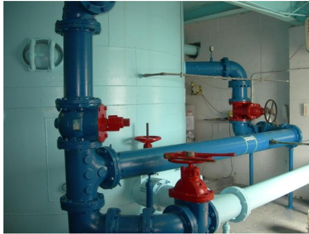
Exhibit II-2 Water Plant One Filter Equipment June 25, 2012
